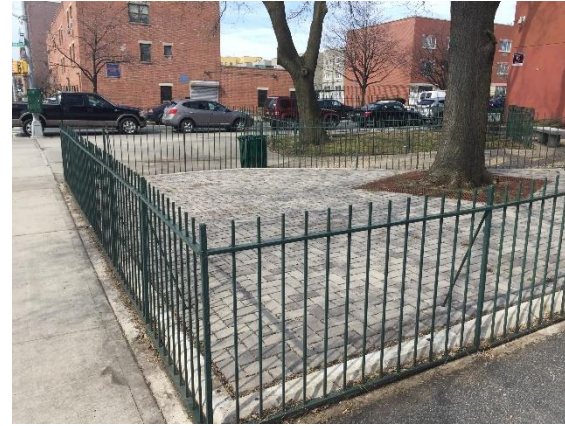
Photo 6: Looking southwest across BCP Site No. C224162; no debris or damages to permeable pavers.
