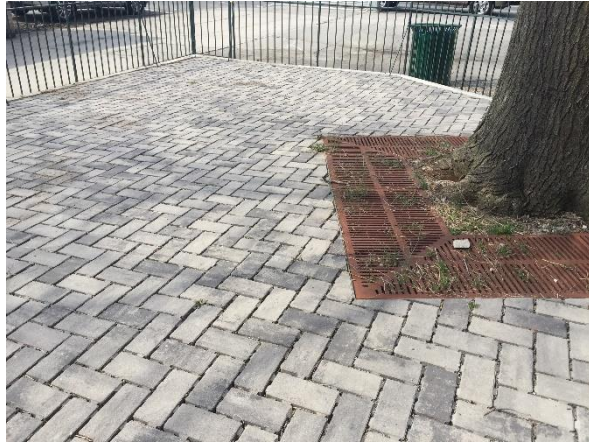
Photo 5: Facing south looking down at grating and permeable pavers; area is clear with no debris present
