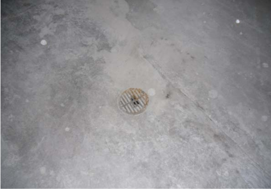
Photo 4 – View of one of the two floor drains inside the building on the subject site
