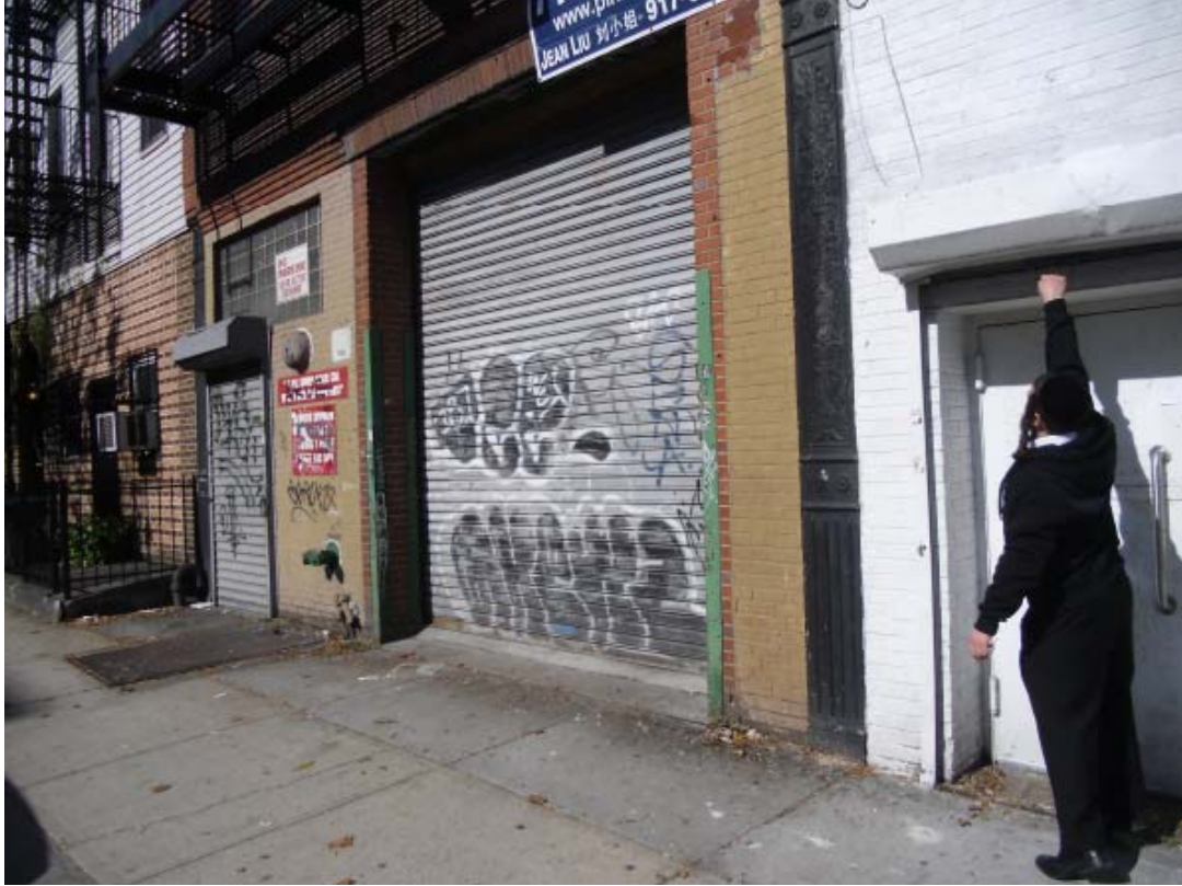
Photo 8 – View of adjacent property (869 Grand Street) with basement, Siamese connection and vents on front of building.
