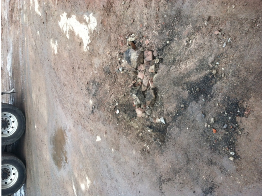
Photo 13: View of FD012 which was destroyed during demolition activities.
