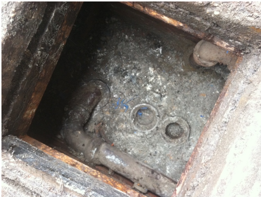
Photo 16: View of FD016 cleaned out. Earthen bottom present.
