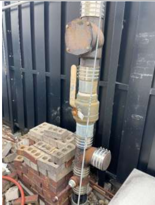
Photo 9: V5 riser in good condition, facing southeast. 05 December 2023.
