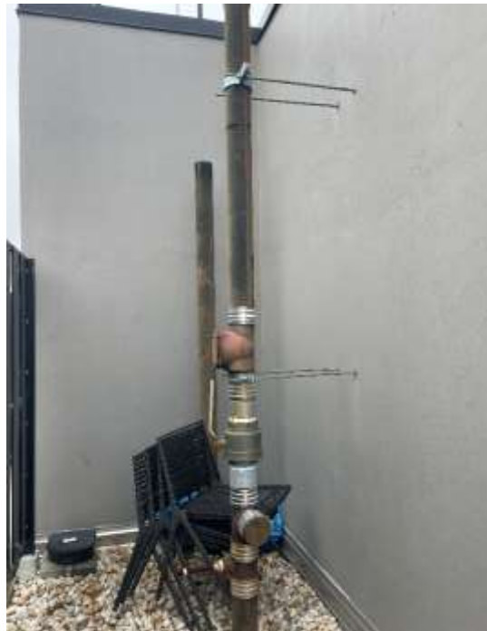
Photo 12: V6 riser and sample port in good condition, facing northwest. 02 March 2023.
