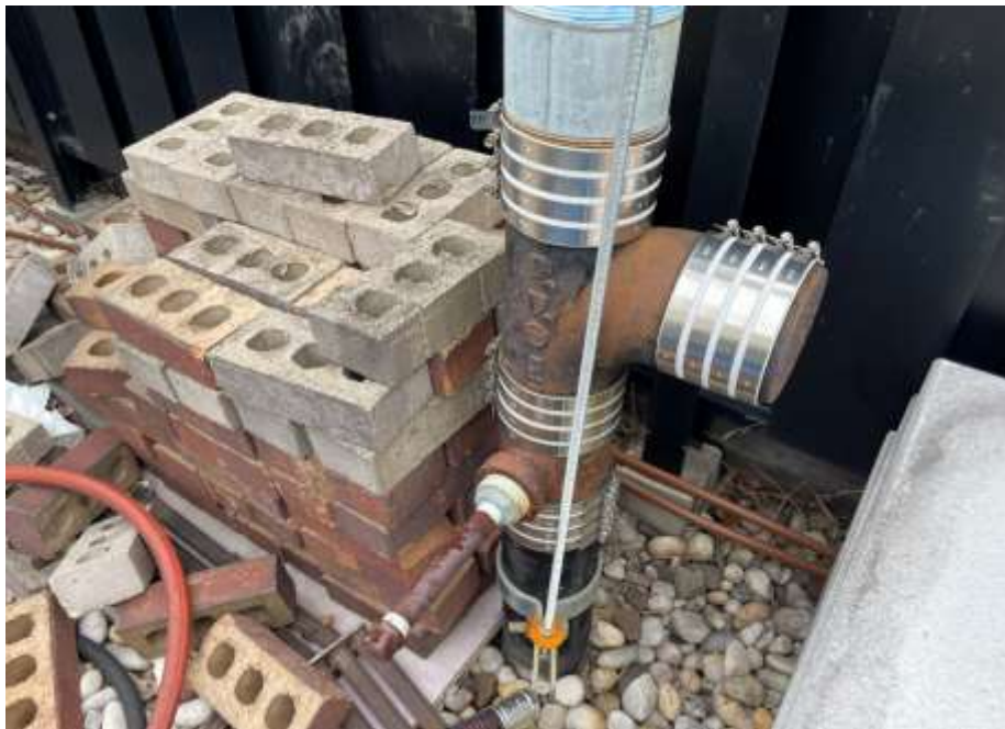
Photo 10: V5 riser and sample port in good condition, facing southeast. 05 December 2023.
