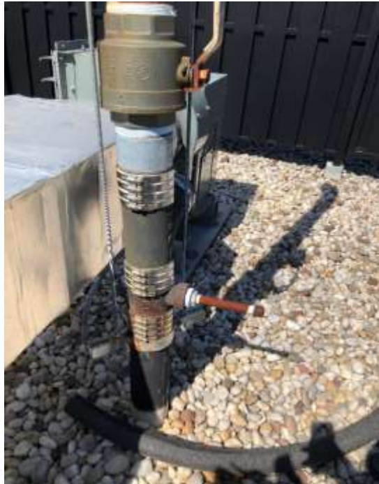
Photo 5: V3 riser and sample port in good condition, facing east. 20 June 2022.
