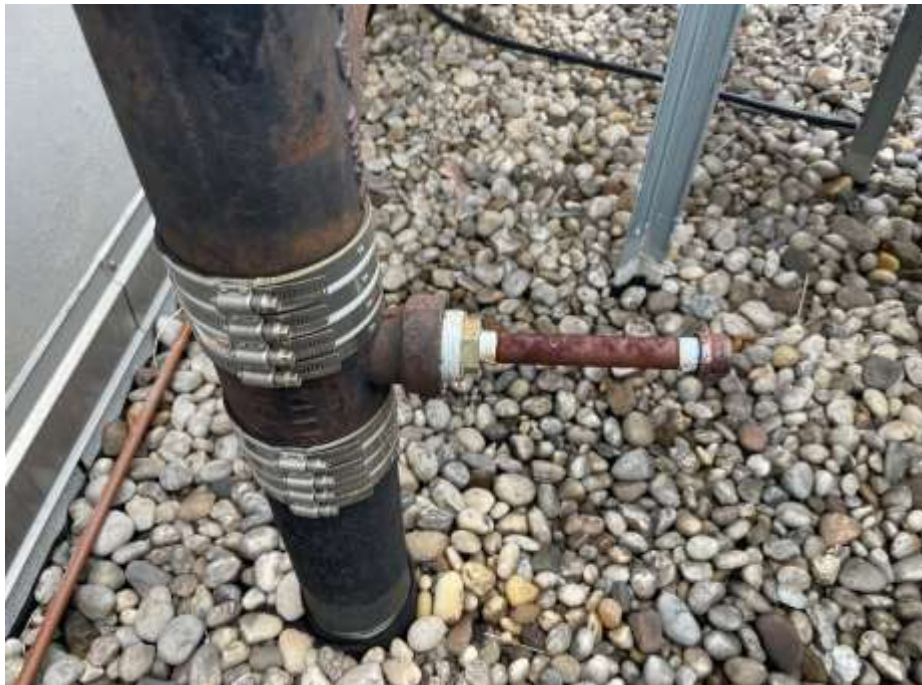
Photo 8: V4 riser and sample port in good condition, facing east. 02 March 2023.
