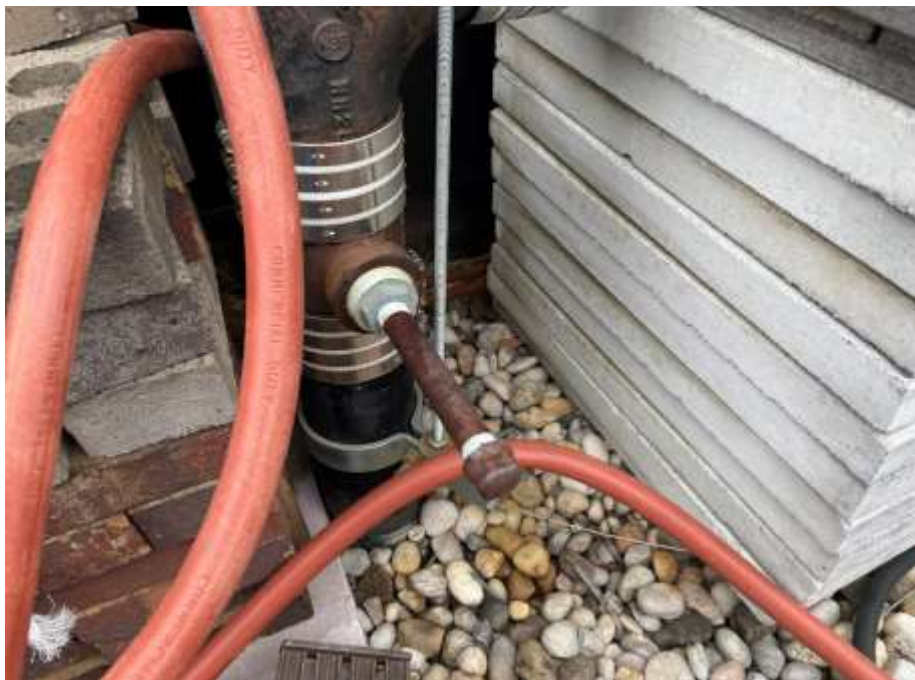
Photo 10: V5 riser and sample port in good condition, facing southeast. 02 March 2023.
