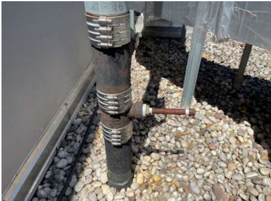
Photo 8: V4 riser and sample port in good condition, facing east. 20 June 2022.
