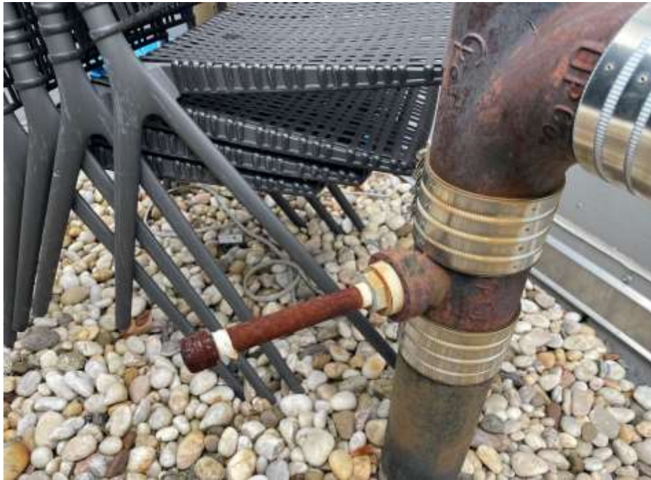
Photo 13: V6 riser and sample port in good condition, facing northwest. 8 April 2021.
