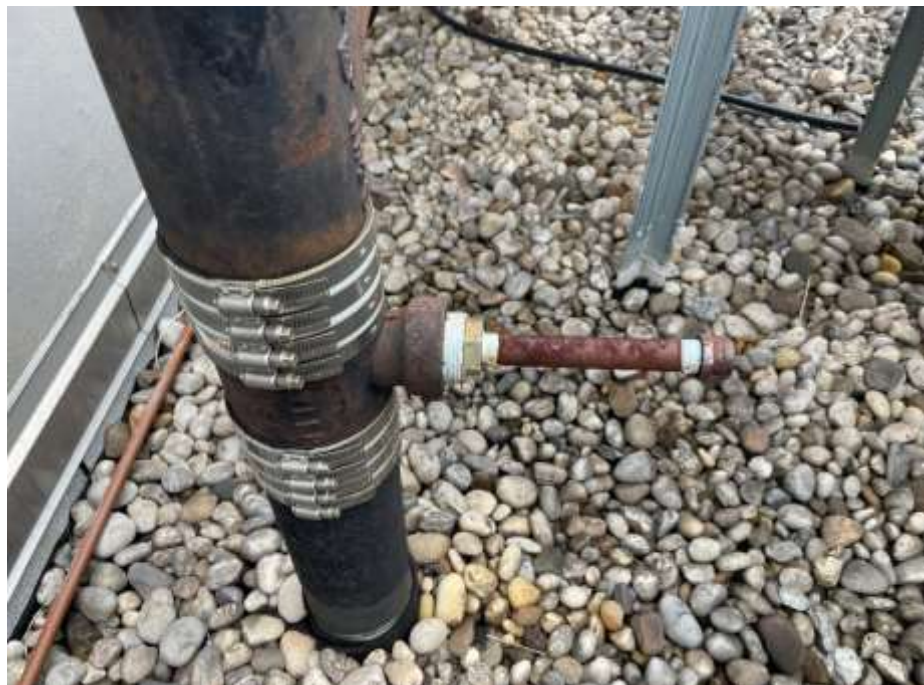
Photo 8: V4 riser and sample port in good condition, facing east. 05 December 2023.
