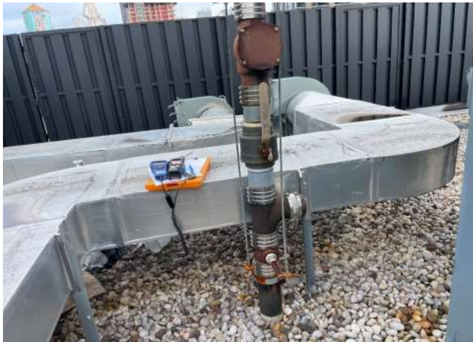
Photo 5: V3 riser and sample port in good condition, facing east. 05 December 2023.
