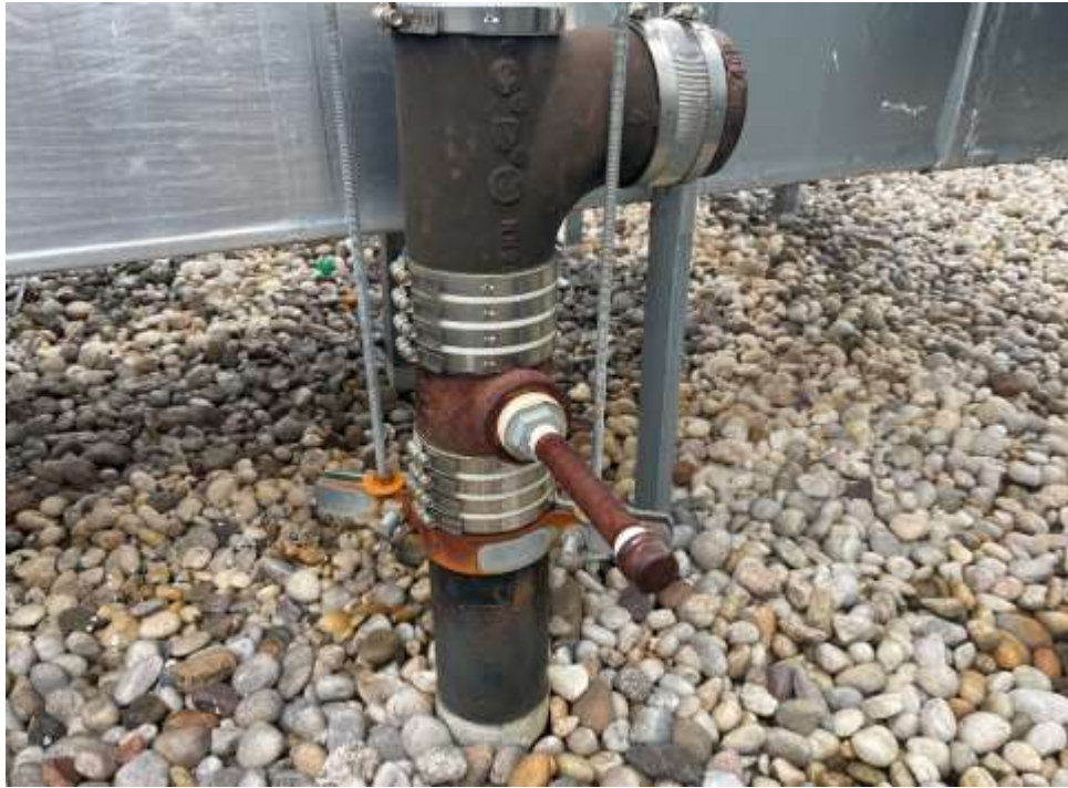
Photo 5: V3 riser and sample port in good condition, facing east. 02 March 2023.
