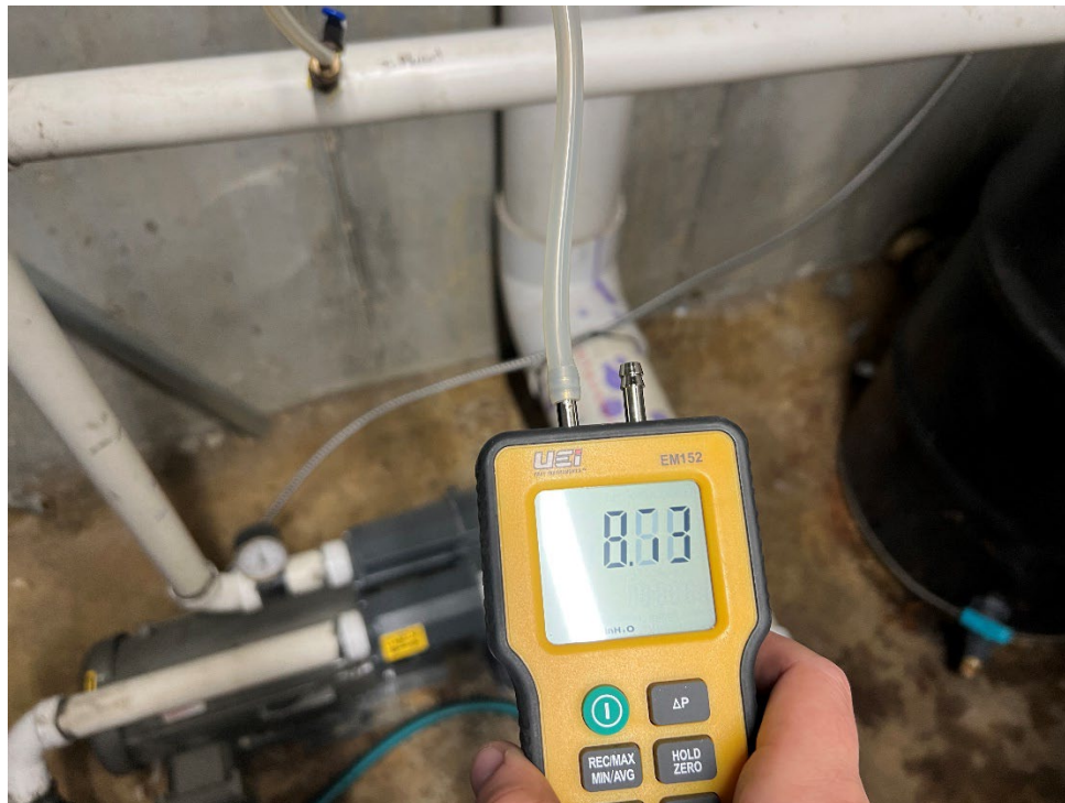
Photograph No. 2: Negative Pressure was confirmed within the influent piping leading to the blower.
