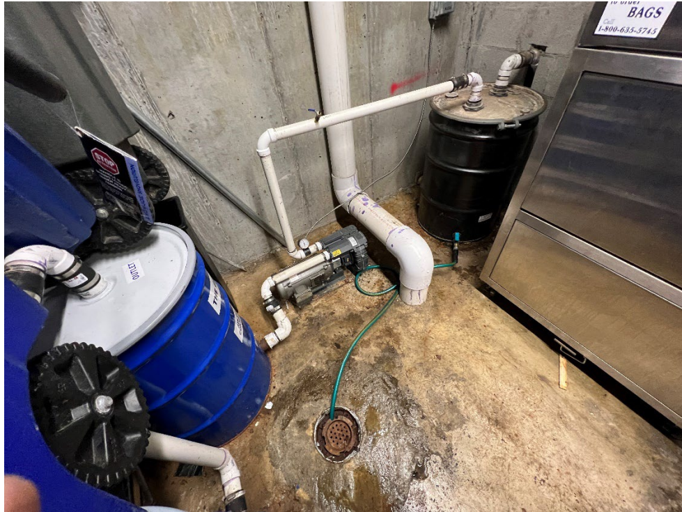
Photograph No. 1: View of the new knockout drum, Blower, and Carbon Drums associated with the SVE system on site.
