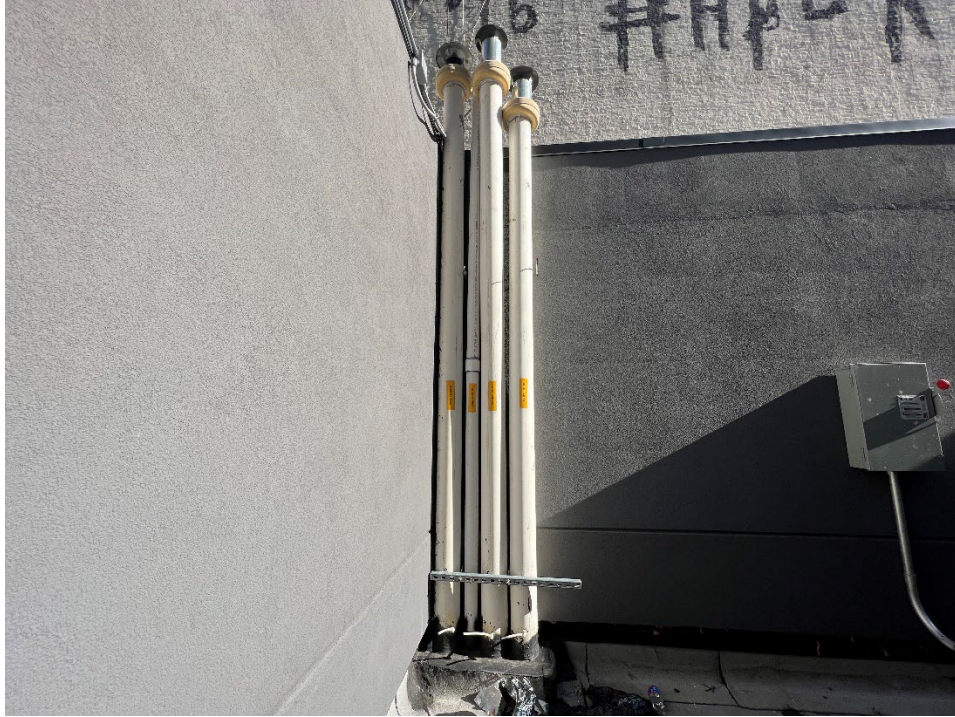
Photograph No. 5: View of the SSDS Discharge Piping with proper signage and no deficiencies,
