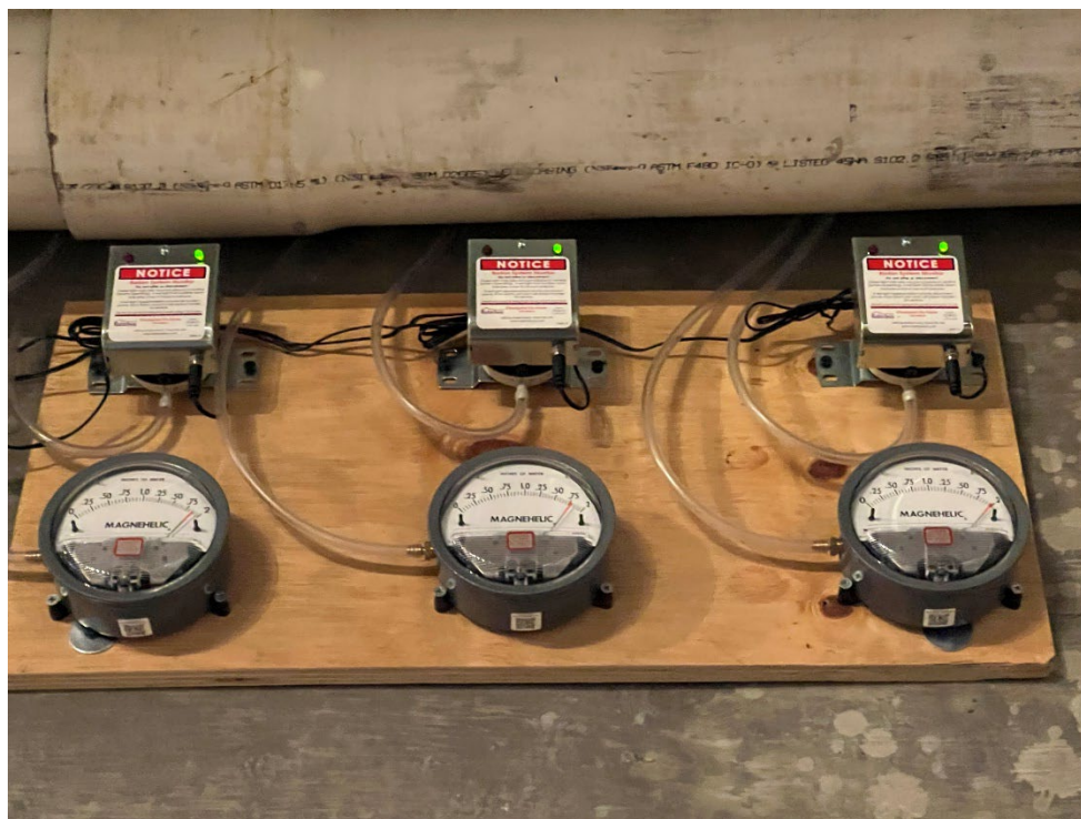
Photograph No. 4: Negative Pressure was confirmed in each leg of the active SSDS on Site. No Alarms were active during the annual inspection.
