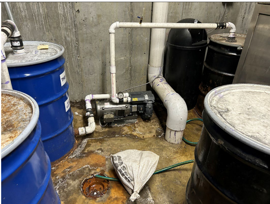
Photo 3 – Overview of the SVE system with knock-out drum, blower, and double granulated activated carbon filtration.
