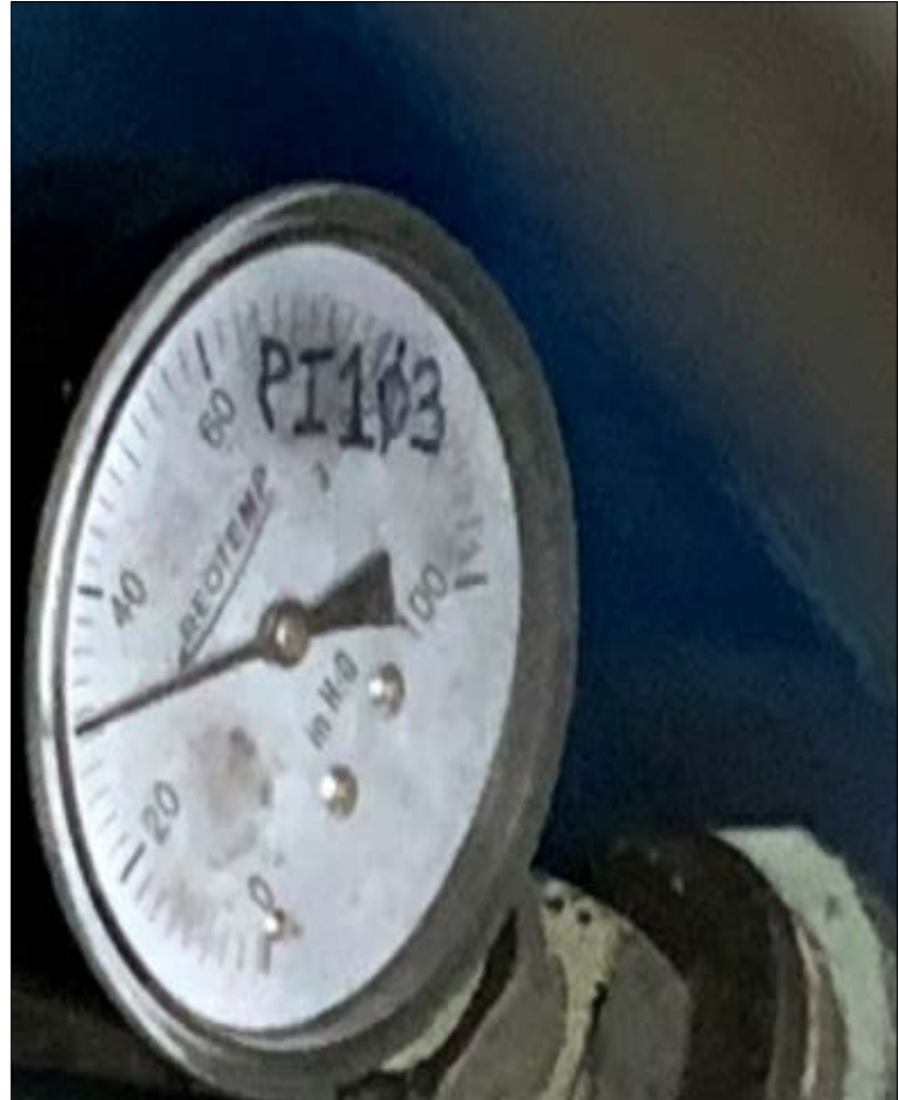
SSDS Pressure Gauge PI103 (After Lead and Before Lag Carbon Treatment Drum) Pressure = 31 inches of H 2 O
