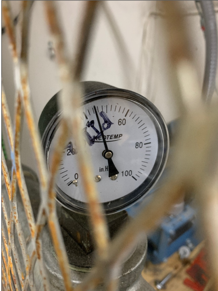
SSDS Pressure Gauge PI102 (Before Lead Carbon Treatment Drum) Pressure = 45 inches of H 2 O
