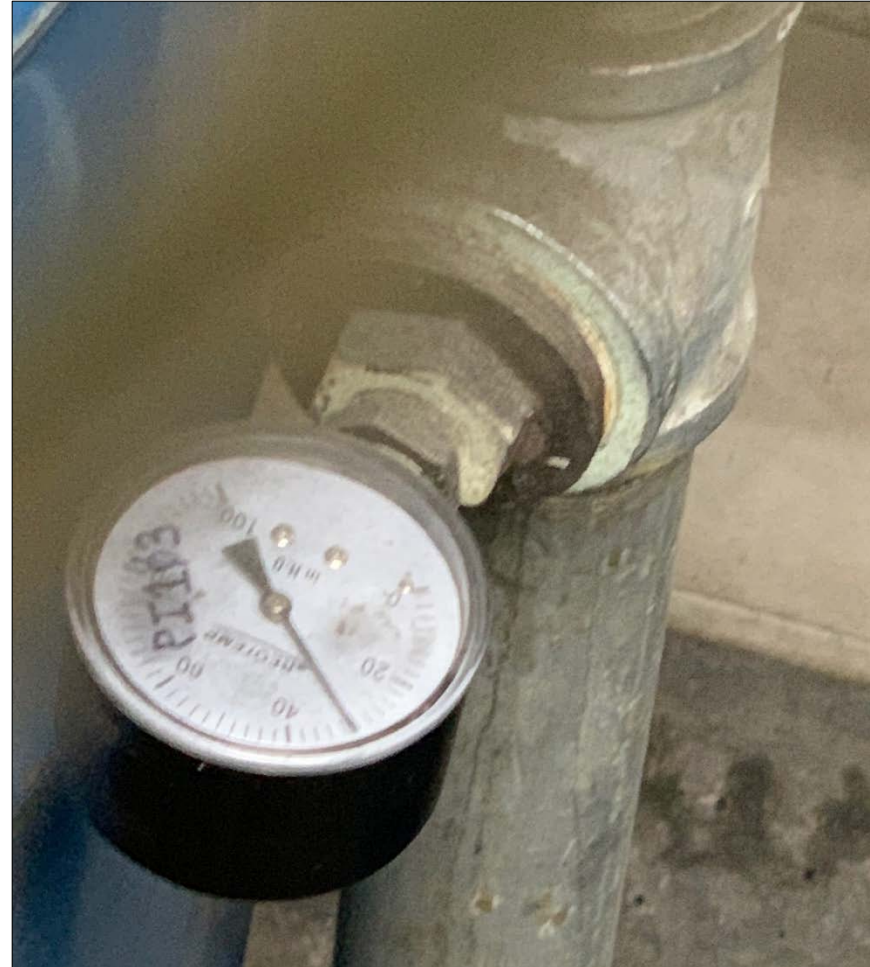
SSDS Pressure Gauge PI103 (After Lead and Before Lag Carbon Treatment Drum) Pressure = 31 inches of H 2 O
