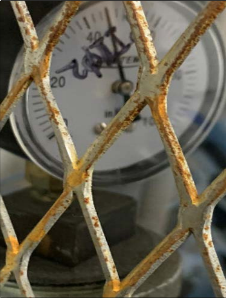
SSDS Pressure Gauge PI102 (Before Lead Carbon Treatment Drum) Pressure = 46 inches of H 2 O
