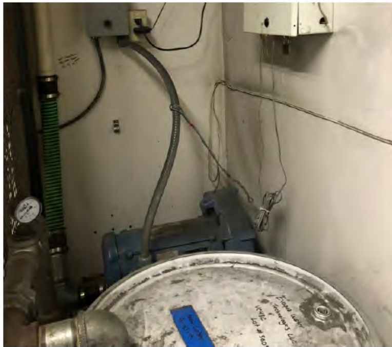
Photograph 2. SSDS Rotron blower and lead carbon drum.
