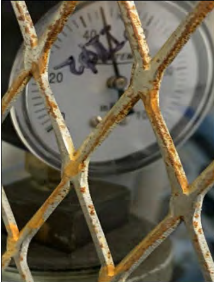
SSDS Pressure Gauge PI102 (Before Lead Carbon Treatment Drum) Pressure = 46 inches of H 2 O
