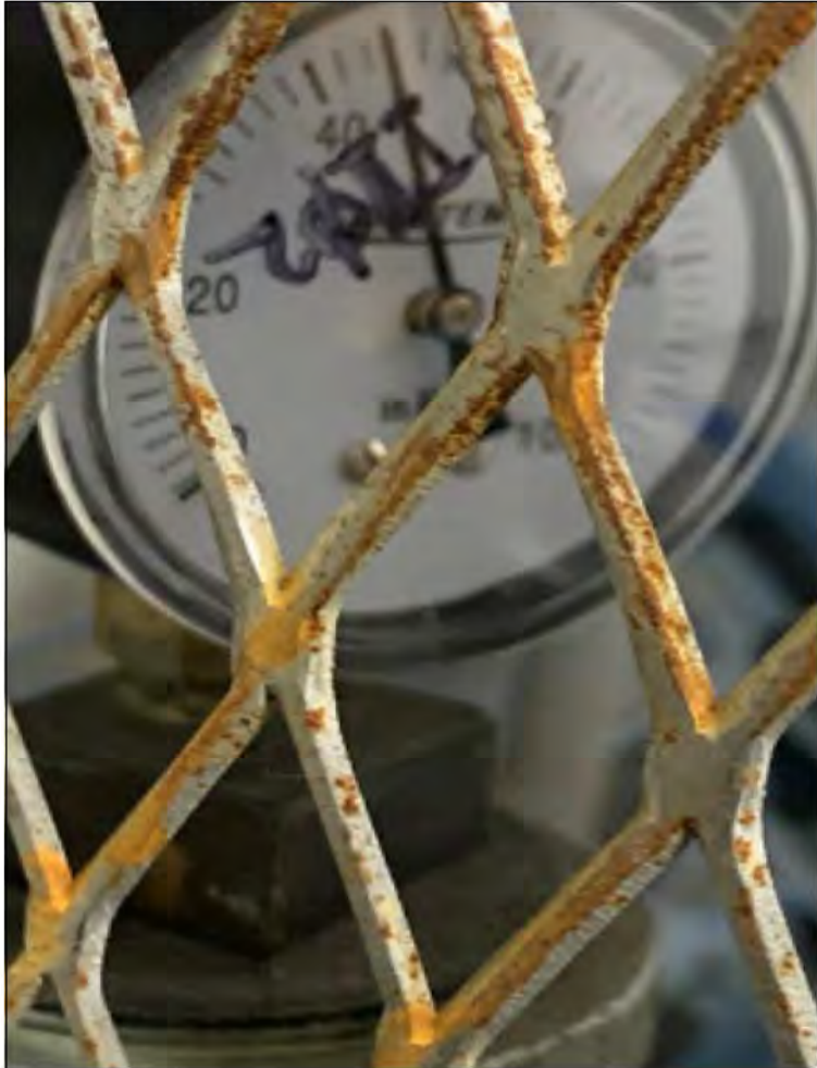
SSDS Pressure Gauge PI102 (Before Lead Carbon Treatment Drum) Pressure = 46 inches of H 2 O
