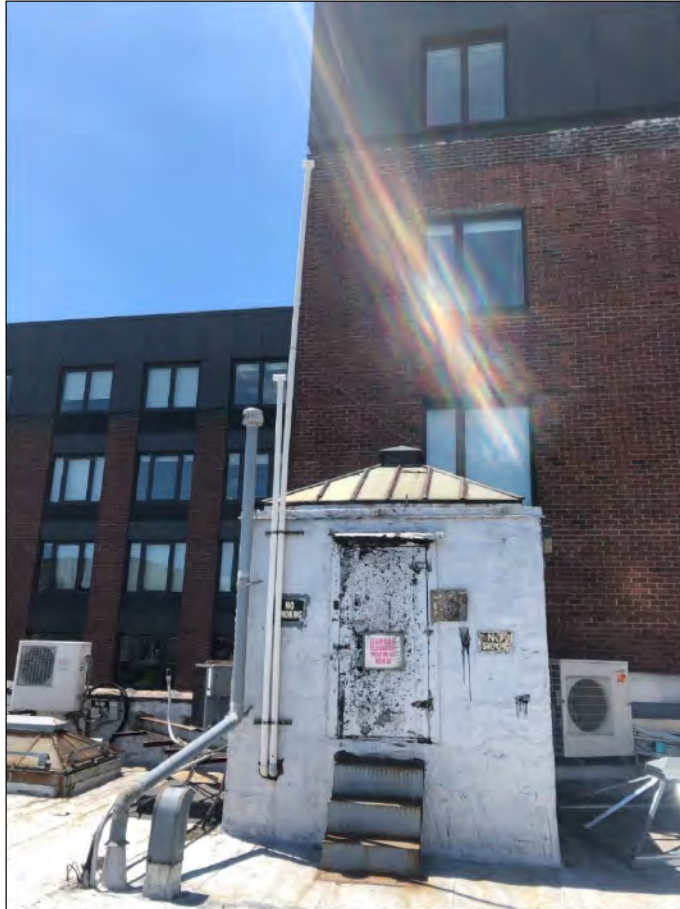
Photograph 7. View of SSDS exhaust riser on the roof.
