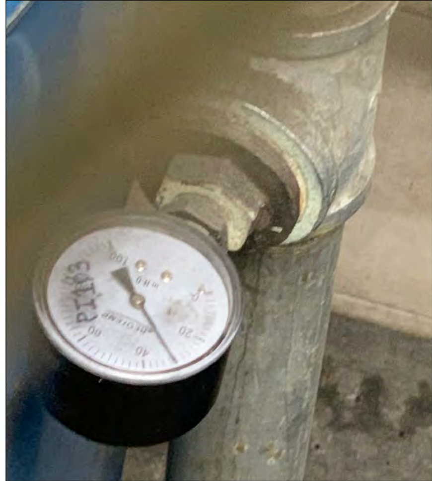
SSDS Pressure Gauge PI103 (After Lead and Before Lag Carbon Treatment Drum) Pressure = 31 inches of H 2 O
