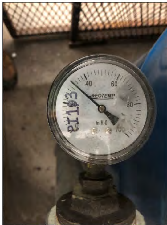
Photograph 4. SSDS pressure gauge PI103 reading 32 iwc.
