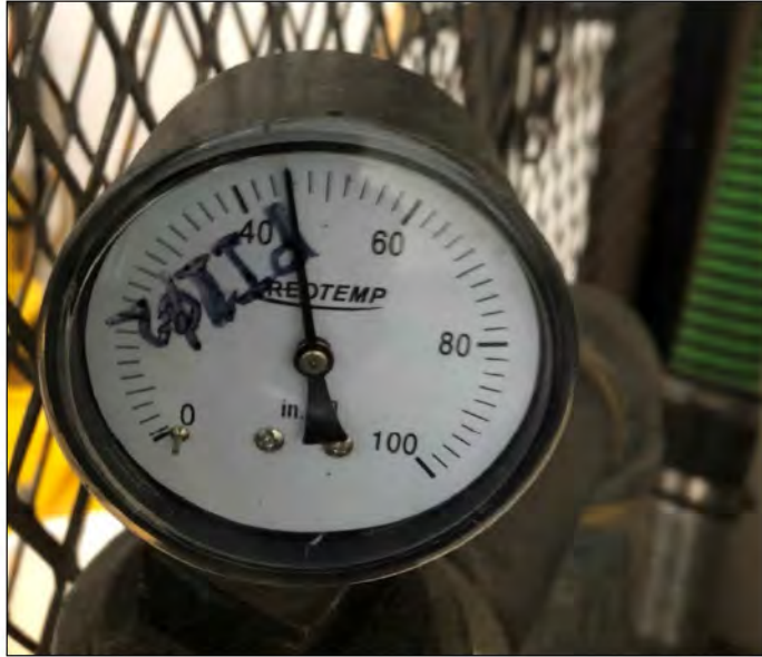
Photograph 3. SSDS pressure gauge PI102 reading 46 iwc.
