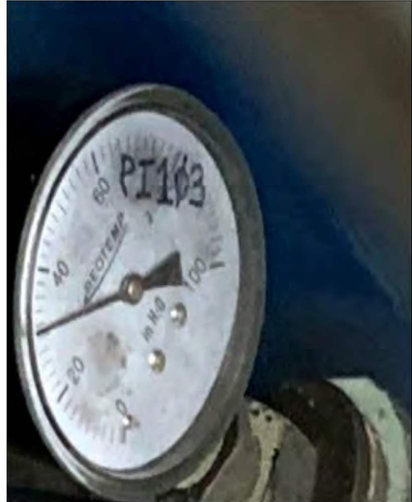
SSDS Pressure Gauge PI103 (After Lead and Before Lag Carbon Treatment Drum) Pressure = 31 inches of H 2 O
