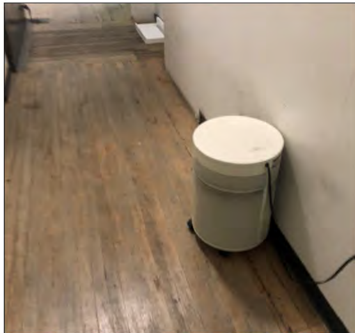
Photograph 8. Air filtration unit in the first-floor rear hallway by the elevator.
