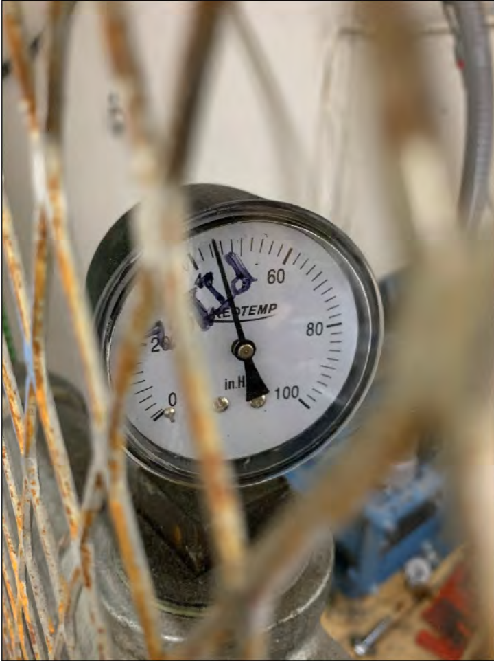
SSDS Pressure Gauge PI102 (Before Lead Carbon Treatment Drum) Pressure = 45 inches of H 2 O
