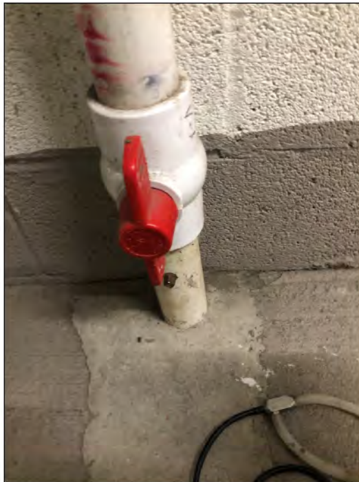
Photograph 6. Vapor well V-1 valve position.
