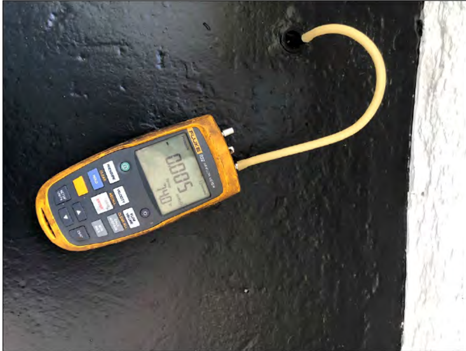
Photograph 5. Fluke 922 Air Flow Meter used for vacuum reading, recording -0.005 iwc at vapor monitoring point PV-11RR.
