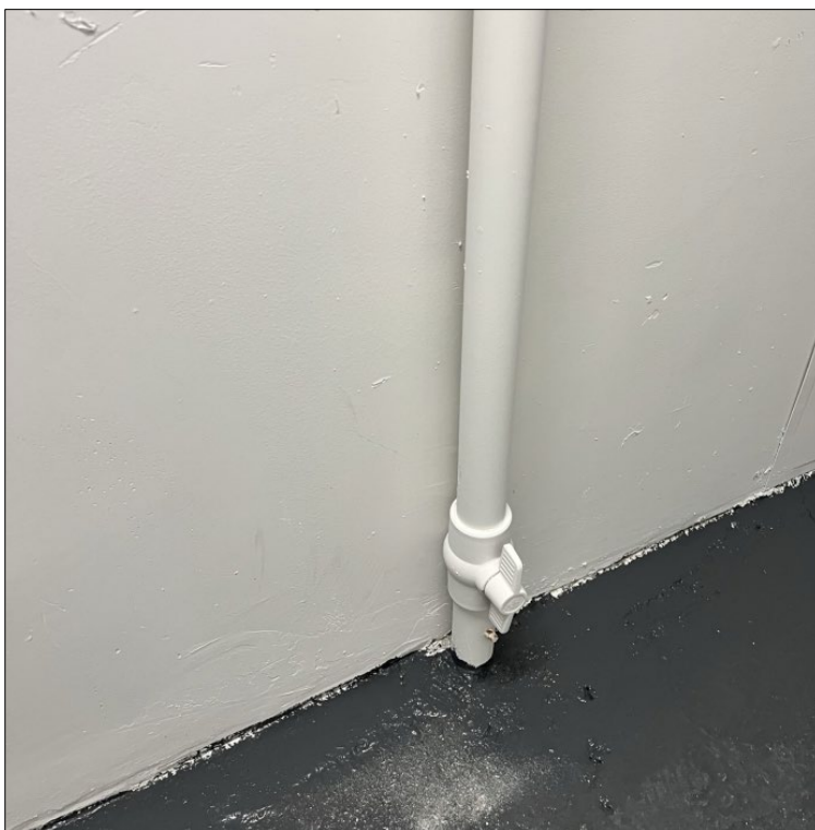
Photograph 6. Vapor well V-4 valve position. December 8, 2022.
