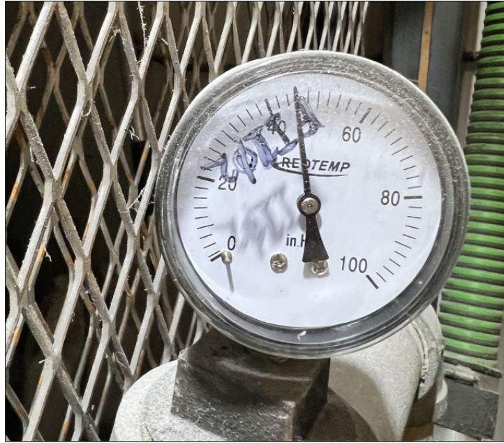
Photograph 3. SSDS pressure gauge PI102 reading 46 iwc. December 8, 2022.
