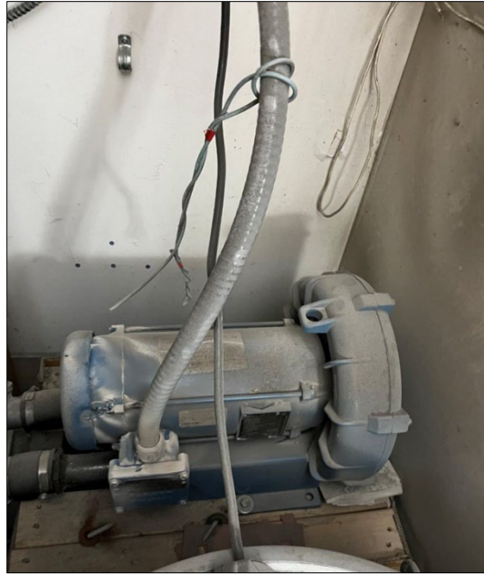
Photograph 10. SSDS Rotron blower. December 27, 2023.
