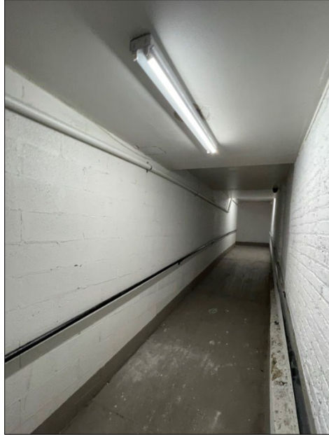
Photograph 14. SSDS piping in rear hallway. December 27, 2023.
