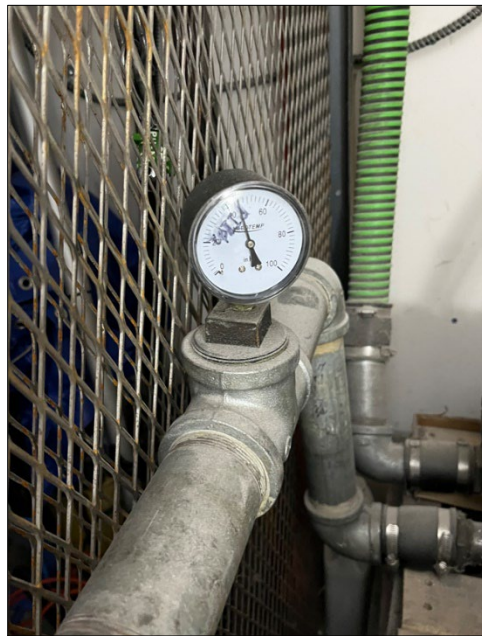
Photograph 11. SSDS pressure gauge PI102 reading 43 iwc. December 27, 2023.
