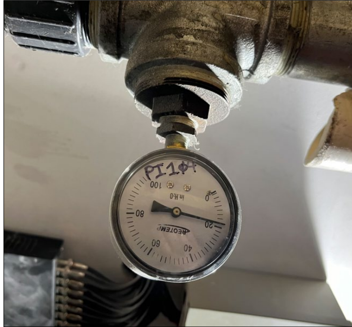
Photograph 12. SSDS pressure gauge PI104 reading 19 iwc. December 27, 2023.
