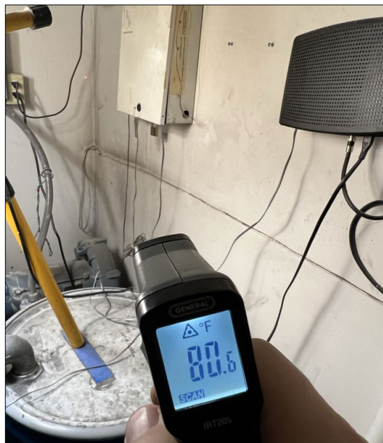
Photograph 2. SSDS Rotron blower, lead carbon drum, and ambient temperature at the time of inspection. December 8, 2022.
