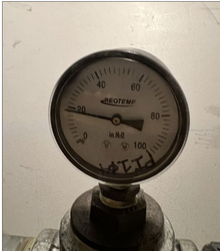
Photograph 4. SSDS pressure gauge PI104 reading 19 iwc. December 8, 2022.
