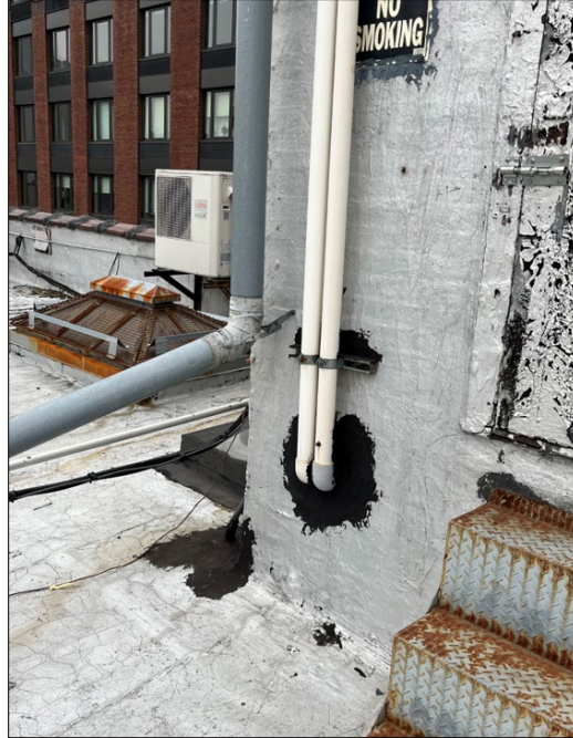
Photograph 16. SSDS exhaust piping on roof. December 27, 2023.
