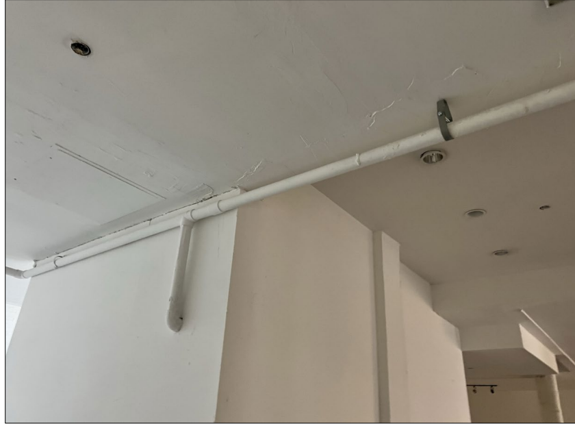
Photograph 7. View of SSDS piping condition. December 8, 2022.
