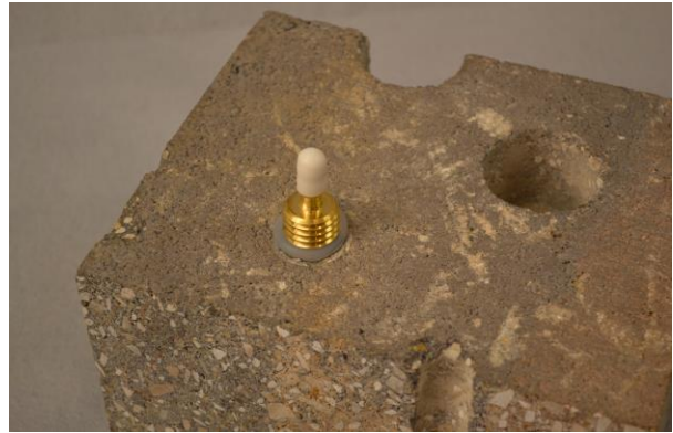
Figure 3. Installed VAPOR PIN® sampling device
