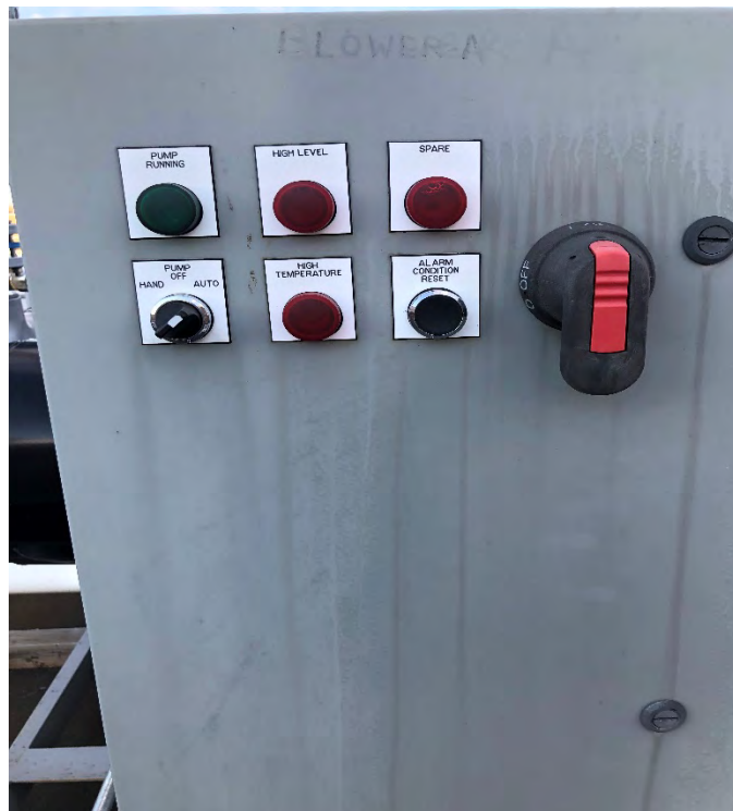
Photo 10: View of Blower A control panel during operation; “pump running” bulb appears to be burnt out
