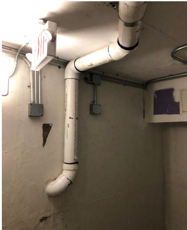
Photo 16: Photo showing monitoring point SVMP-B6 located in the northernmost basement below the residential side of the Site.
