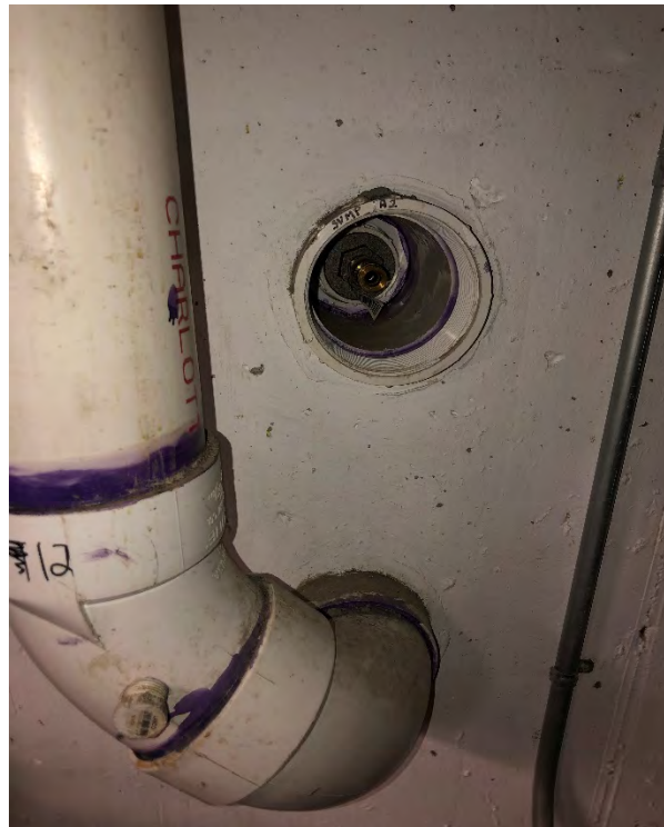
Photo 14: Photo showing monitoring point SVMP-A2 and suction point MG-A12, located in the boiler room.
