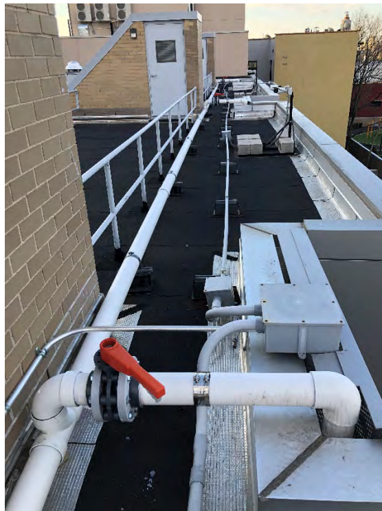
Photo 8: looking south, a photo of Blower A SSDS piping run along the roof on the residential (west) side of the building.
