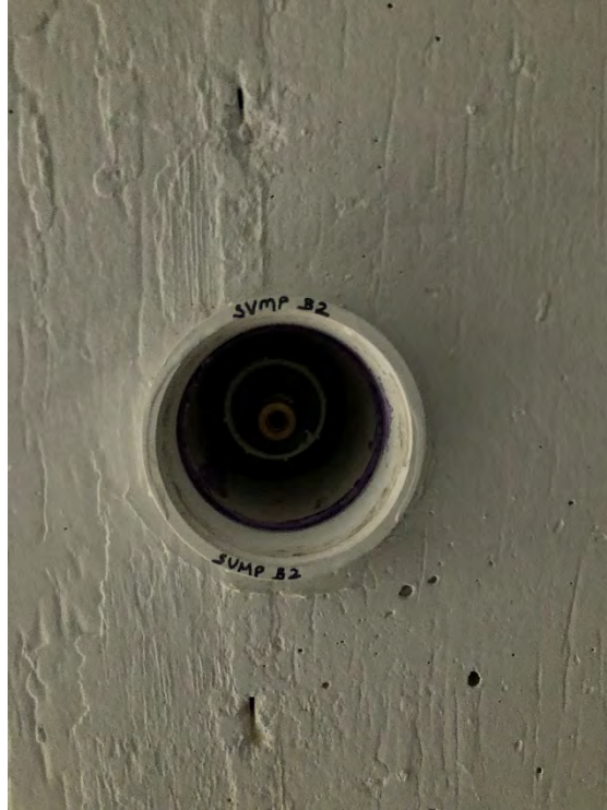
Photo 15: Photo showing monitoring point SVMP-B2 located in the north basement below the commercial space prior to testing.
