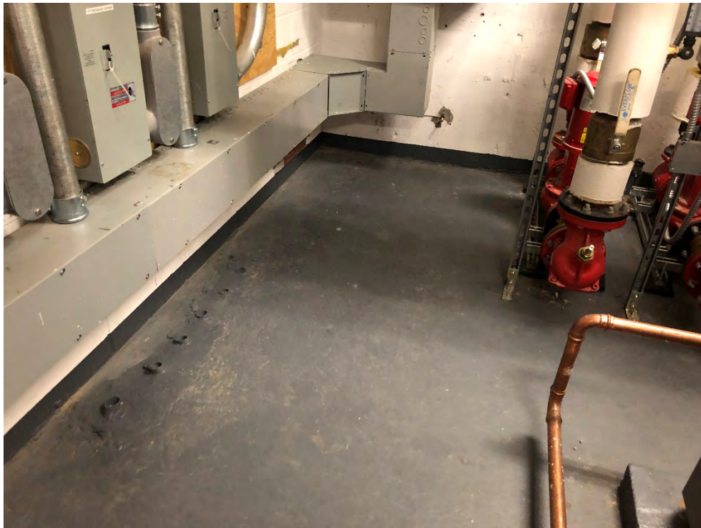
Photo 2: Photo of the concrete slab in the Site's boiler room (west and south wall).
