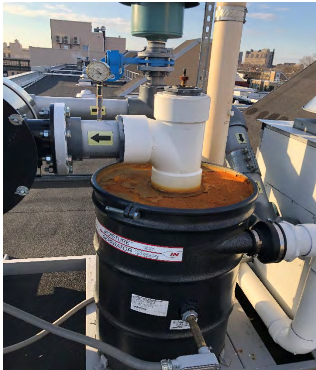
Photo 12: View of Blower B knockout tank and vacuum gauge.
