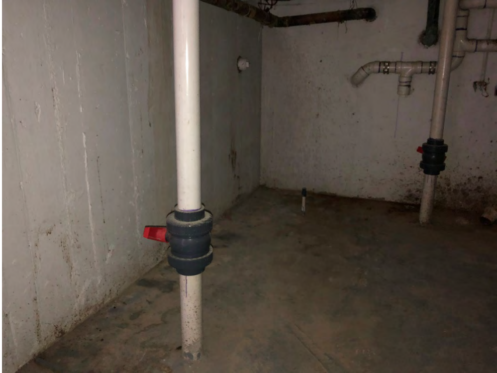
Photo 7: Southwest corner of the north basement; SVE wells, SSDS piping, an injection point, and SVMP-B5 are in view.
