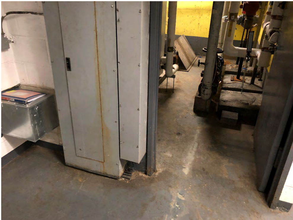
Photo 4: Photo during site cover system inspection in the water main room, located next to the boiler room.
