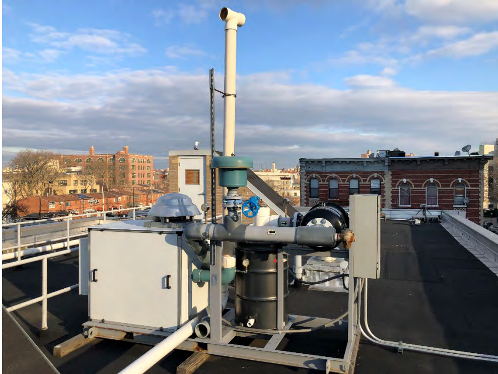
Photo 11: View of Blower B, looking north.
