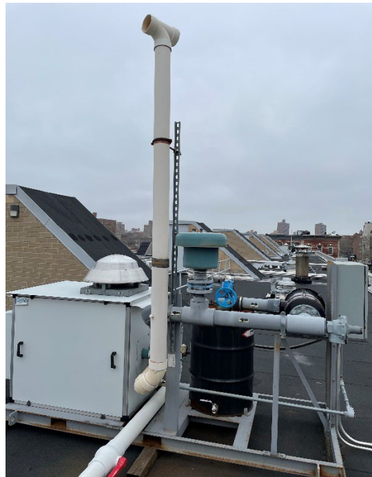
Photo 2: Looking north, a photo of Blower A SSDS enclosure, knock out tank, and exhaust, and influent piping is shown.
