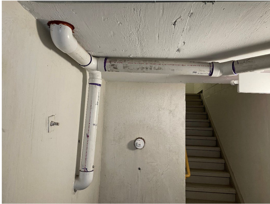
Photo 17: Photo showing piping layout and SVMP-B4 and adjacent suction point MG-B3.
