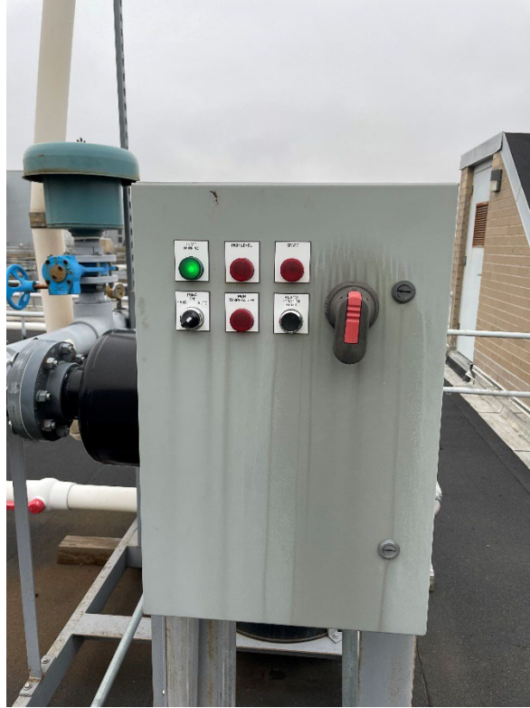
Photo 1: View of Blower A panel with functioning “pump running” bulb shown as functional.
