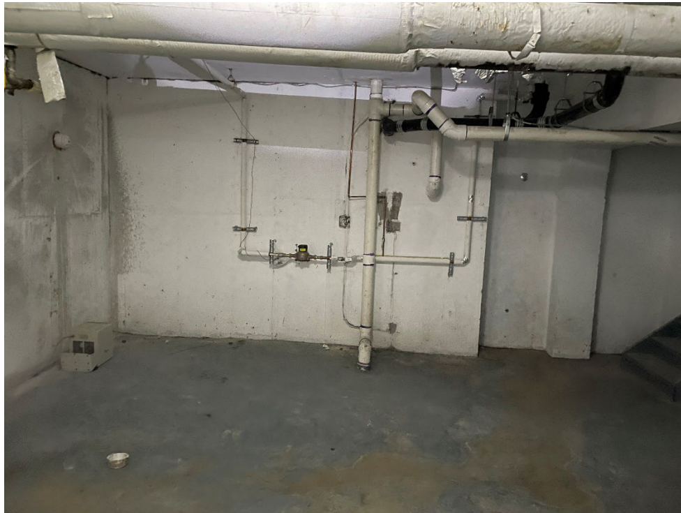
Photo 14: Photo showing Blower B exposed piping in cellar and inspecting. SVMP-B5 to the left and suction points MG-13 and -14.
