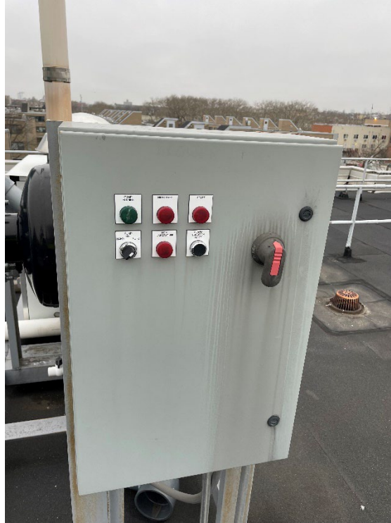
Photo 3: View of Blower B SSDS control panel.
