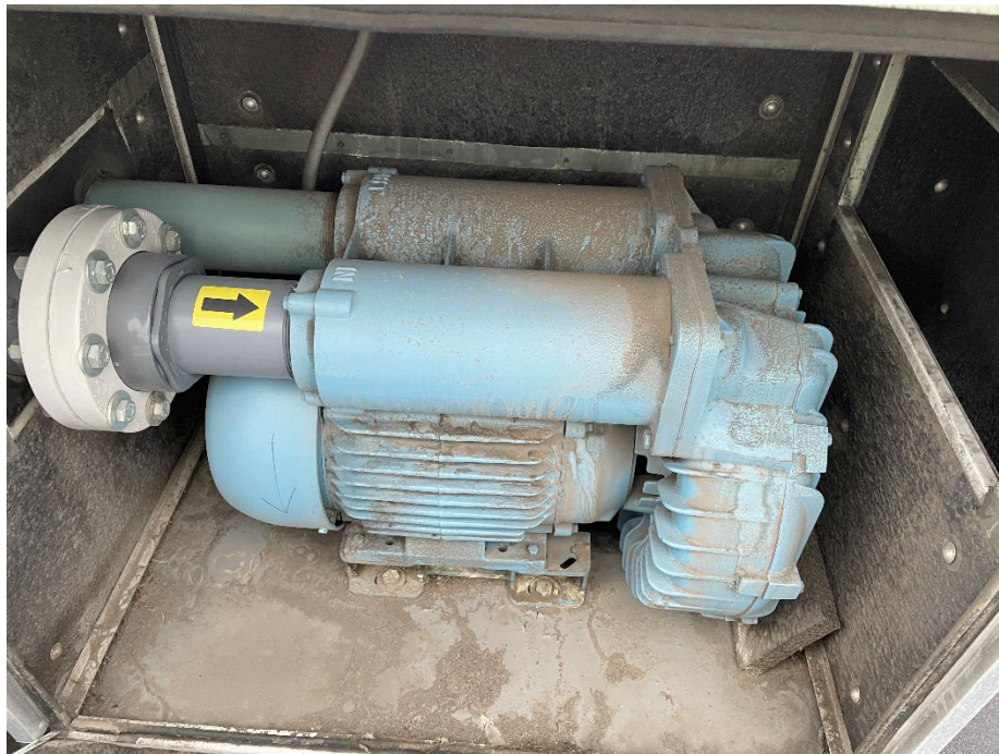
Photo 4: View of Blower B blower fan.
