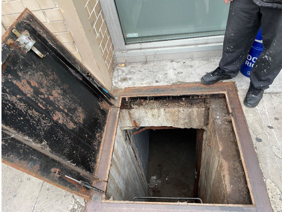
Photo 11: Sidewalk vault leading to exposed SSDS and monitoring points related to Building B blower (southern basement area).
