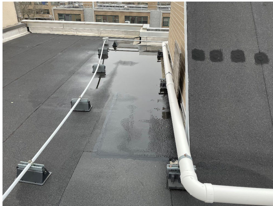
Photo 8: Looking north, photo showing SSDS piping run along the roof with legs leading towards the residential building side.
