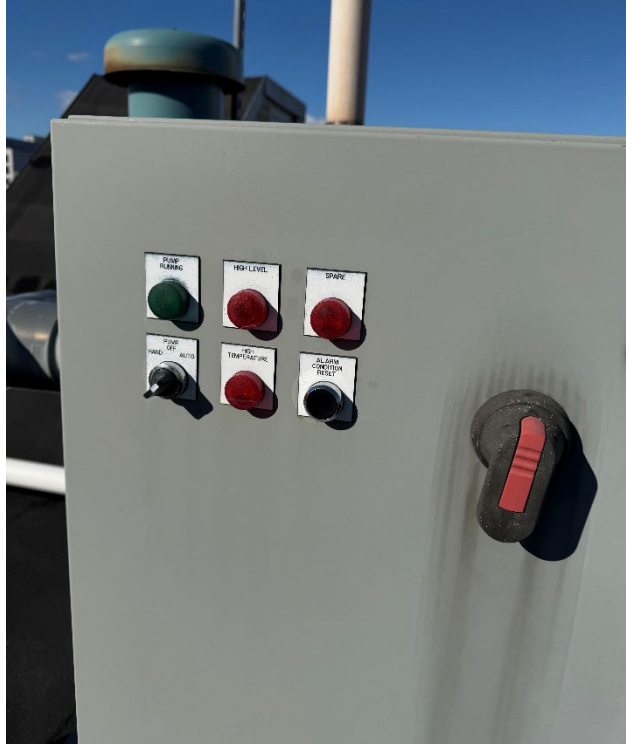
Photo 1: View of Blower B (northern) SSDS control panel.
