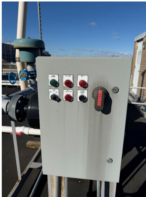
Photo 2: View of Blower A (southern) SSDS control panel.
