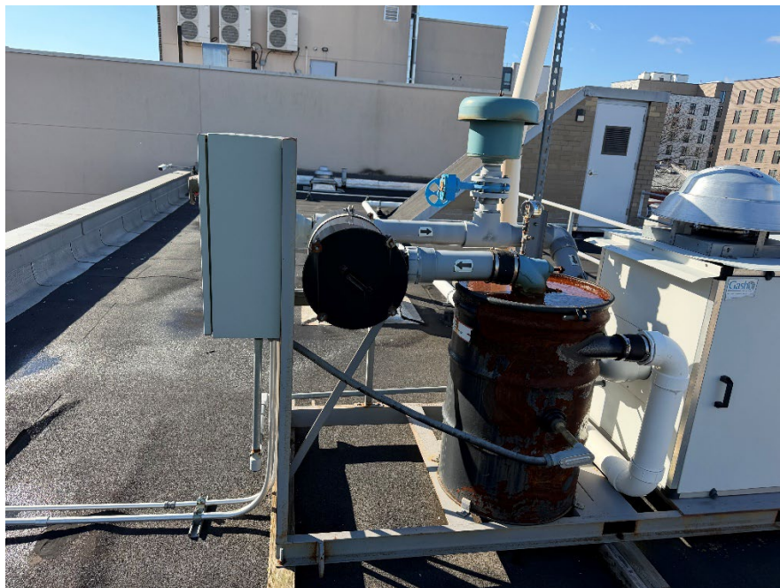
Photo 14: Photo of knockout/condensate tank on the Blower A unit.
