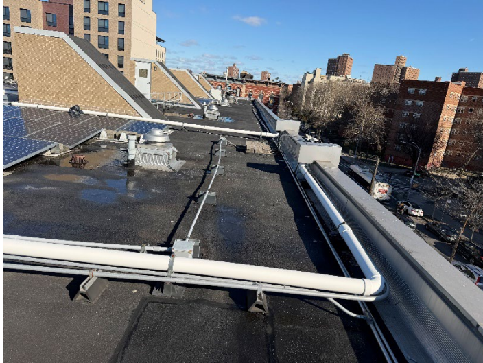
Photo 5: Photo of SSDS piping along Rockaway Avenue.
