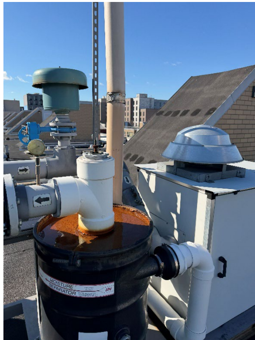
Photo 4: Photo of knockout/condensate tank influent gauge on the Blower A unit.
