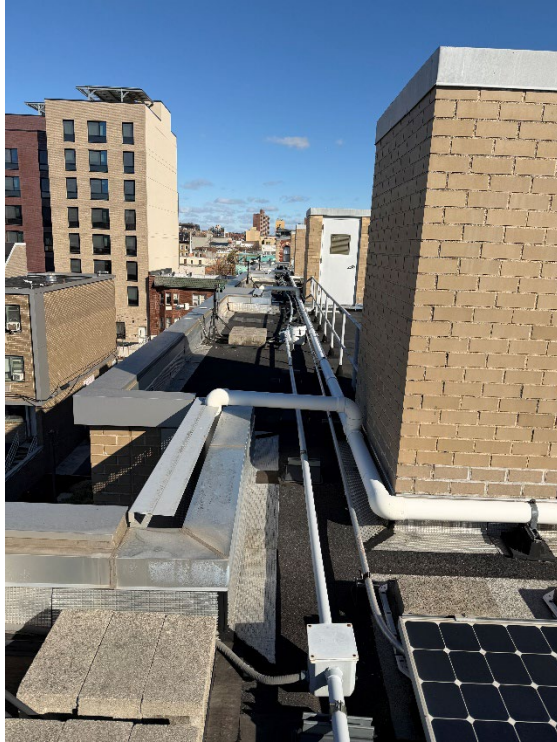
Photo 7: View showing Blower A SSDS piping run along the roof with legs heading down the side of the building.
