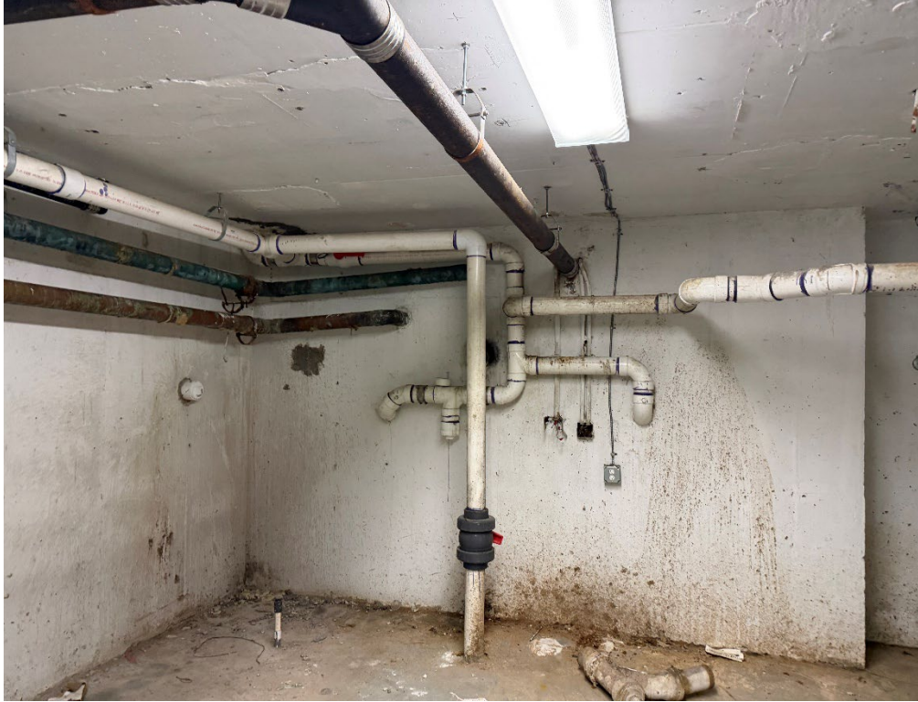
Photo 9: View of SSDS blower legs in the southern basement area.
