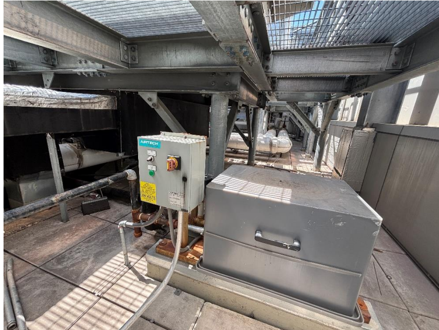
Photograph 7: View of blower box on the building roof (04/14/2026)
