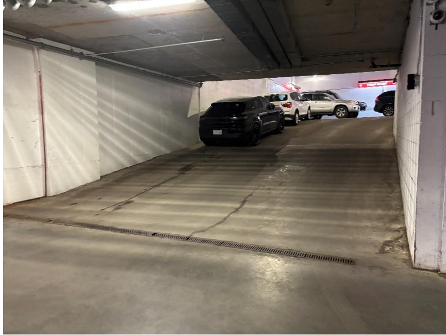
Photograph 5: View of example trench drain located within the cellar level ventilated parking garage (04/14/2026)
