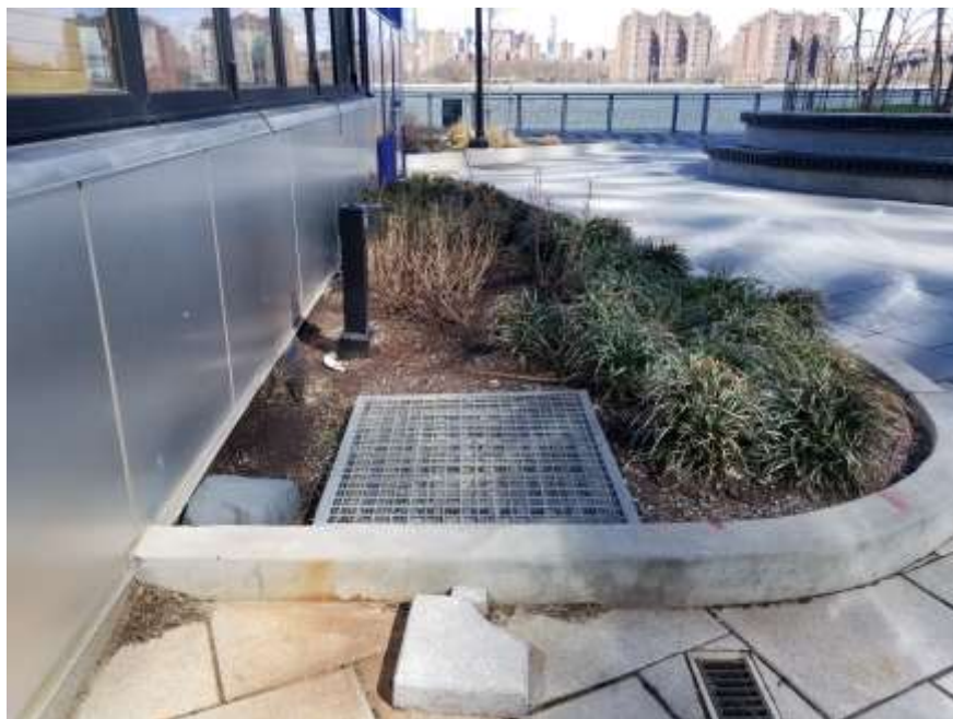
Photograph 8: View of the composite cover in a landscaped area in the northwest part of the site (03/29/2021)
