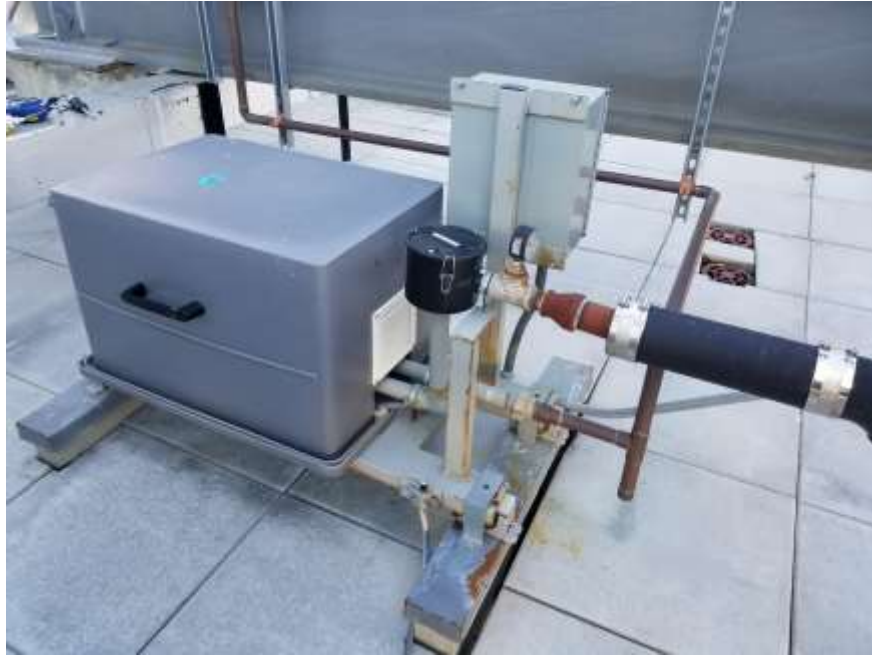
Photograph 7: View of blower box on the roof of the building, facing west (03/29/2021)
