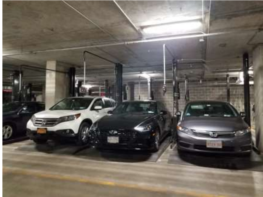
Photograph 3: Example view of car stackers in the cellar level ventilated parking garage (03/29/2021)
