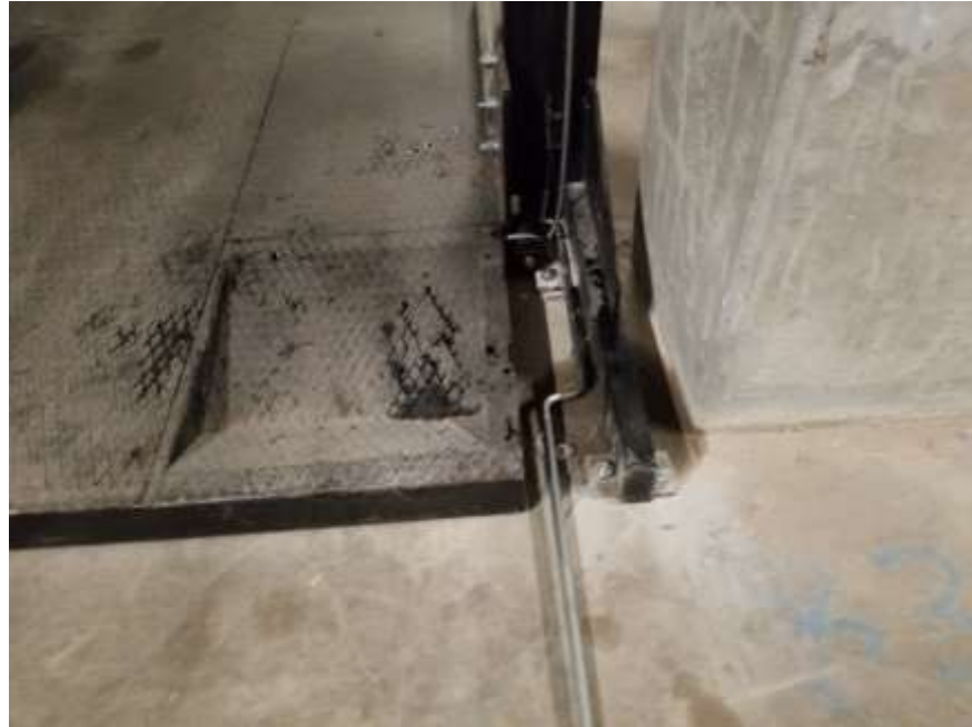
Photograph 5: Area of minor staining observed in the cellar level ventilated parking garage; stain related to hydraulic fluid from a car stacker (03/29/2021)
