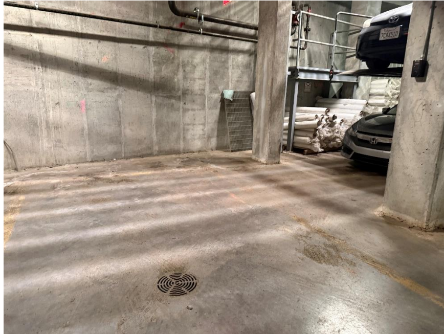
Photograph 3: Example floor drain in the cellar level ventilated parking garage (04/14/2026)
