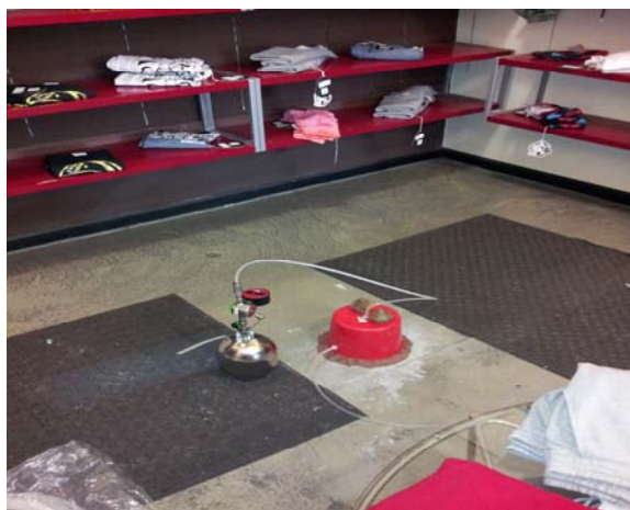
Photo 5: Sub-slab vapor sample point assembly.
