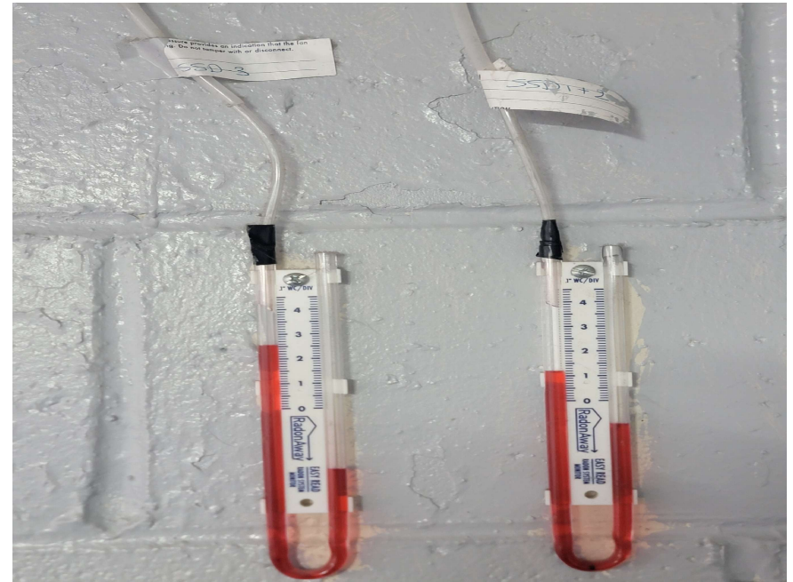
Vacuum monitoring U-Tube at SSDS 1 & 2 and at SSDS-3
