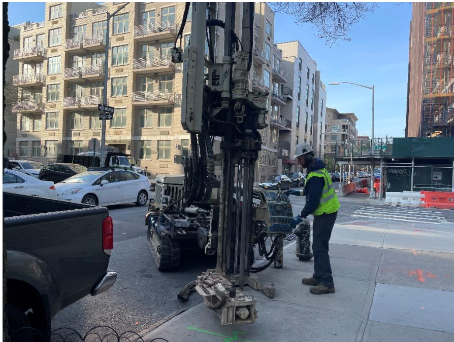
Photograph 2: Eastern Environmental Solutions, Inc. (Eastern) advancing soil vapor sampling location SV05 with a Geoprobe® 7822 DT track-mounted drill rig (facing south).
