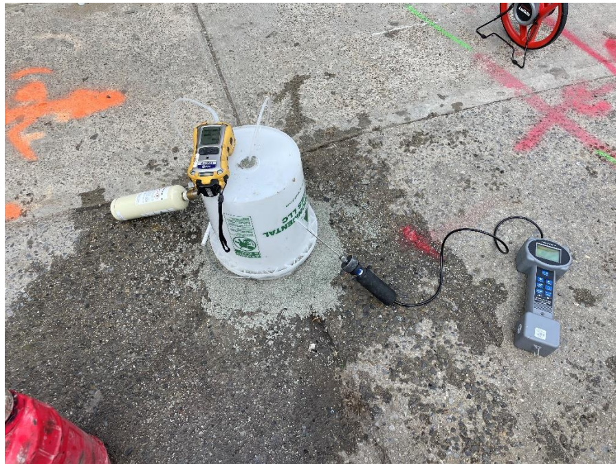
Photograph 4: Langan field engineer conducting a helium test on soil vapor point SV05 prior to sampling.
