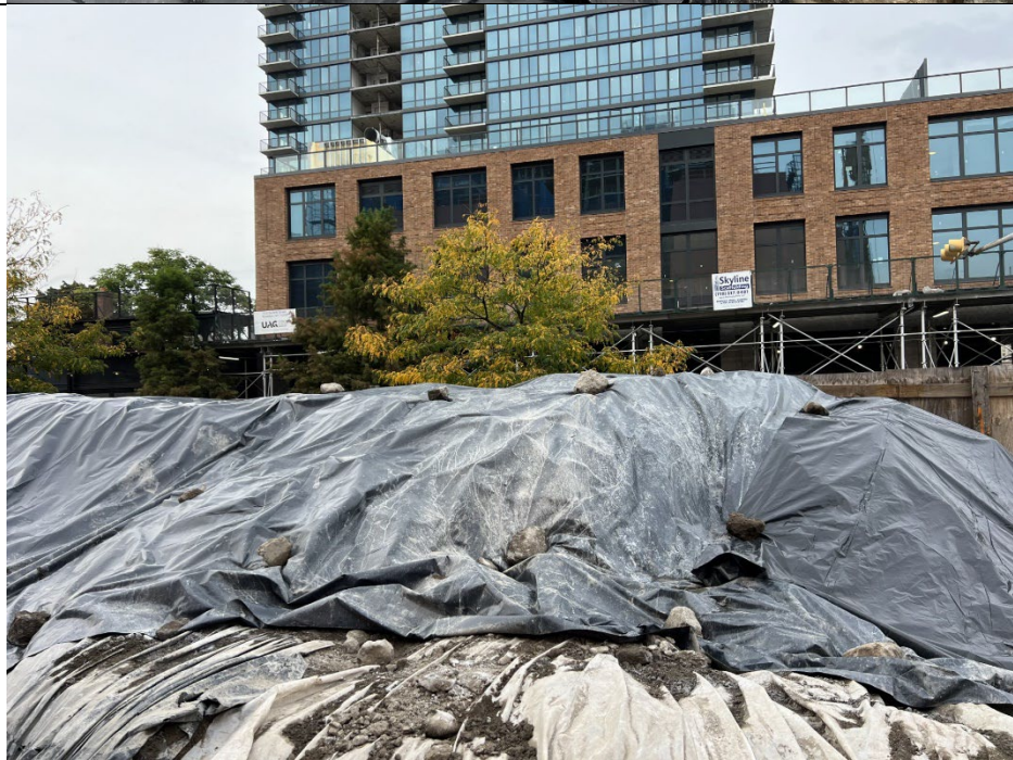
Photo 4: Poly coverage on top of spoils within berm at the end of the day after being secured, facing north.
