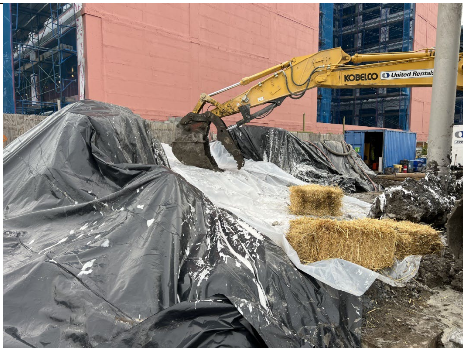
Photo 3: Poly sheeting is placed atop of ISS spoils and secured at the end of the day, facing southwest.
