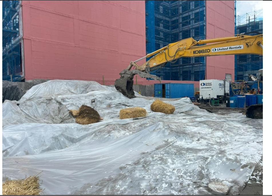
Photo 5: Poly sheeting is placed on top of ISS work area and secured with weights at the end of the day, facing southwest.
