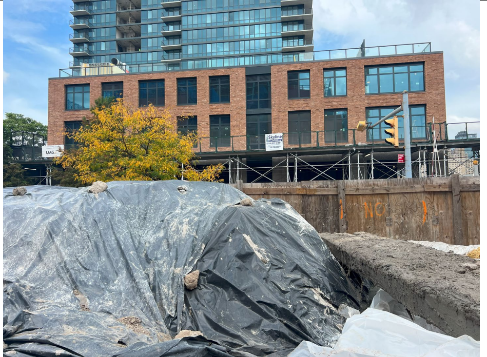
Photo 4: Poly sheeting is placed atop of ISS spoils and secured at the end of the day, facing northwest.
