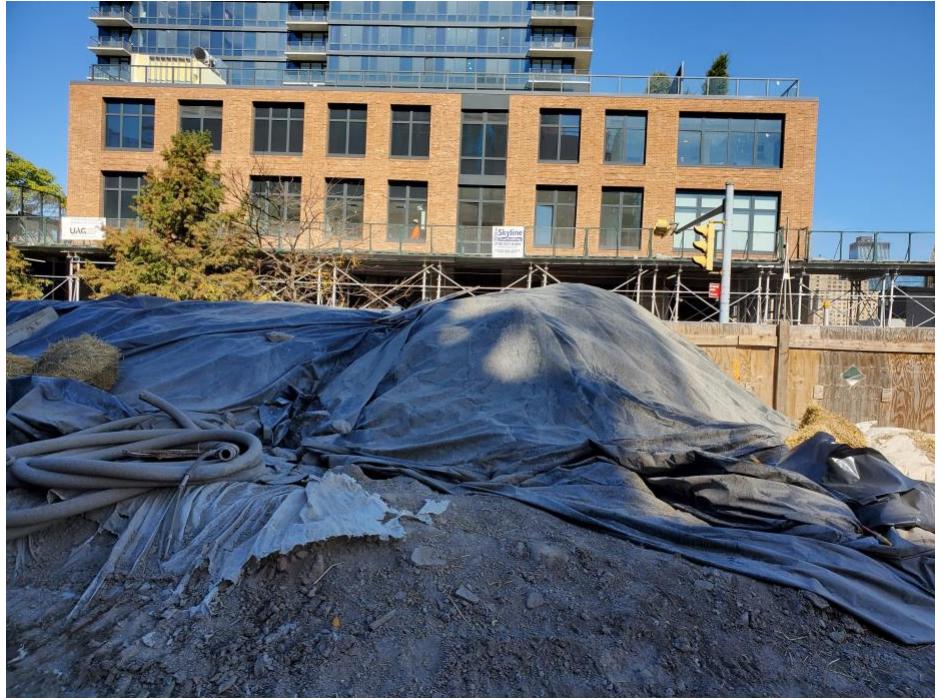
Photo 5: Poly sheeting placed on top of berm with ISS material and secured at the end of the day, facing north.
