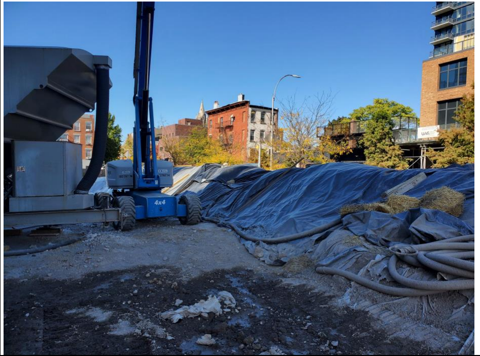
Photo 3: Poly sheeting placed atop ISS spoils and secured at the end of the day, facing northwest.
