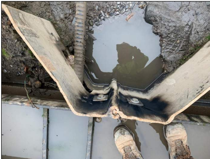
Photo 2: General view of bolt installation along the deadman wale and sheet piles.
