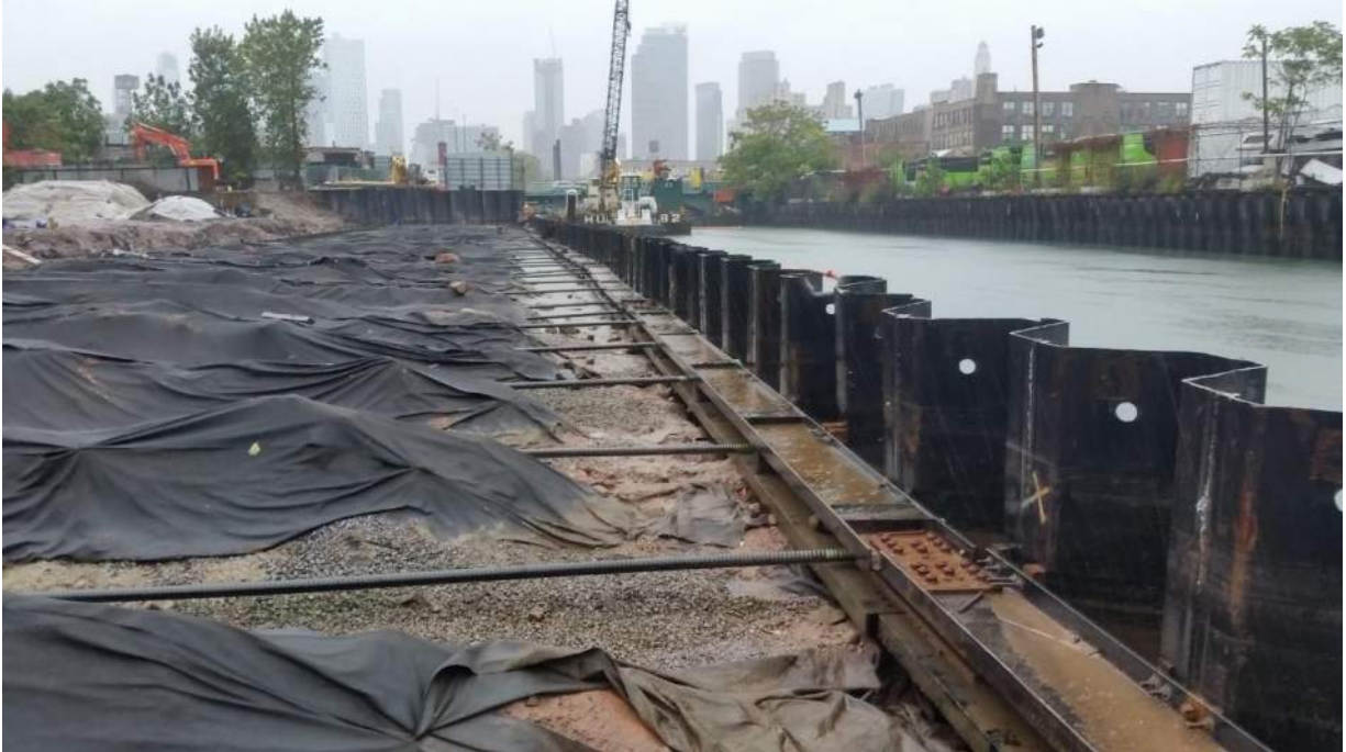
Photo 1: General view of bulkhead installation progress along the eastern site extent (facing north)
