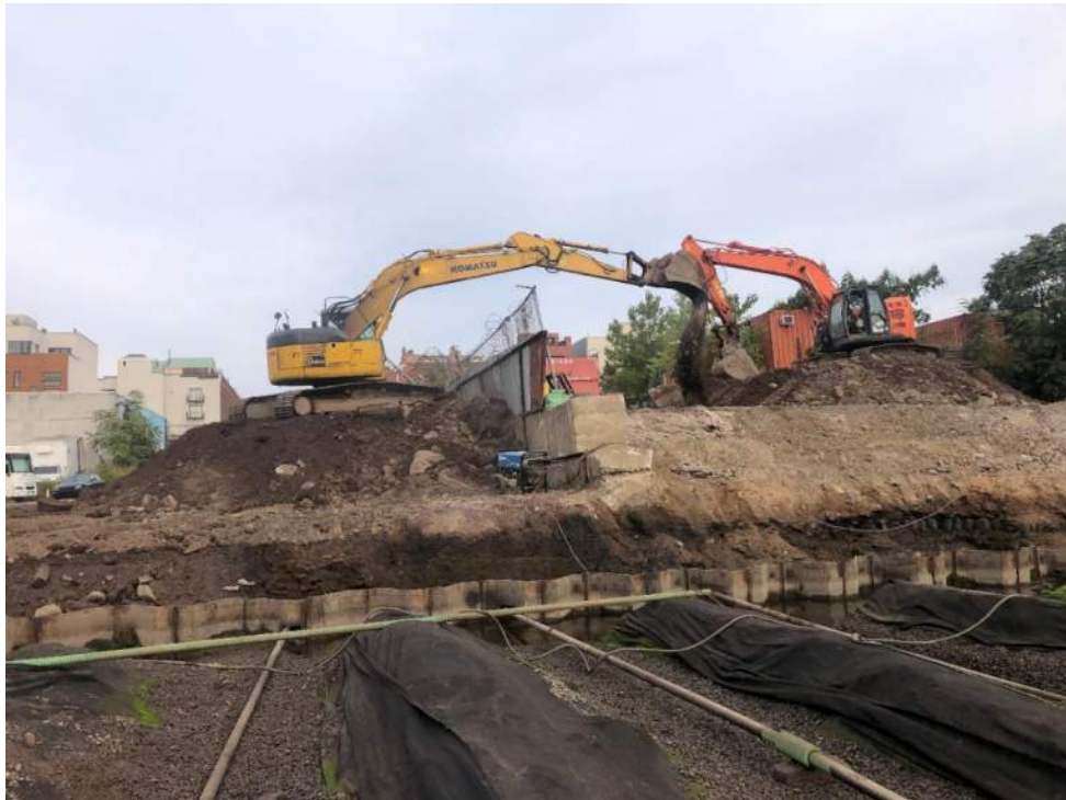
Photo 2: View of A-Construction relocating soil to the stockpile on Lot 3 in preparation for off-site disposal (facing west).
