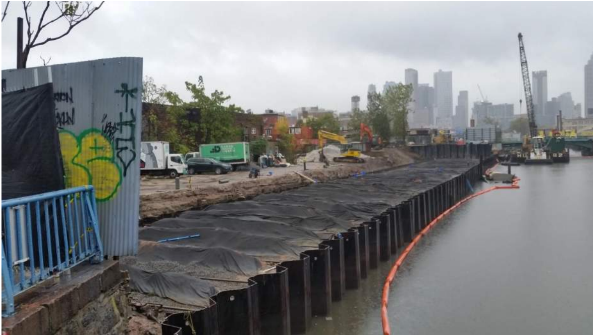
Photo 1: General view of bulkhead installation progress along the eastern site extent (facing north).
