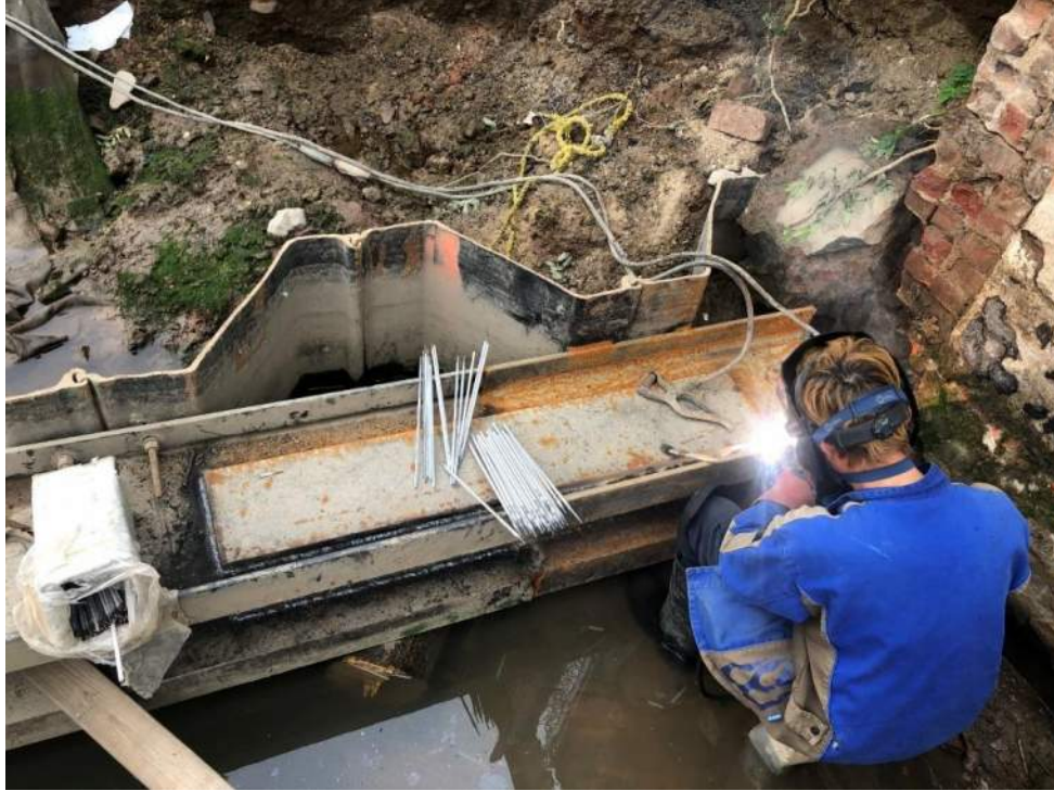
Photo 1: View of Agra welding splice plates at south end of deadman wale no. 1 (facing east).
