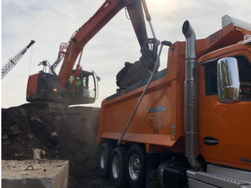
Photo 3: View of non-hazardous soil/fill being loaded into permitted tri-axle trucks for off-site disposal (facing east).
