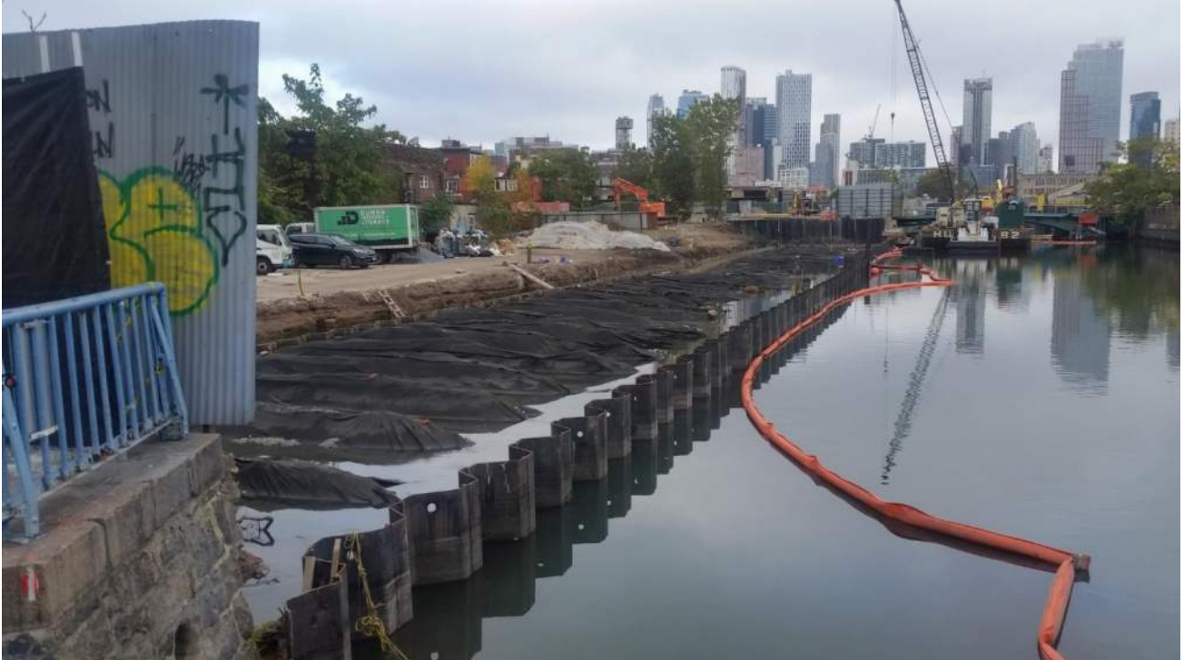
Photo 1: General view of bulkhead installation progress along the eastern site extent (facing north).
