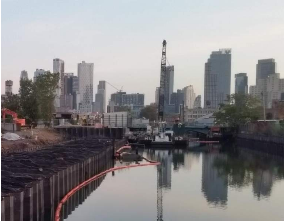
Photo 1: General view of bulkhead installation progress along the northeast region of the site (facing north).
