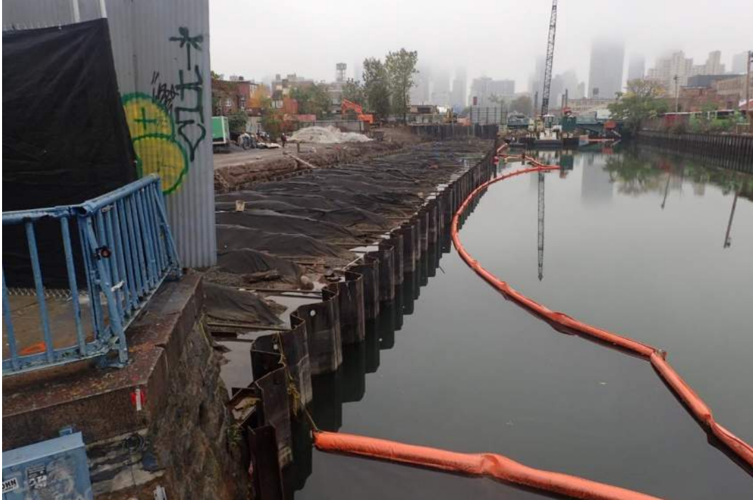
Photo 1: General view of bulkhead installation progress along the eastern site extent (facing north).
