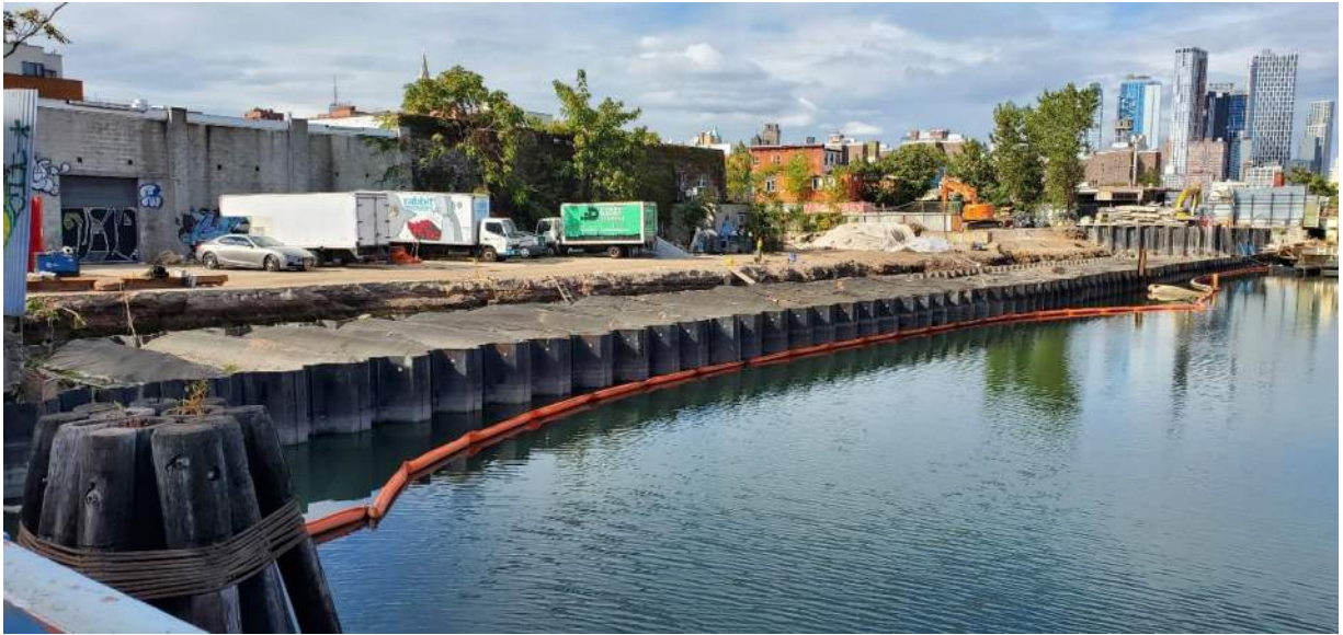
Photo 3: View of the site at the end of the day from the Carroll Street Bridge (facing west).
