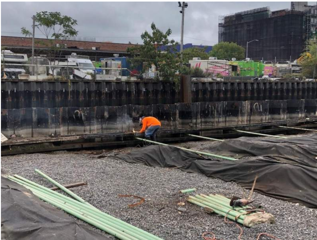
Photo 2: View of Agra welding stiffener plates to bulkhead wale no. 5 facing east).
