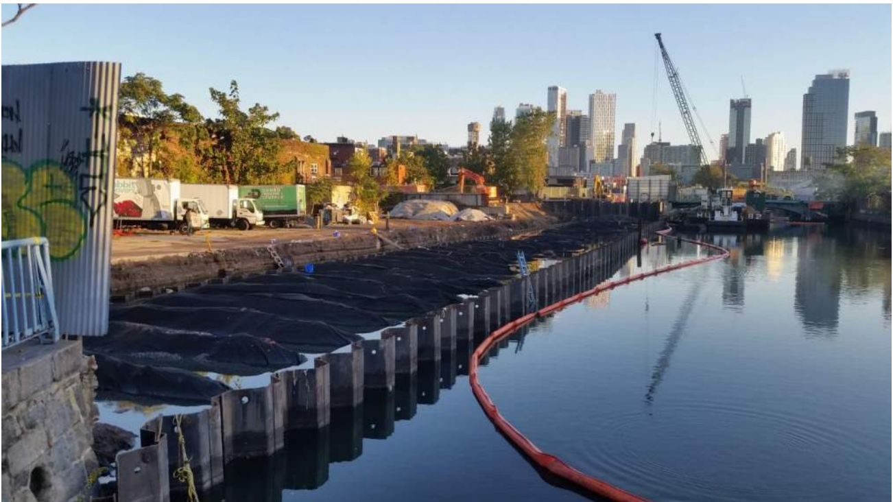
Photo 2: View of the bulkhead installation progress from the Carroll Street Bridge (facing northwest).
