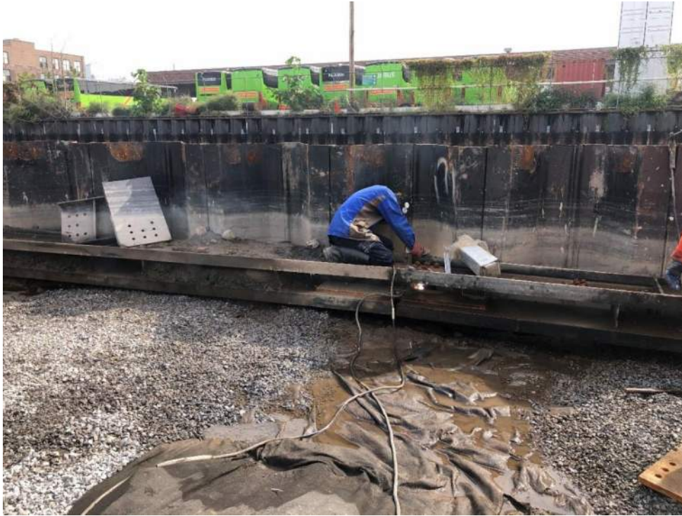
Photo 1: View of Agra welding splice plates between bulkhead wale nos. 6 and 5 (facing east).
