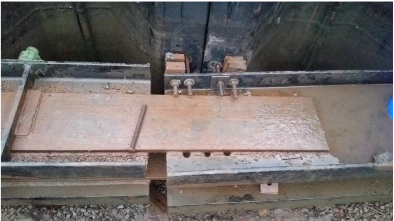
Photo 2: View of washer, bolt, and shim installation between a bulkhead sheet pile and wale (facing east).
