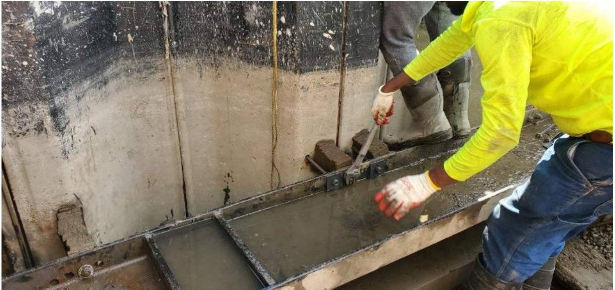
Photo 1: View of Agra installing bolts at the north end of bulkhead wale no. 9 (facing east).
