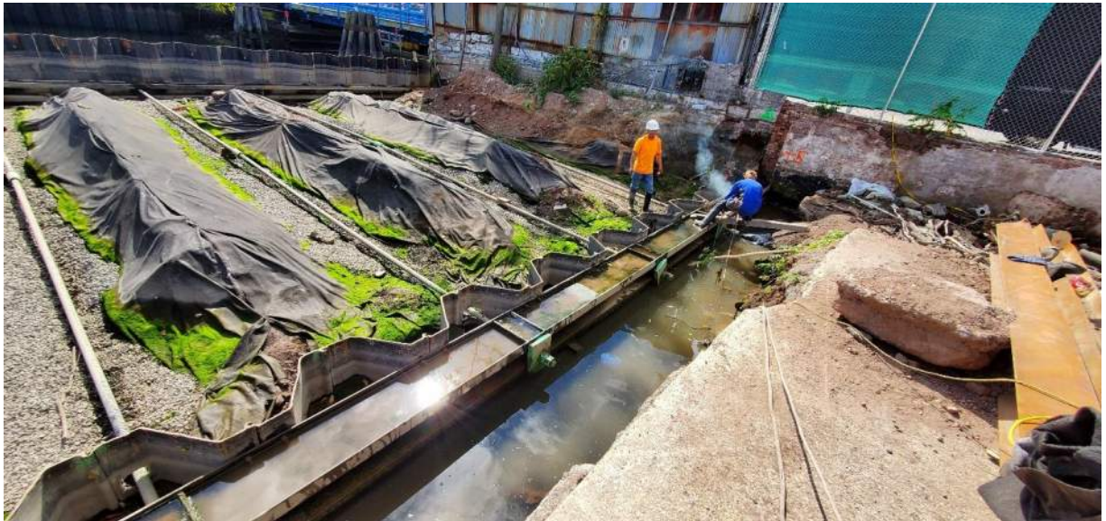
Photo 2: View of Agra tact welding anchor plates at the southern end of deadman wale no. 1 (facing south).
