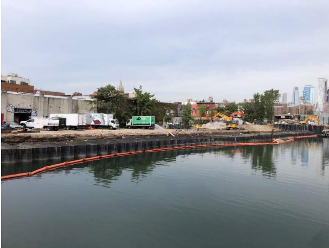
Photo 3: View of the site at the end of the day from the Carroll Street Bridge (facing west).
