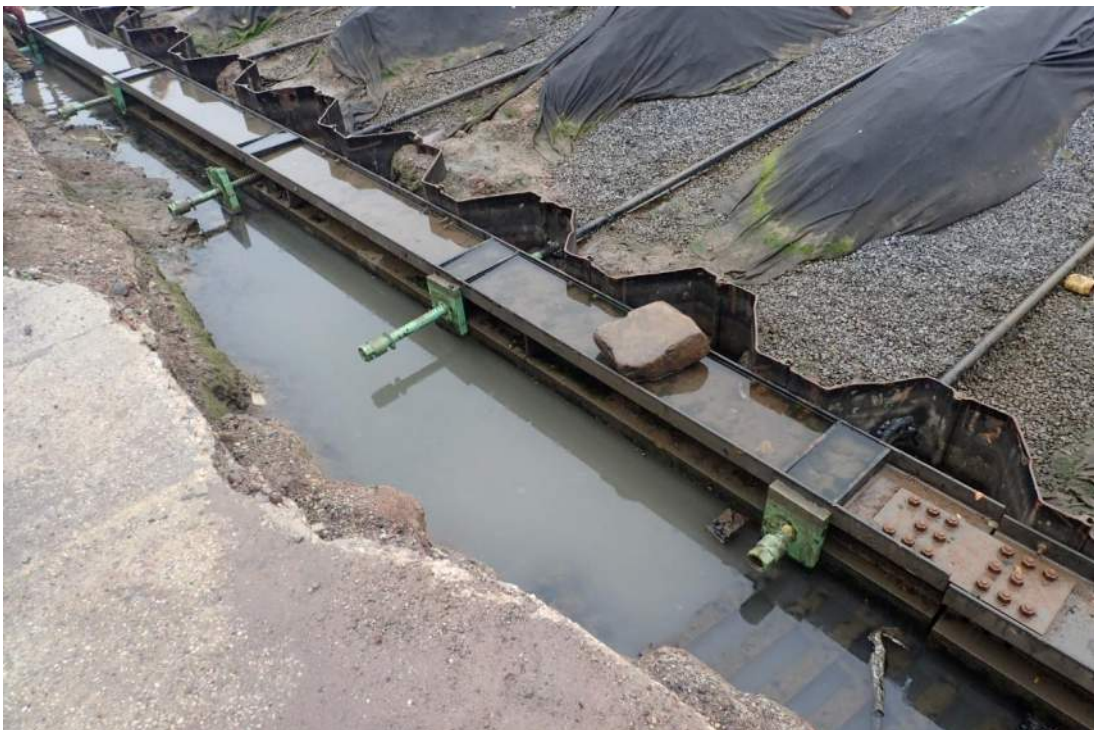
Photo 2: View of tie rod installation progress along the deadman sheet piles (facing northeast).
