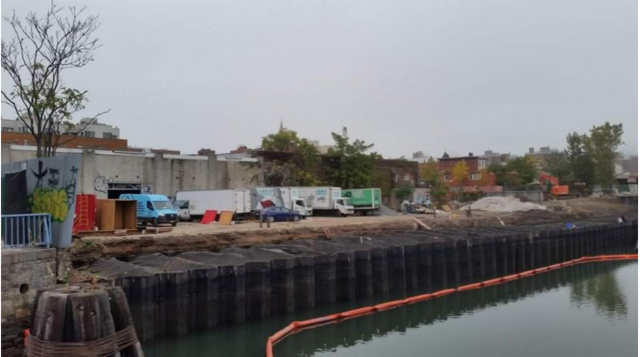
Photo 1: General view of bulkhead installation progress along the eastern site extent (facing north).
