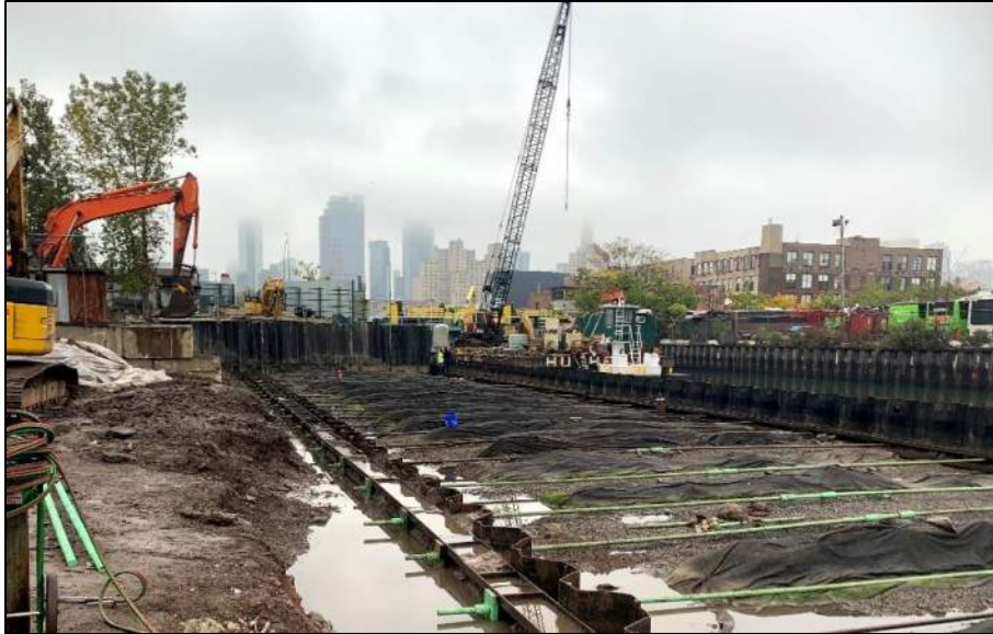
Photo 1: General view of bulkhead installation progress along the eastern site extent (facing northeast).
