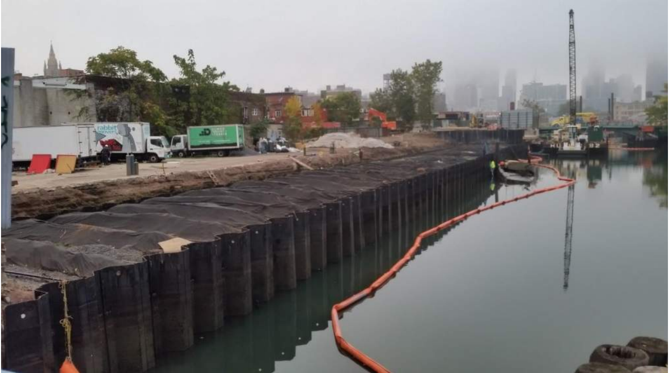
Photo 1: General view of bulkhead installation progress along the eastern site extent (facing north).
