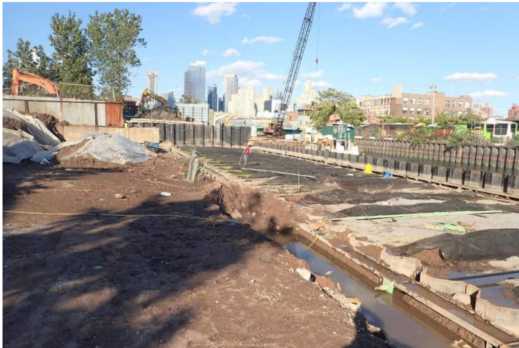
Photo 2: View of the bulkhead installation progress in the northern region of the site (facing northeast).
