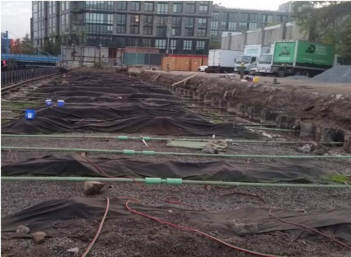
Photo 1: General view of tie rod installation in the central-east region of the site (facing south).
