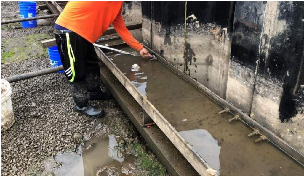
Photo 1: View of Agra adjusting the bolts and installing washers on bulkhead wale no. 8 (facing north).
