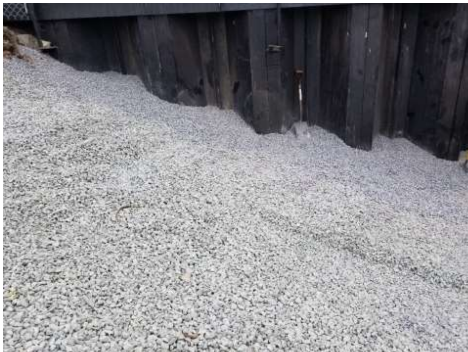
Photo 2: View of 6-inch lift of ASTM #57 ¾-inch crushed stone placed over previously compacted recycled engineered fill (facing north).
