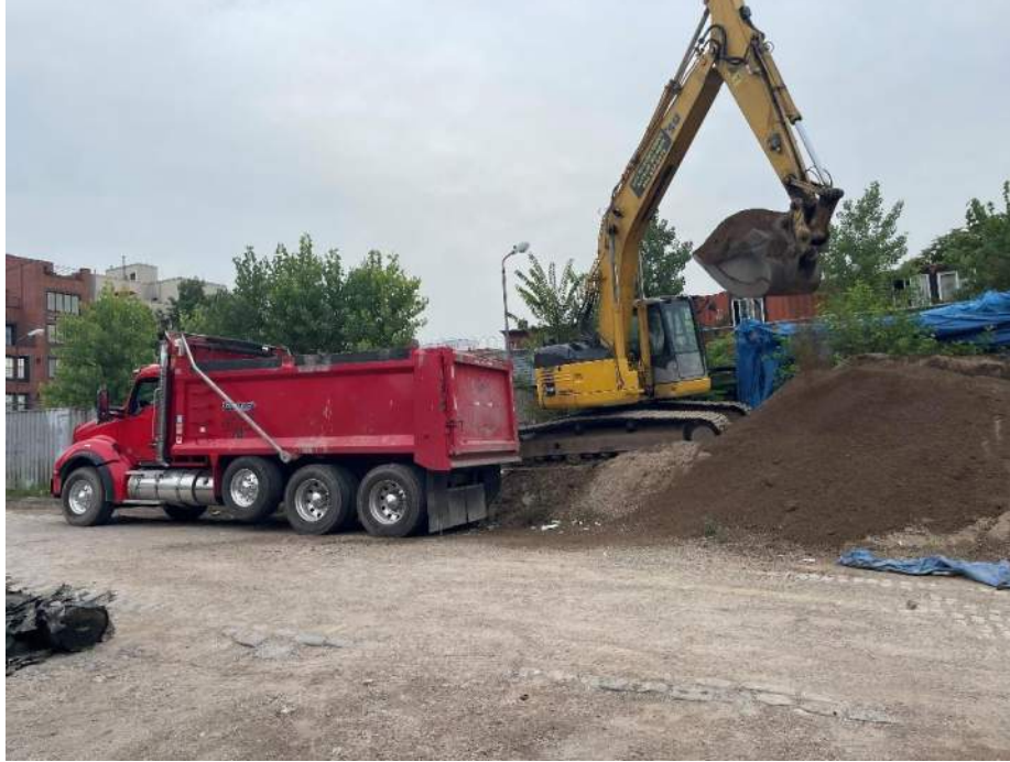
Photo 1: View of Maspeth Masonry loading stockpiled soil/fill into a permitted tri-axle truck for off- site disposal (facing north).
