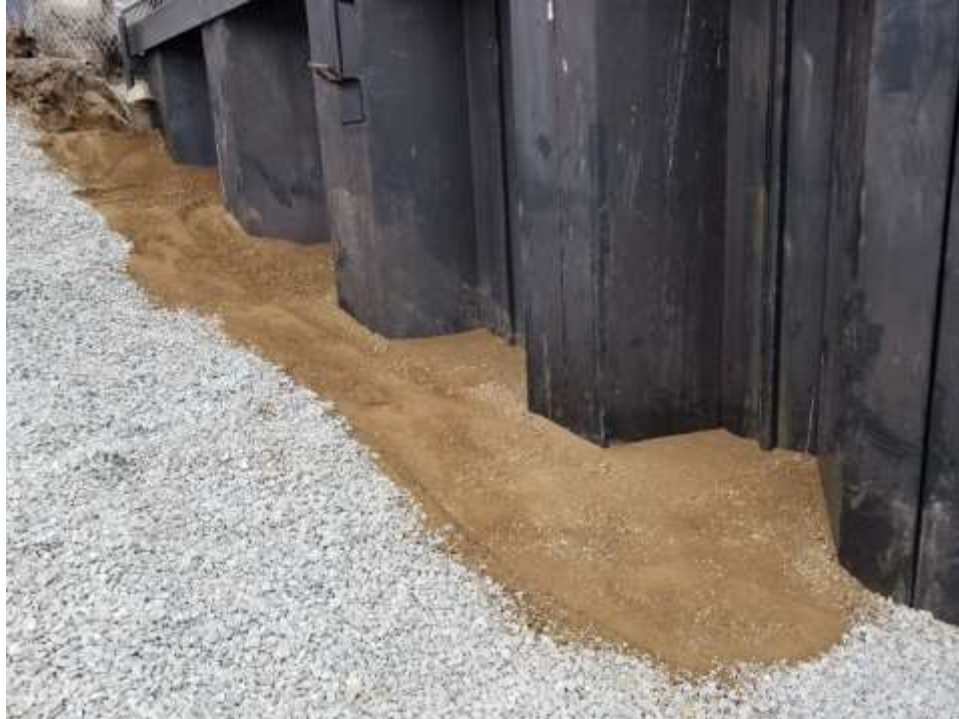
Photo 1: View of compacted final 8-inch lift of recycled engineered fill along the closure wall in the northern part of Lot 3 (facing northwest).
