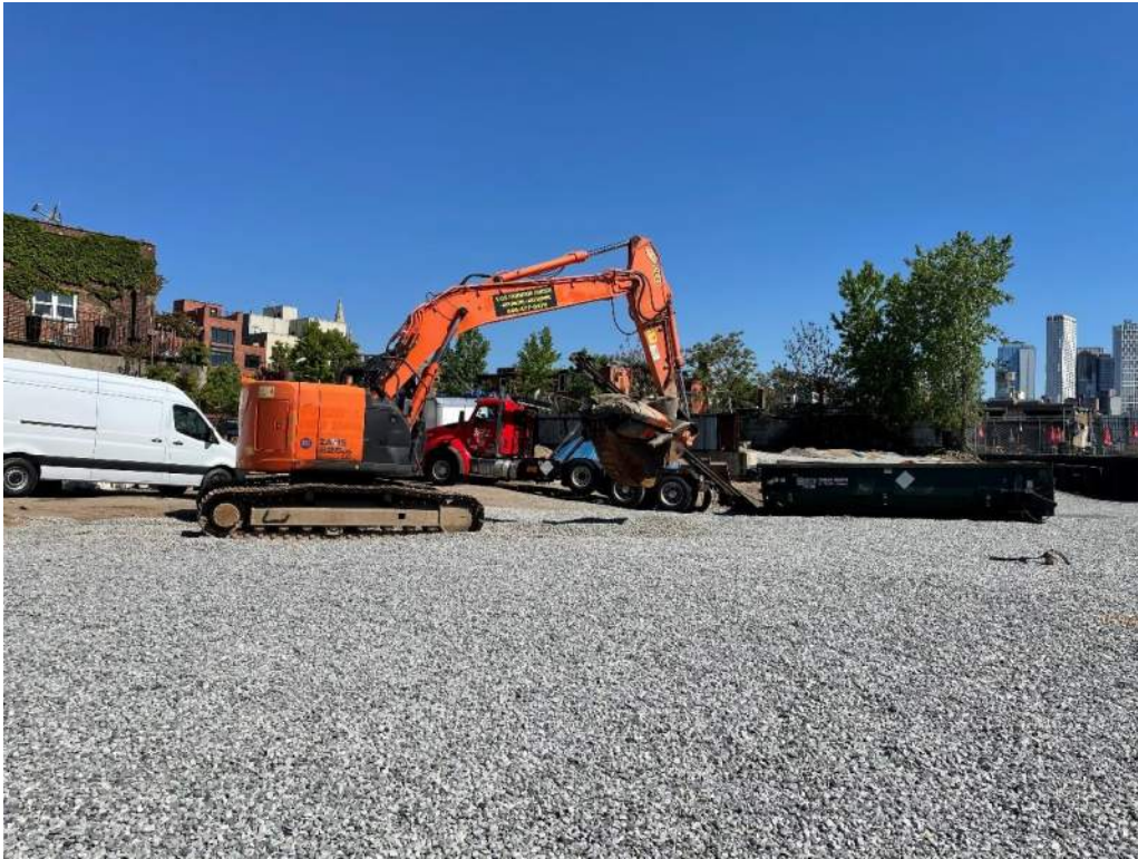
Photo 1: View of Maspeth Masonry using a Hitachi 225US Excavator to load the spent turbidity curtain into a permitted tri-axle truck for off- site disposal (facing north).
