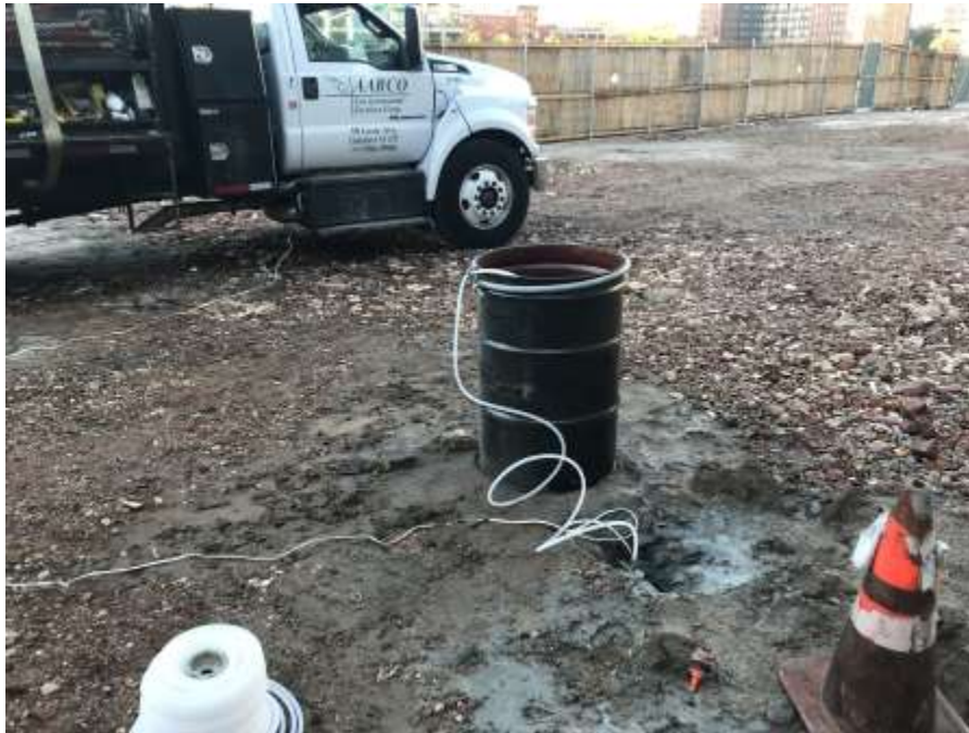
Photo 1: AARCO developing monitoring well MW-202 (facing south).
