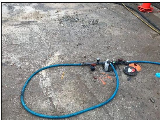
Photo 3: Typical setup of an Injection Well being pumped on with safety valves and pressure gauge.
