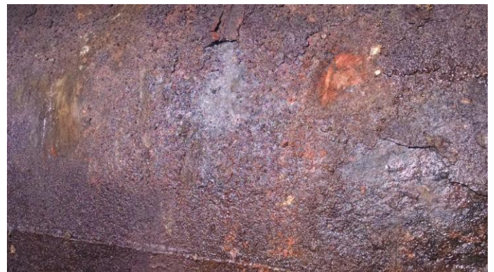
Photo 12: Tank 2 Very Rusty but no holes
