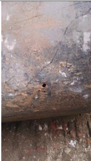
Photo 5: Small hole Tank 1 – No visual leakage
