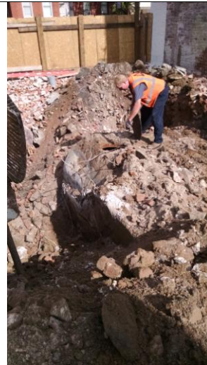
Photo2: Pump out Tank 1
