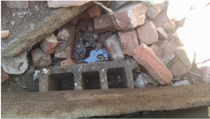
Photo 13: Tank 2 small amount of oil on fmr vault slab
