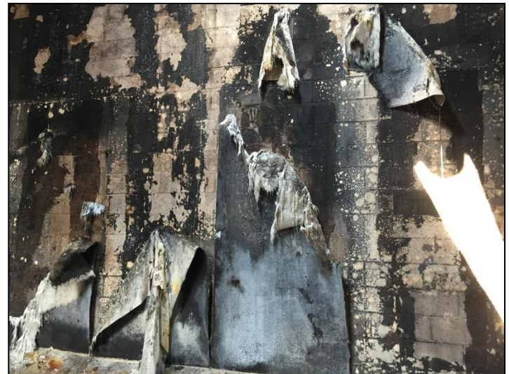
Photograph 8: Fire damage to the eastern portions of the Site buildings.
