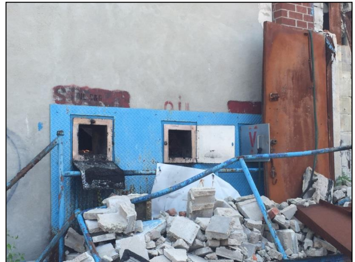
Photograph 4: Former apparent fuel oil fill ports on the eastern portion of the Site.
