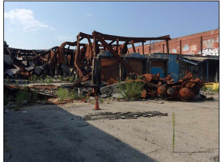
Photograph 2: Former receiving area on the central portion of the Site, facing south.
