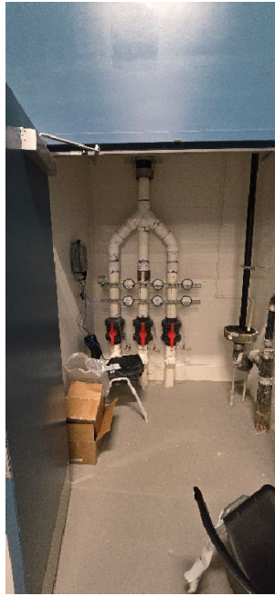
20 - SSDS manifold in the southeastern manifold closet.
