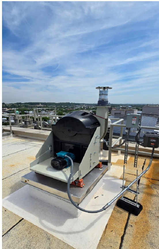
21 - SSDS fan and exhaust on the roof.
