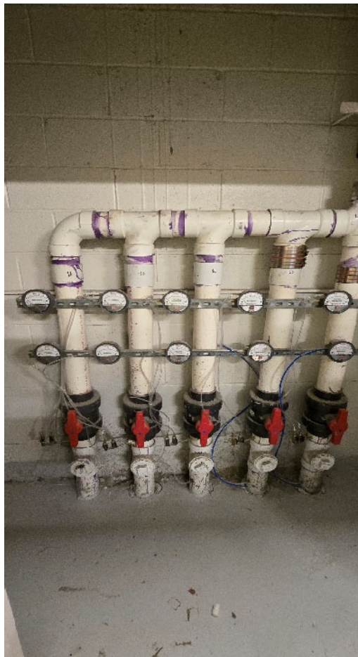
14 – SSDS gauges in the west manifold closet.
