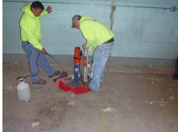
PAL coring through the basement slab for the collection of soil and groundwater samples
