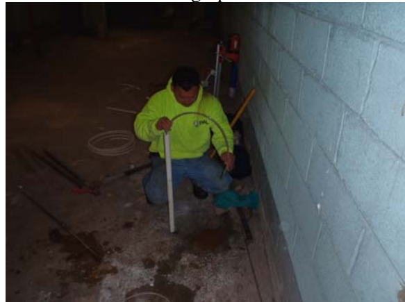
Temporary well point installed in SB01 for the collection of a groundwater sample
