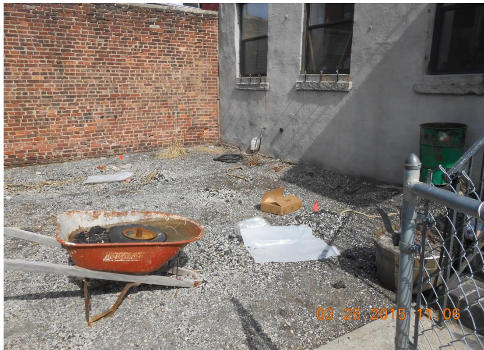
Photograph 10: View of soil sample locations P001-SS005 and P001-SS006 prior to sample collection.
