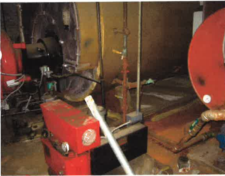
BOILER IN BASEMENT OF LARGE BUILDING
