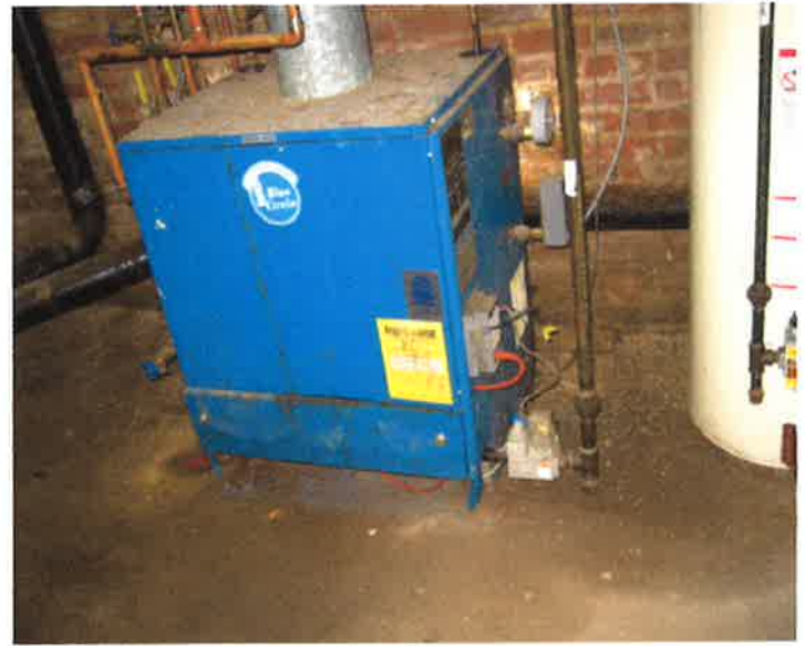
BOILER IN SMALLER BUILDING
