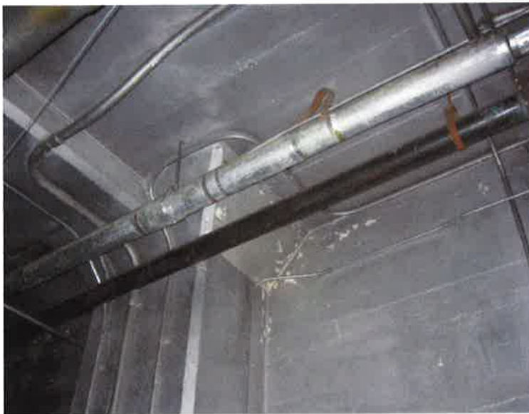
PACM ON PIPES IN BASEMENT
