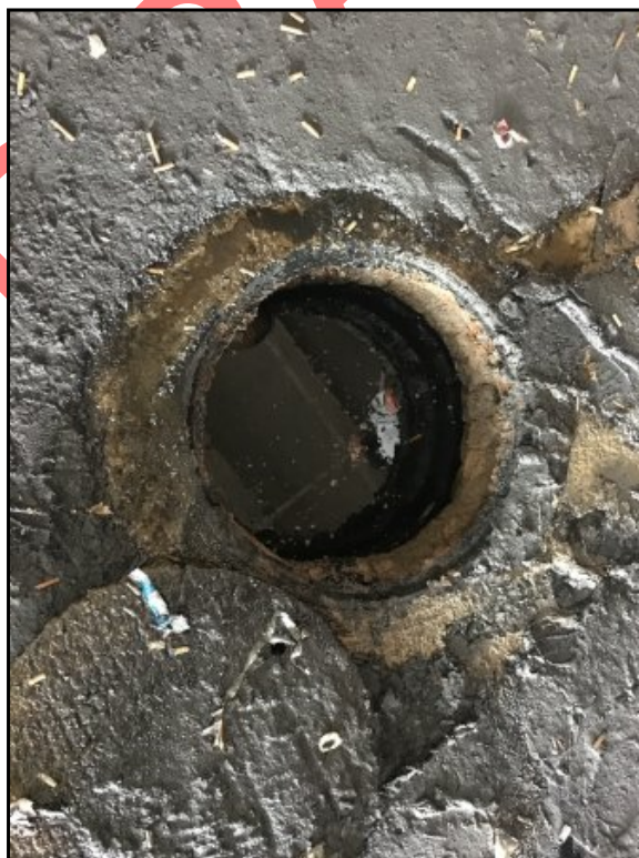
14 : Catch basin filled with mostly hydraulic oil
