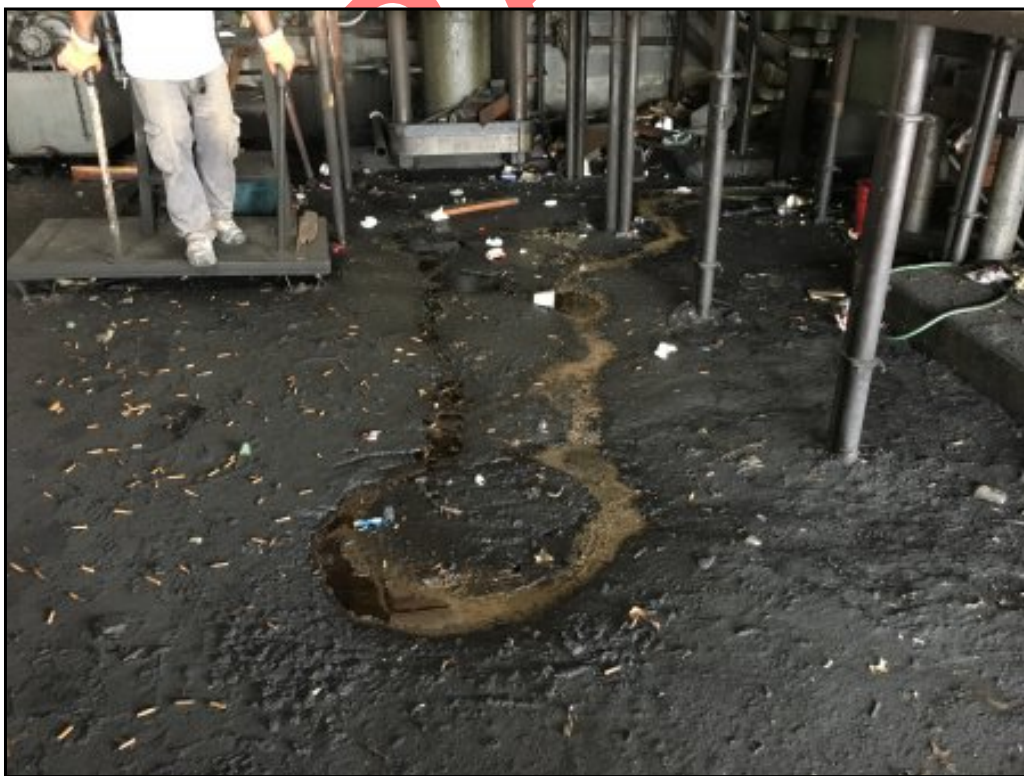
12 : View of hydraulic oil leak area at NE corner of Property
