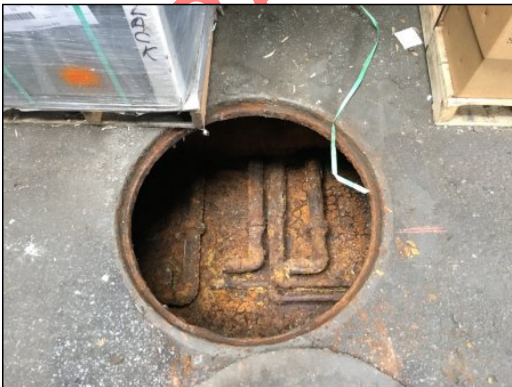
2 : View of suspected ~5,000-gal UST beneath manhole cover
