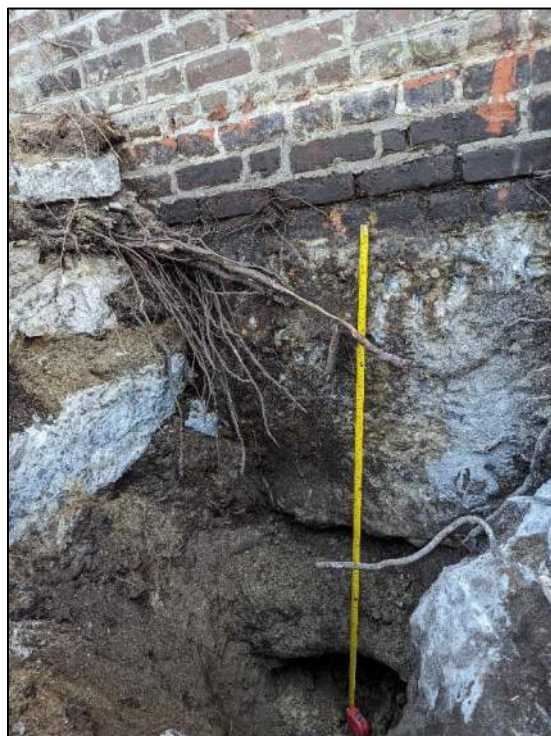
Photo 2: View of footing under 1-story portion of building in test pit TP-1 (facing east).
