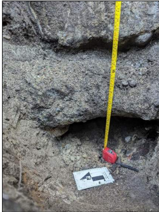
Photo 3: View of footing bottom under 1-story portion of building in test pit TP-1 (facing southeast).
