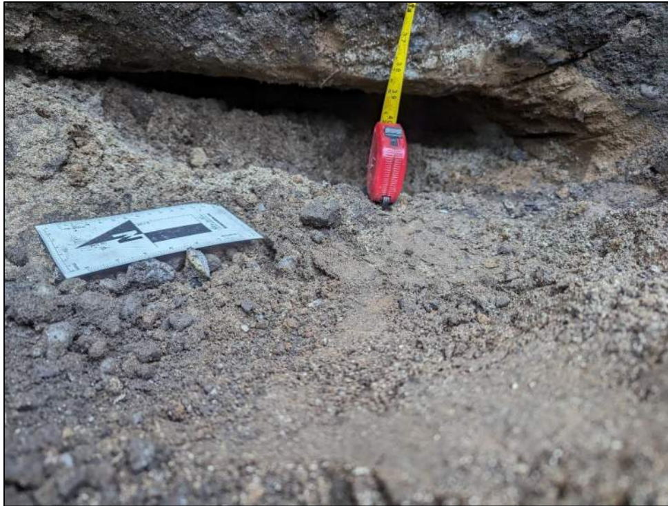
Photo 5: View of footing bottom under 2-story portion of building in test pit TP-1 (facing southeast).
