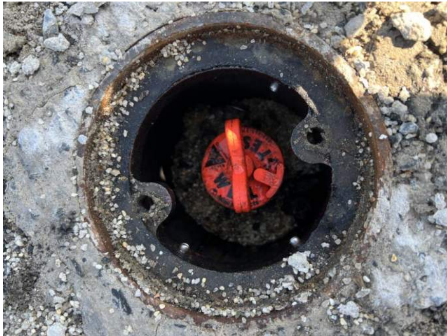
Photo 2: J-Plug condition of well MW-03S.
