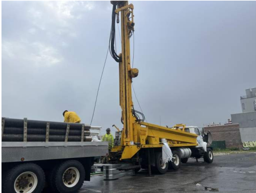
Photo 1: Coastal advancing soil boring SBD09 in the western part of the site (facing east)
