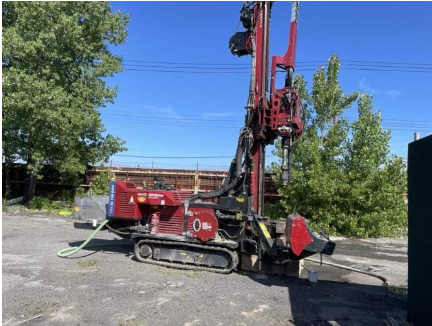
Photo 1: Coastal advancing soil boring SBD02 in the western part of the site (facing west)
