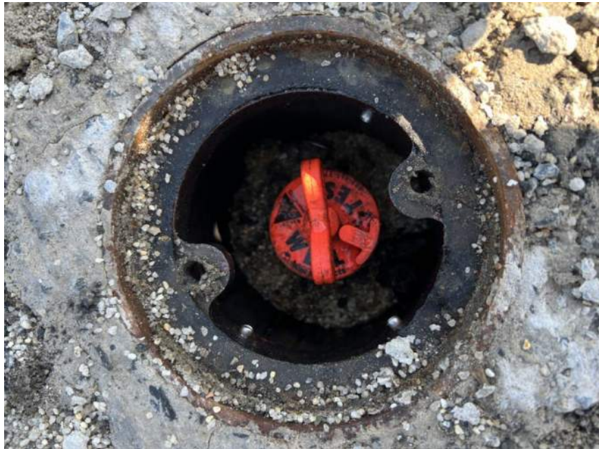
Photo 2: J-Plug condition of well MW-03S.
