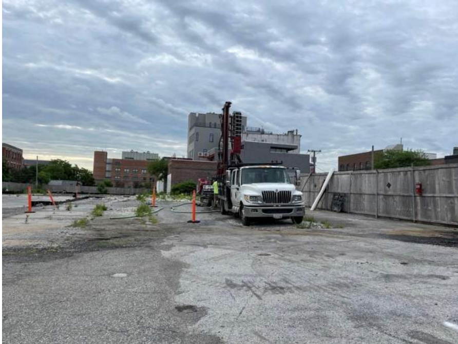
Photo 1: Coastal advancing soil boring SB05 in the western part of the site (facing south)
