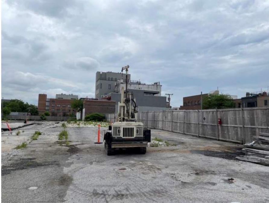
Photo 1: Coastal advancing soil boring SBT-E in the western part of the site (facing south).
