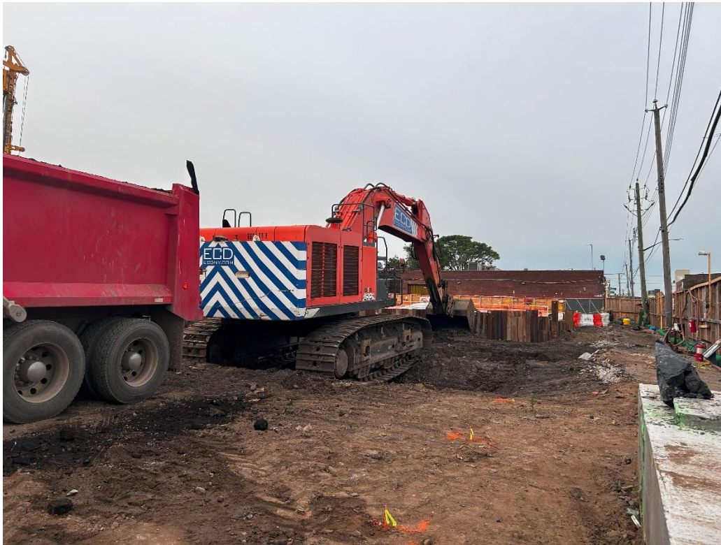
Photo 1: View of ECD live-loading hazardous non-native material in the northwestern part of the site (facing west)
