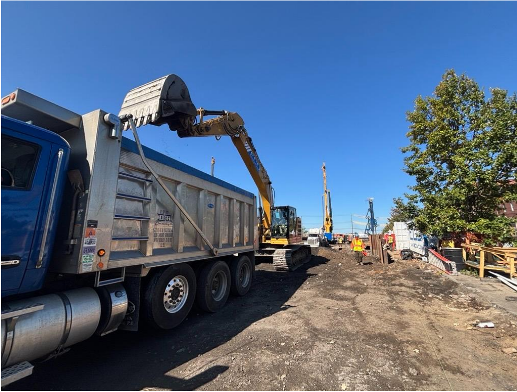
Photo 1: View of ECD live-loading hazardous non-native fill in the central part of the site (facing north)
