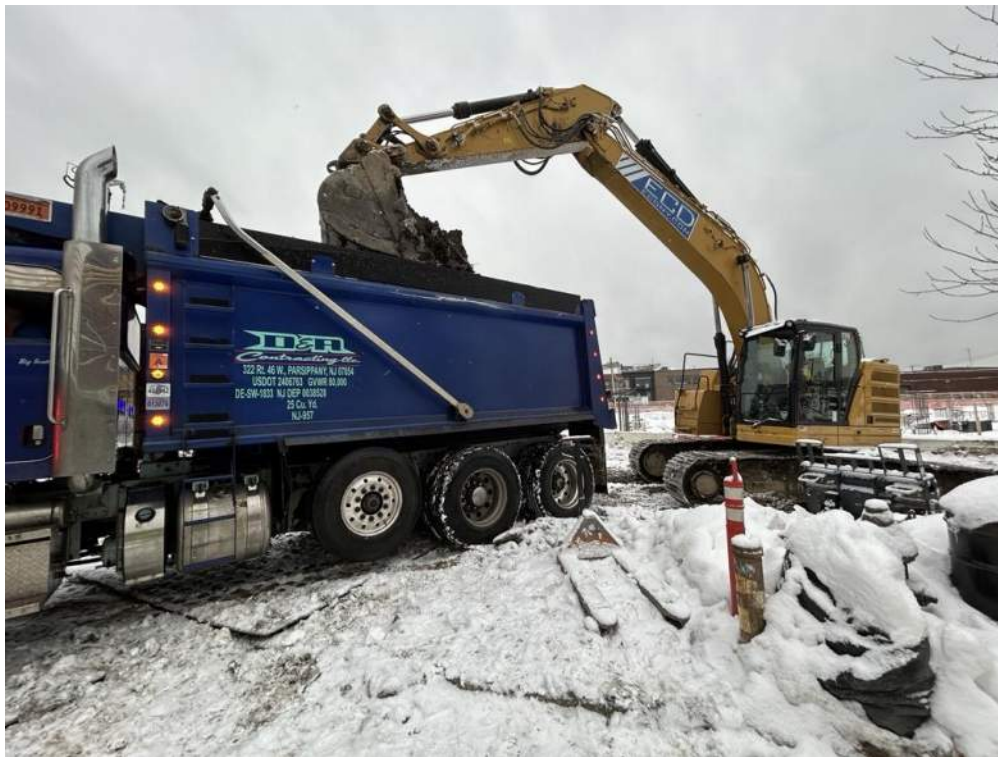
Photo 1: ECD loading a permitted tri-axle truck with non-hazardous non-native fill from the central part of site for off-site disposal (facing west)
