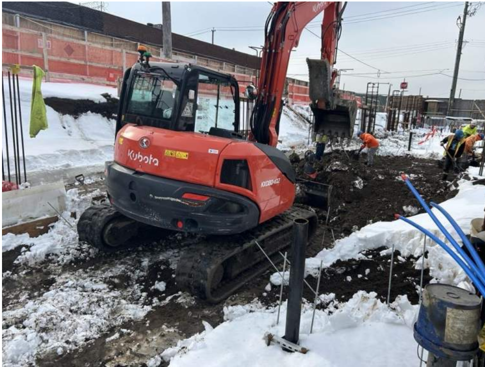
Photo 1: ECD excavating non-hazardous non-native fill in the western part of the site for utility pipe installation (facing west)
