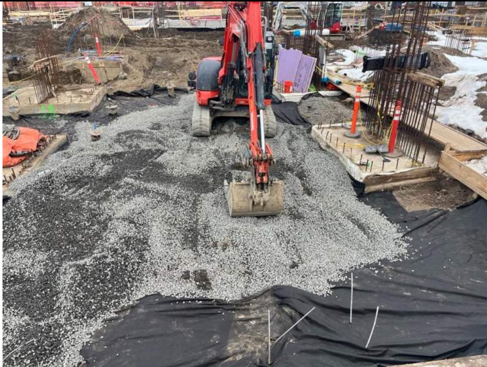
Photo 3: ECD backfilling gas permeable aggregate as part of the SSD system in the western part of the site (facing east)
