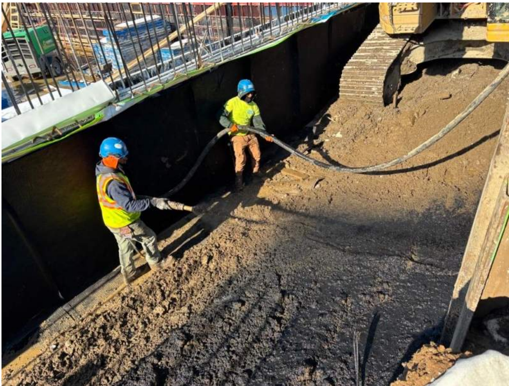
Photo 2: ECD backfilling with previously imported clean fill and PetroFix in the central part of site (facing northeast)
