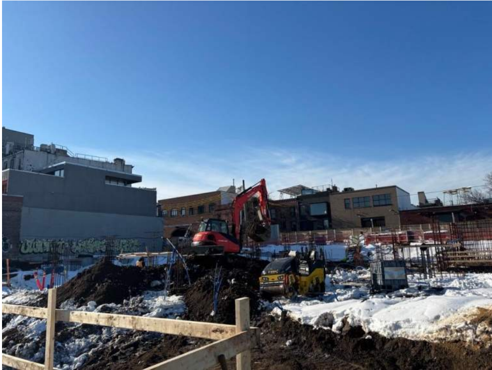
Photo 1: ECD excavating non-hazardous non-native fill in the western part of the site (facing west)
