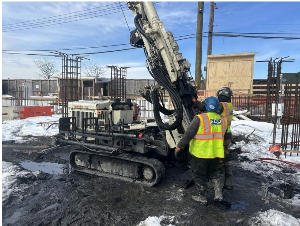
Photo 4: ECD using a Geoprobe 7822DT to inject PetroFix in Treatment Area 1 in the northern part of the site (facing northwest)
