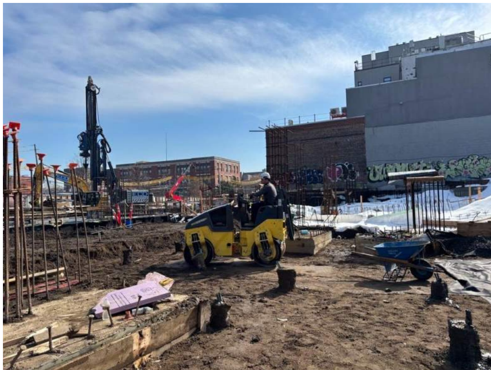
Photo 4: ECD compacting previously backfilled clean fill in the western part of the site (facing southeast)
