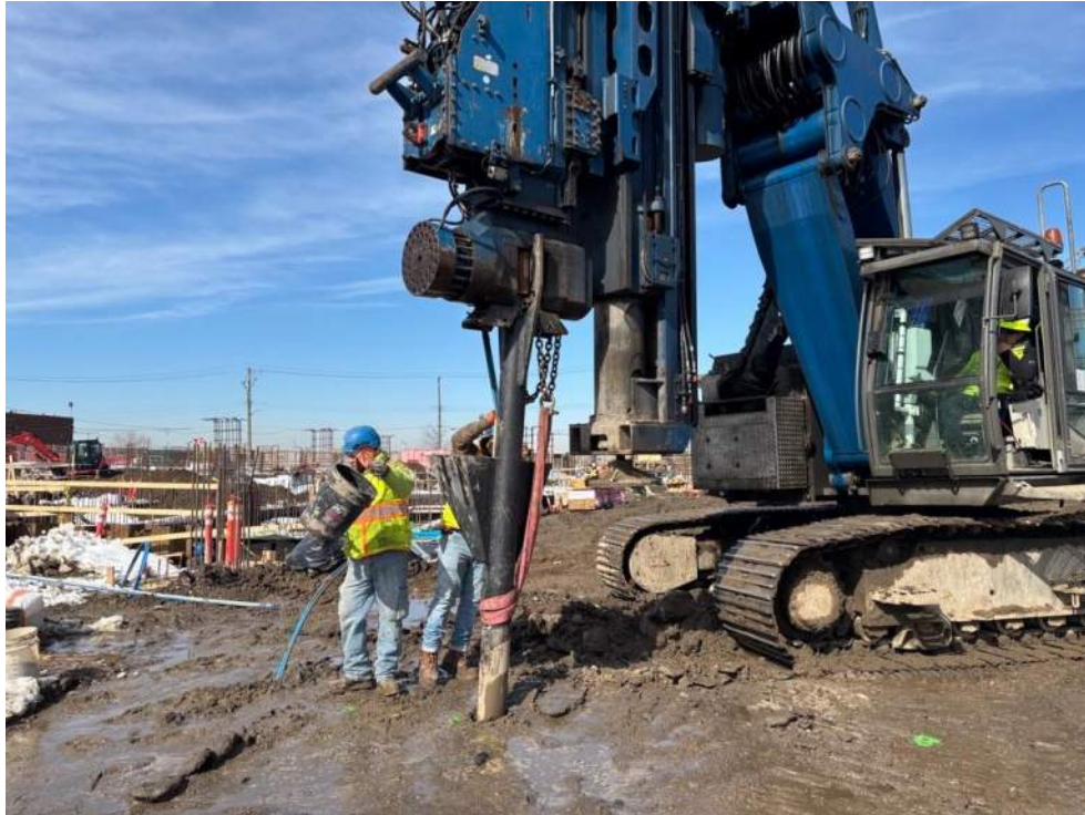
Photo 3: ECD advancing PetroFix injection points in Treatment Area 2 in the eastern part of the site (facing northwest)
