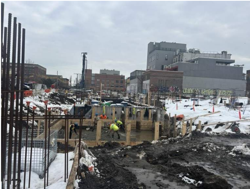
Photo 2: ECD pouring concrete within the crane pad in the central part of site (facing southeast)
