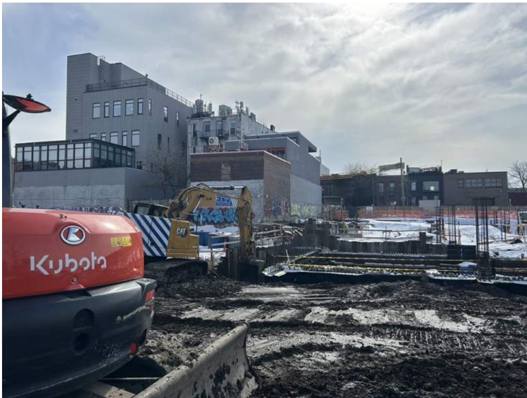
Photo 2: ECD backfilling with previously imported clean fill in the central part of site (facing southwest)
