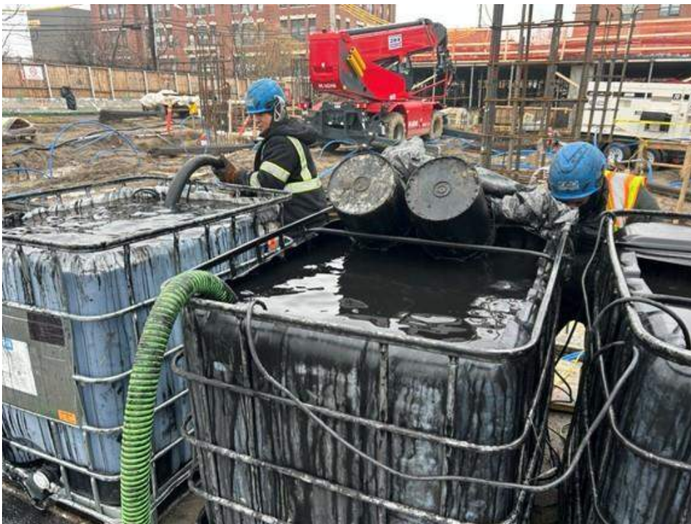
Photo 2: ECD injecting PetroFix in Treatment Area 2 within the central part of the site (facing southeast)
