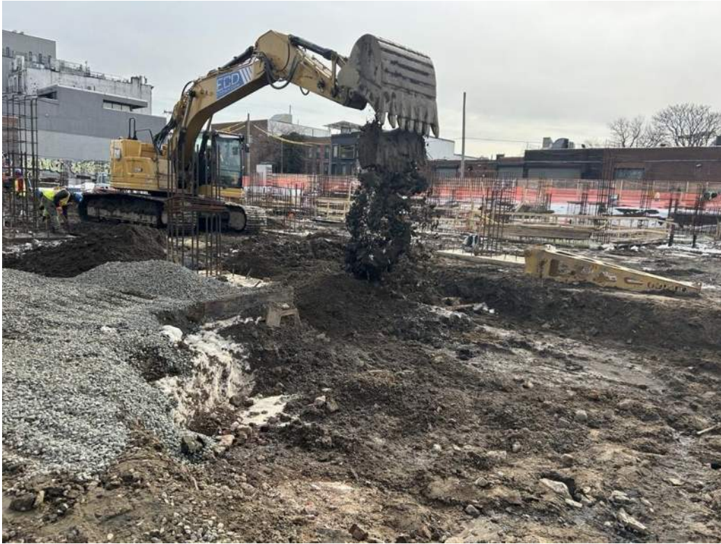
Photo 1: ECD backfilling previously imported clean fill in the northern part of the site (facing southwest)
