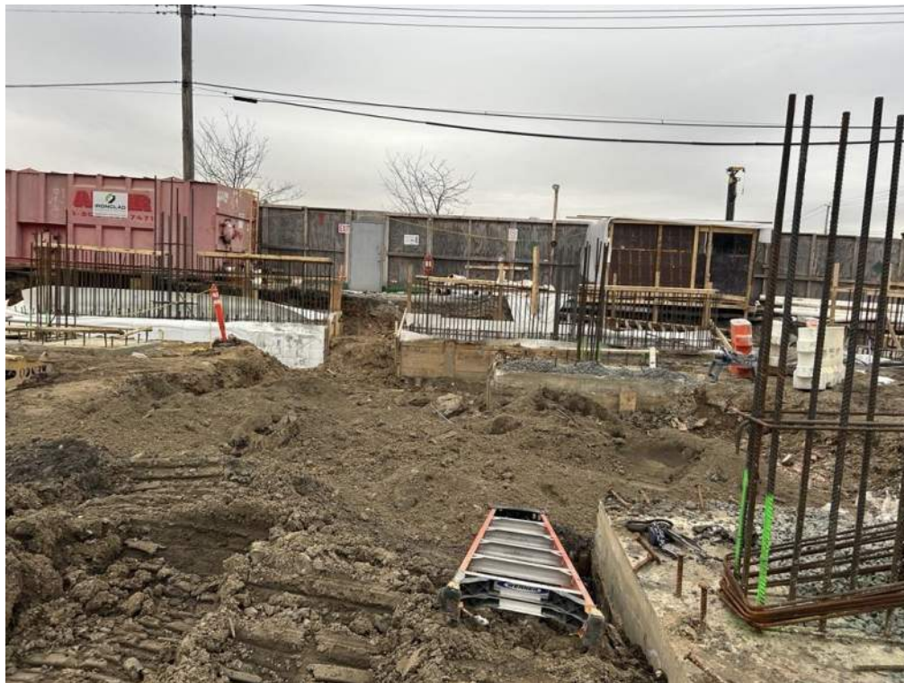
Photo 1: ECD backfilling with previously imported clean fill in the northern part of the site (facing northwest)
