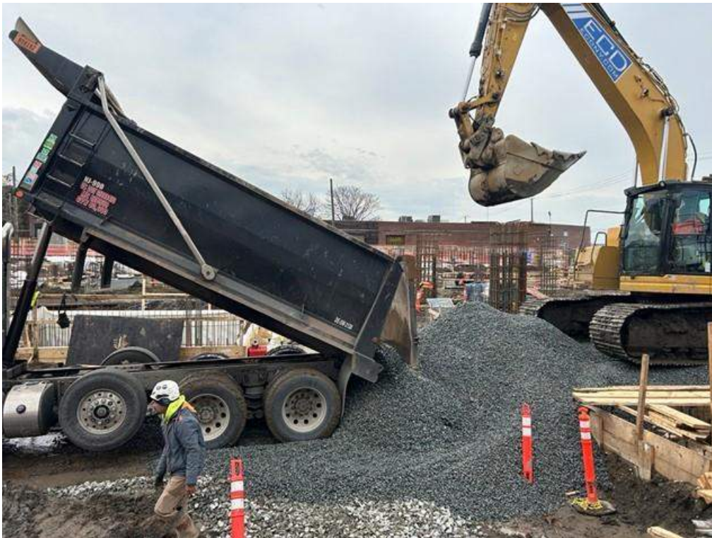
Photo 2: ECD importing ASTM #5 stone in the eastern part of the site (facing west)
