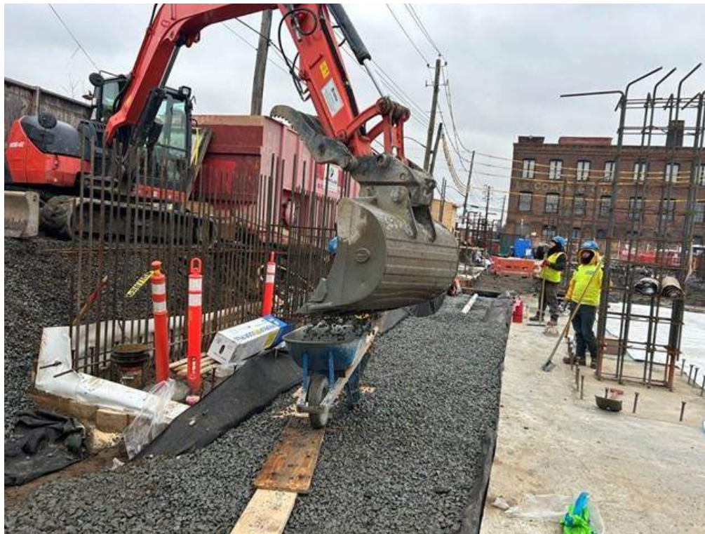
Photo 1: ECD backfilling \frac{3}{4} inch virgin stone atop geotextile fabric as part of the SVE system in the western part of the site (facing north)
