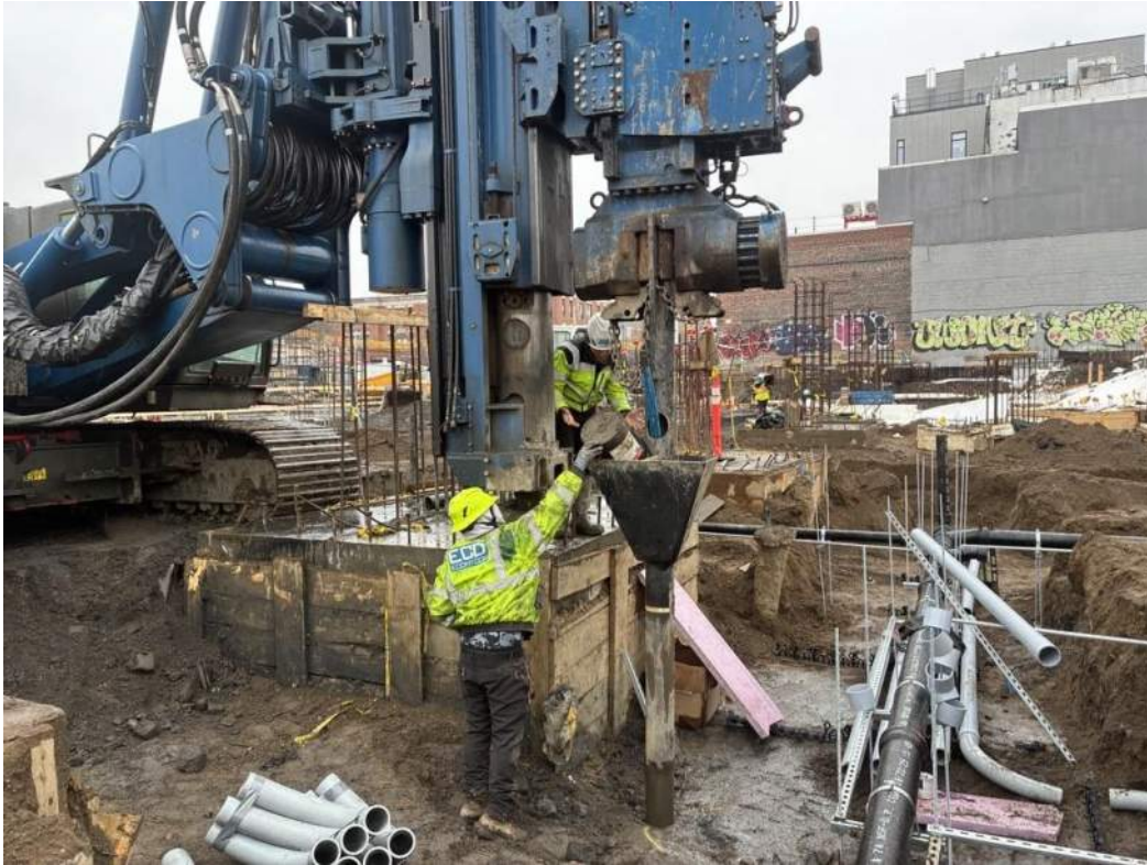
Photo 3: ECD installing injection point 281 in Treatment Area 3 in the western part of the site (facing southeast)
