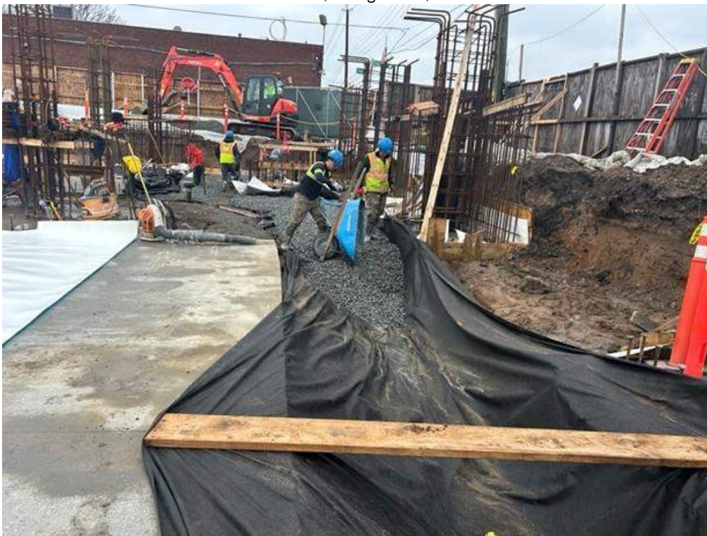
Photo 2: ECD backfilling \frac{3}{4} virgin stone atop geotextile fabric as part of the SVE system in the western part of the site (facing west)
