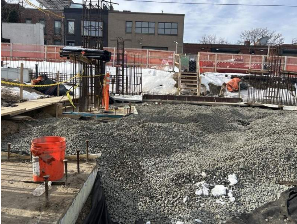
Photo 3: ECD installing the gas permeable aggregate layer as part of the SSD system in the western part of the site (facing southwest)
