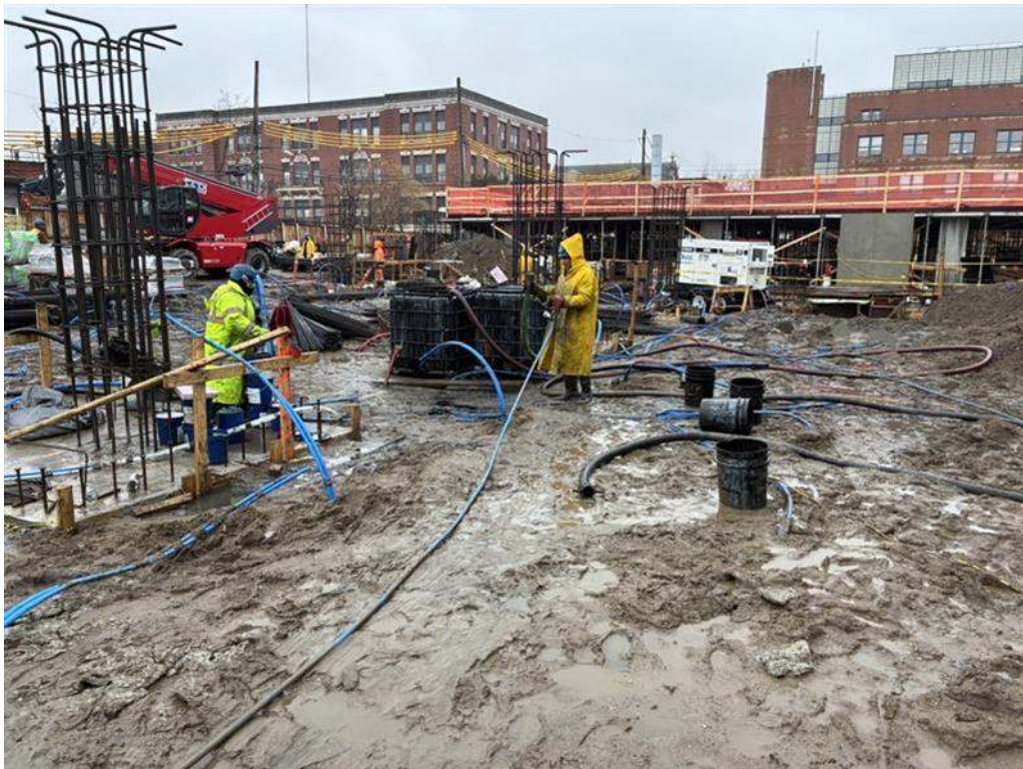
Photo 4: ECD injecting PetroFix in Treatment Area 2 within the central part of the site (facing southeast)
