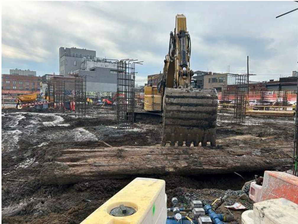
Photo 1: ECD grading previously imported clean fill in the northern part of the site (facing northwest)
