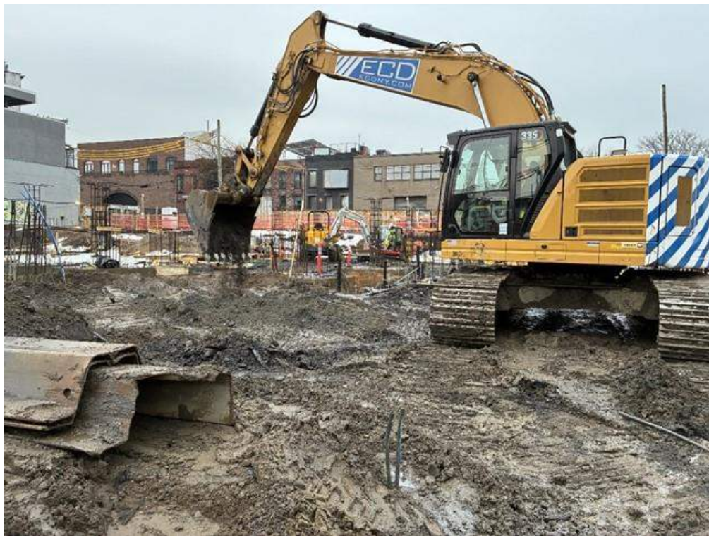
Photo 1: ECD grading previously imported clean fill in the western part of the site (facing southwest)
