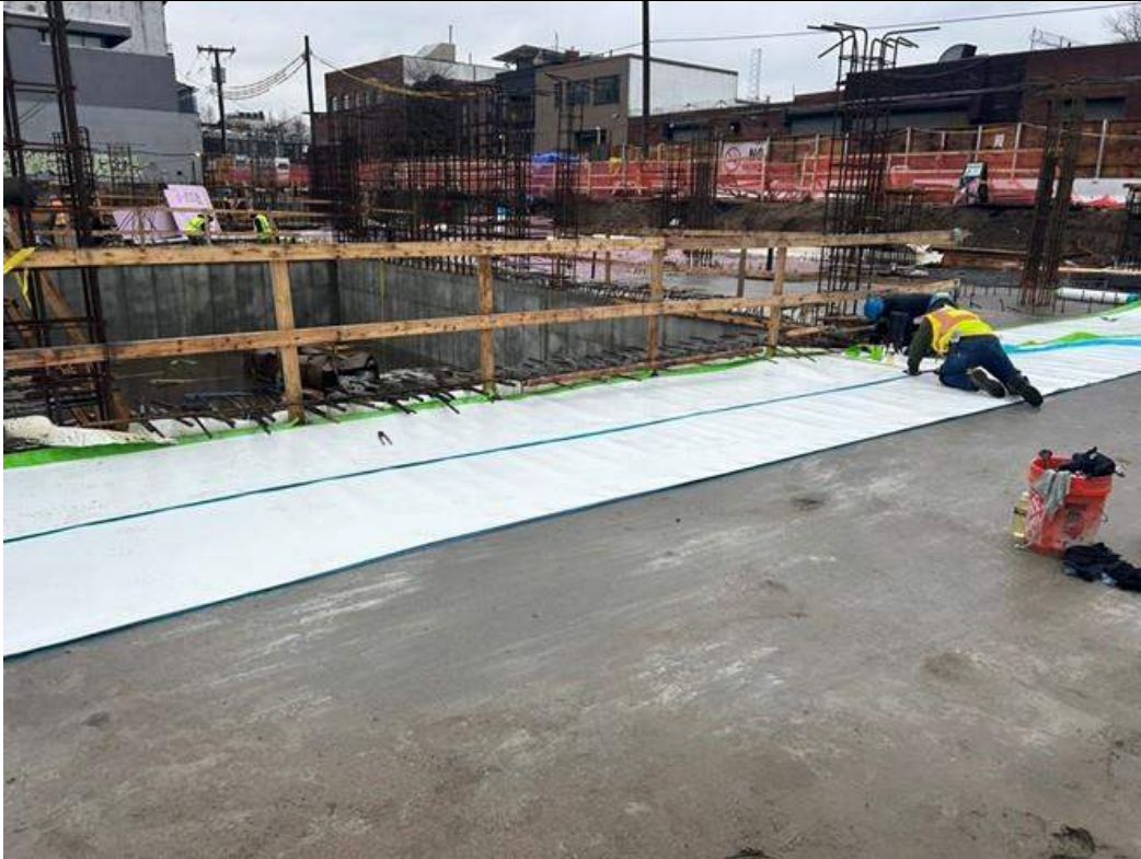
Photo 3: ECD installing Preprufe 300R Plus waterproofing/vapor barrier membrane atop rat slab in the western part of the site (facing southwest)
