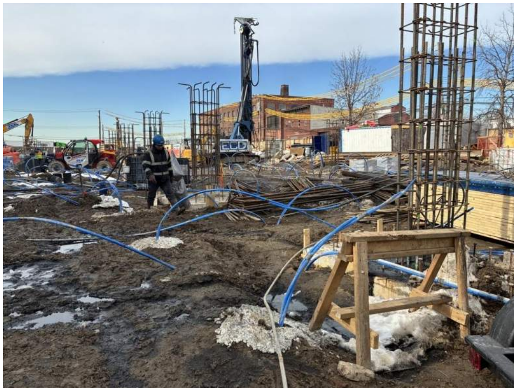
Photo 4: ECD injecting PetroFix in Treatment Area 2 in the central part of the site (facing north)
