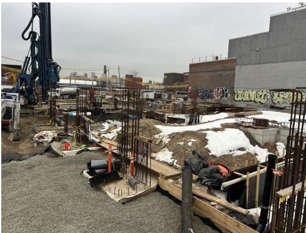
Photo 2: ECD excavating for the installation of utility piping in the western part of the site (facing east)
