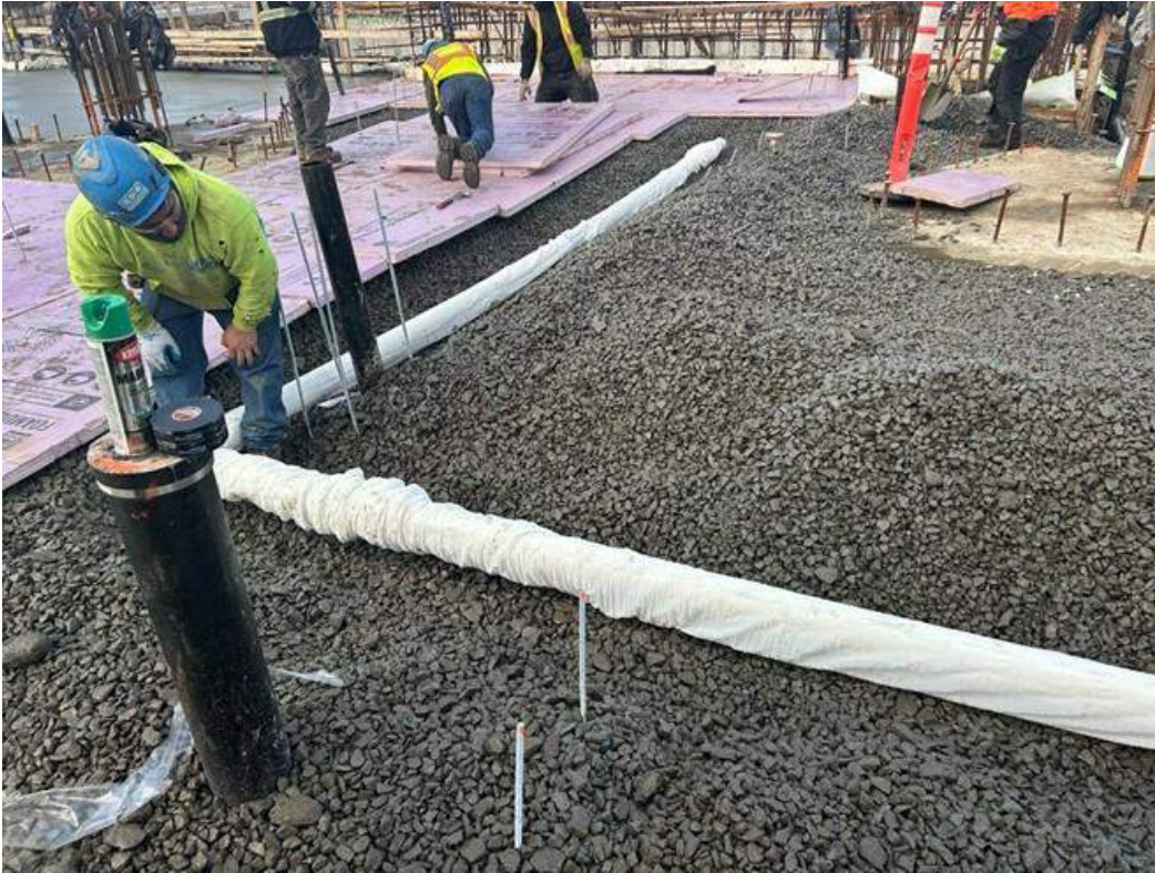
Photo 3: ECD installing the SSD system in the western part of the site (facing north)
