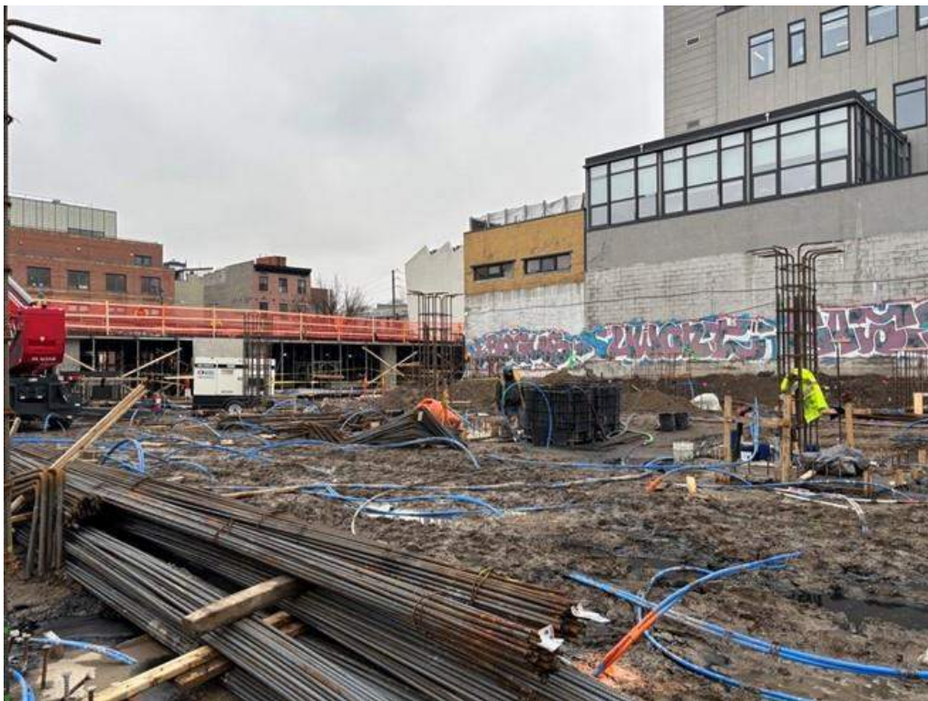
Photo 4: ECD injecting PetroFix in Treatment Area 2 within the central part of the site (facing south)
