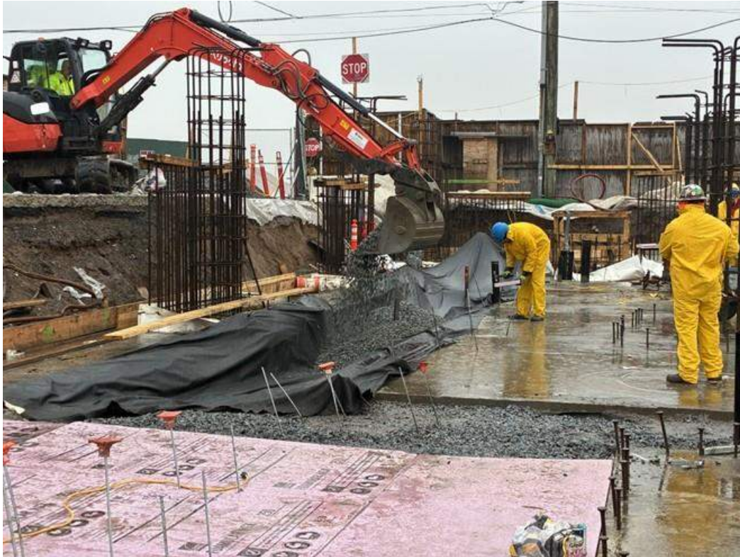
Photo 3: ECD backfilling clean imported \frac{3}{4} virgin stone atop geotextile fabric as part of the SVE system in the western part of the site (facing northwest)
