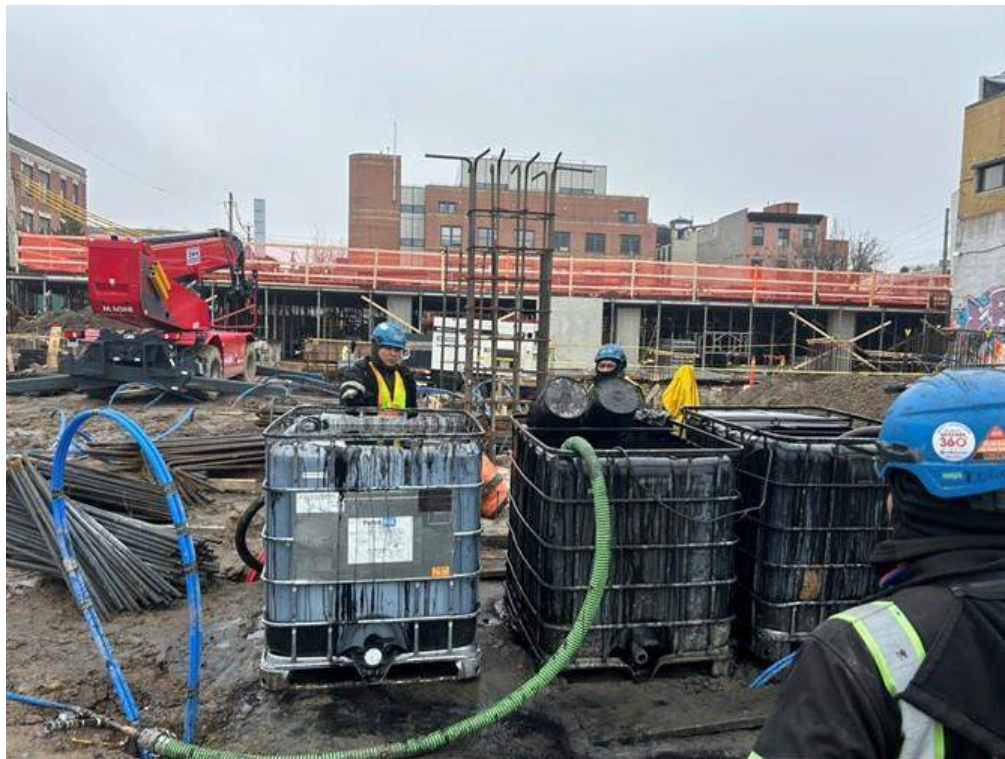
Photo 1: ECD injecting PetroFix in Treatment Area 2 within the central part of the site (facing south)
