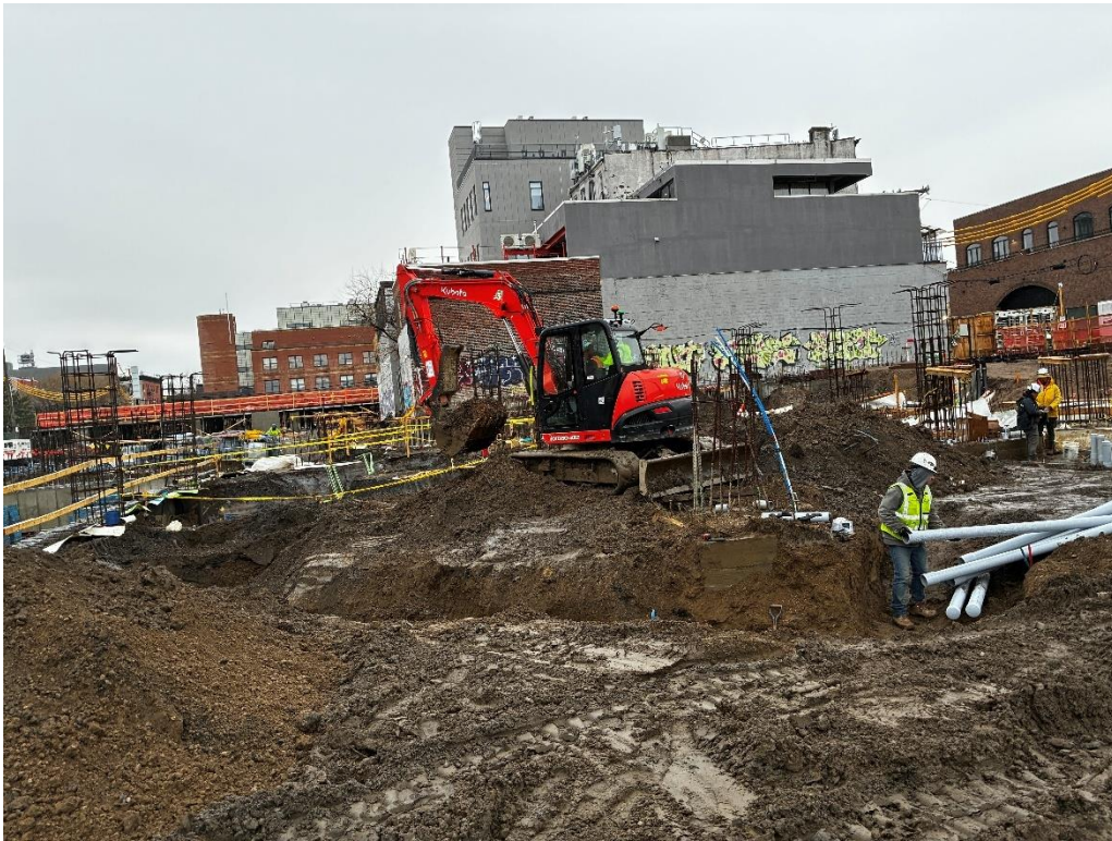
Photo 1: ECD excavating within non-native fill for utility trenches in the central part of the site (facing south)
