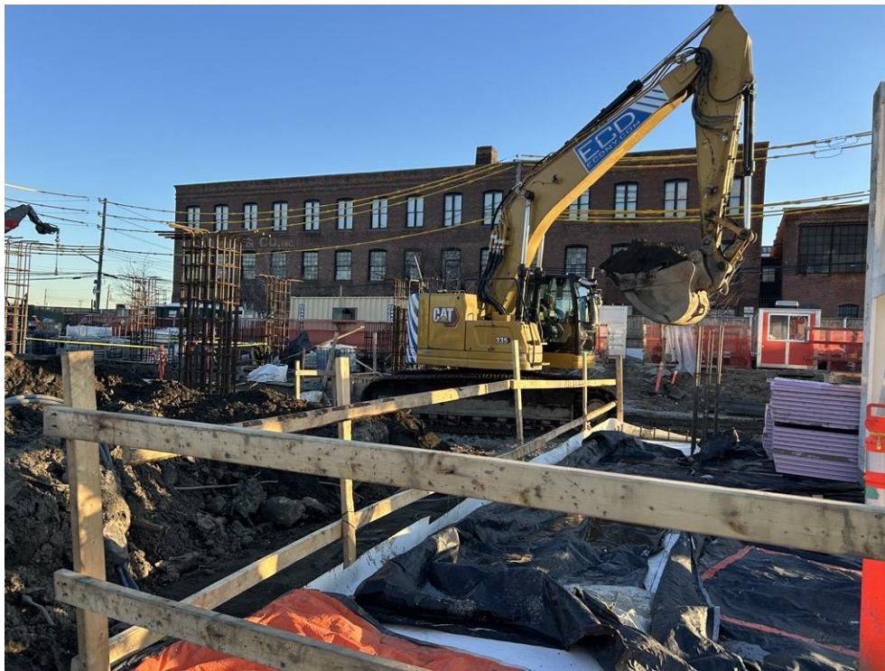
Photo 4: ECD backfilling with previously imported clean fill in the central part of the site (facing east)
