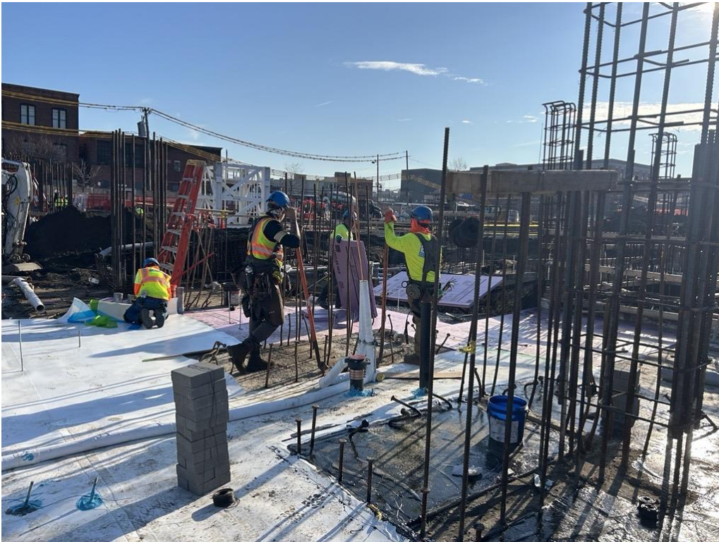
Photo 1: ECD installing Preprufe 300R Plus waterproofing/vapor barrier membrane atop rat slab in the western part of the site (facing east)
