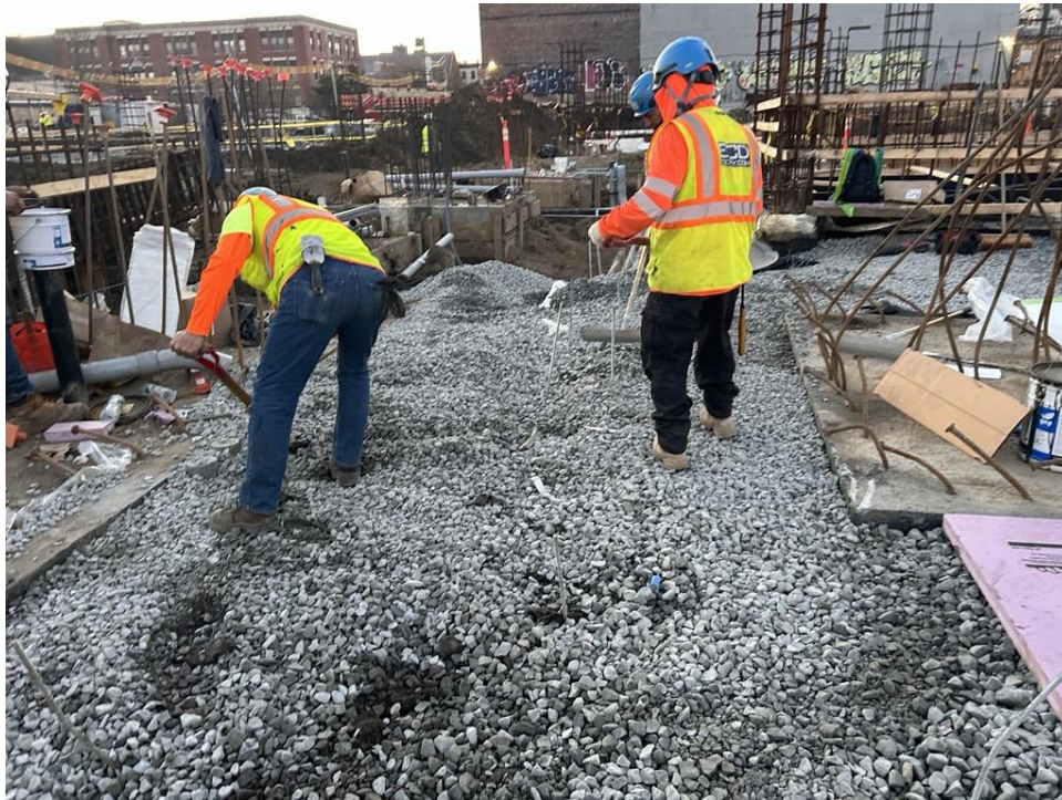
Photo 2: ECD backfilling with previously imported stone atop the SSDS in the western part of the site (facing southeast)
