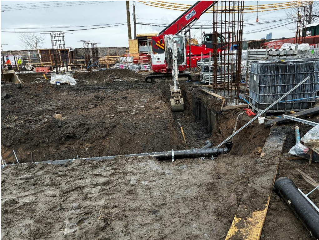
Photo 2: ECD excavating within non-native fill for utility trenches in the northern part of the site (facing northwest)
