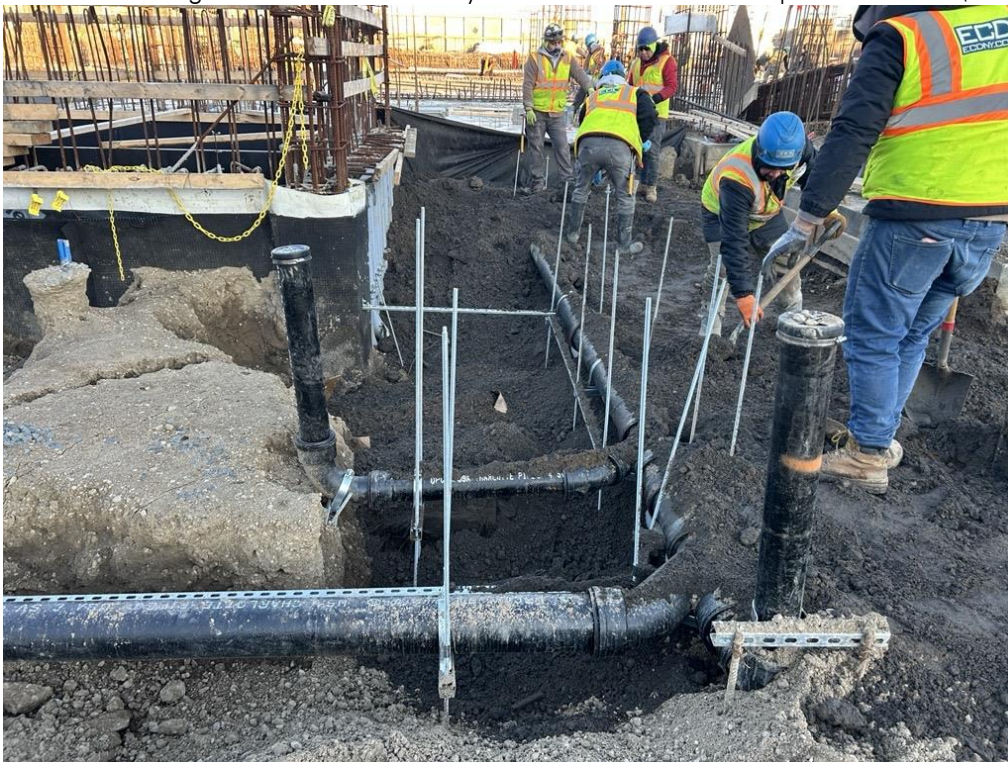
Photo 2: ECD backfilling utility trenches with previously imported clean fill in the western part of the site (facing northwest)
