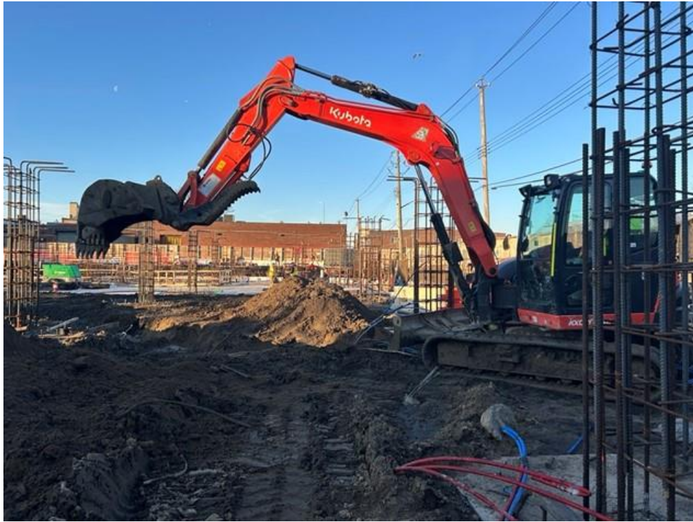
Photo 3: ECD excavating for the installation of utility piping in the western part of the site (facing north)
