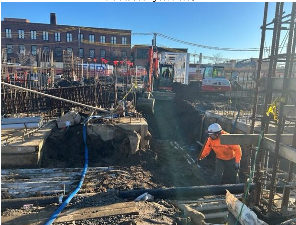
Photo 2: ECD backfilling utility trench excavations in the western part of the site with previously imported clean fill (facing east)
