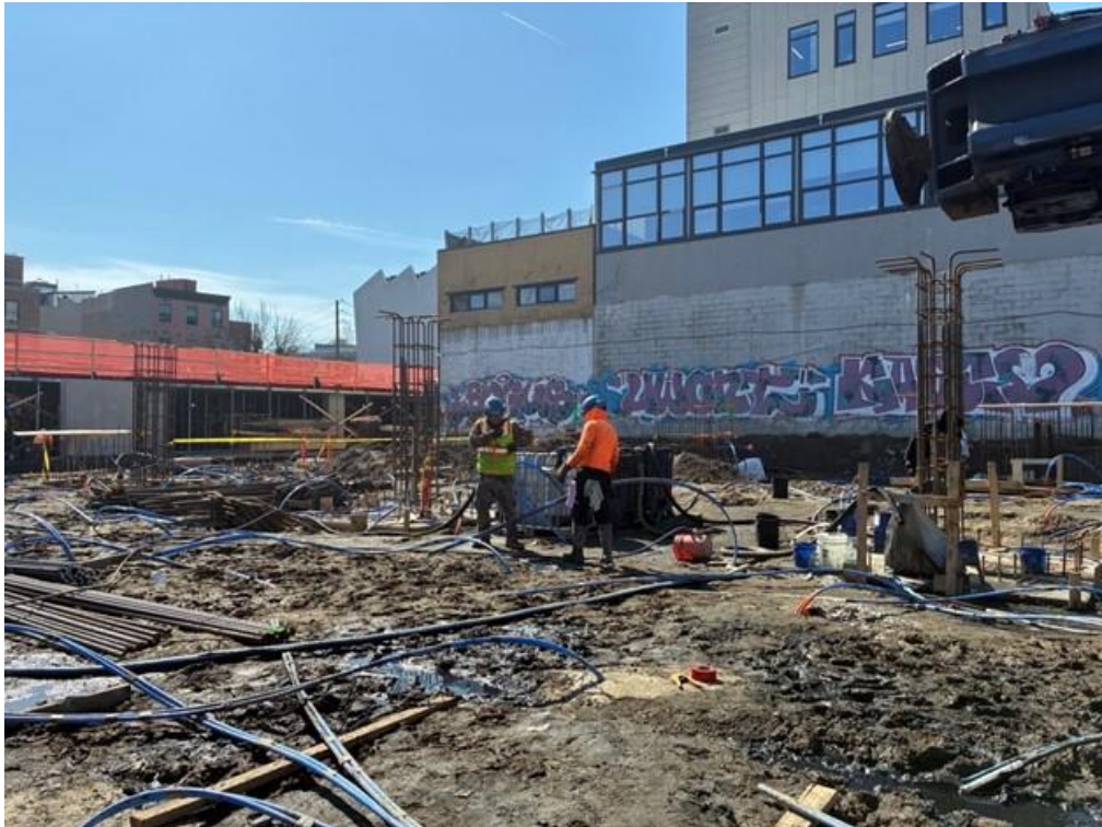
Photo 4: ECD injecting PetroFix in Treatment Area 2 within the central part of the site (facing northwest)
