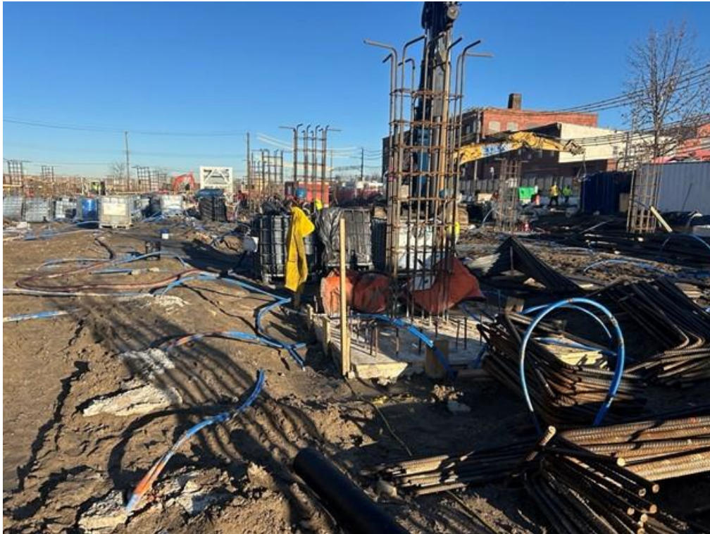
Photo 4: ECD injecting PetroFix in Treatment Area 2 within the central part of the site (facing northwest)
