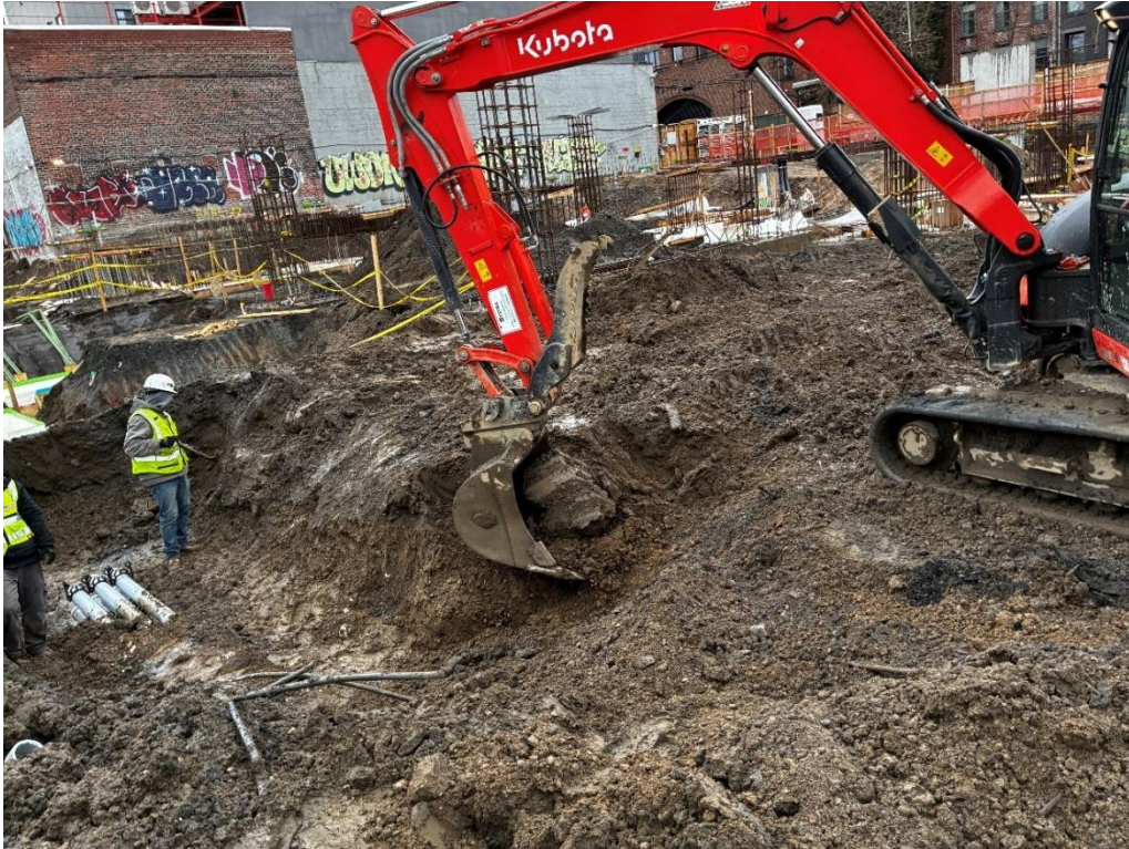
Photo 3: ECD backfilling utility trenches with previously imported clean fill in the central part of the site (facing south)
