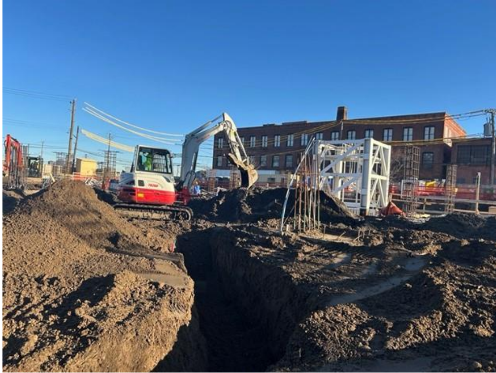
Photo 3: ECD excavating for the installation of utility piping in the western part of the site (facing north)
