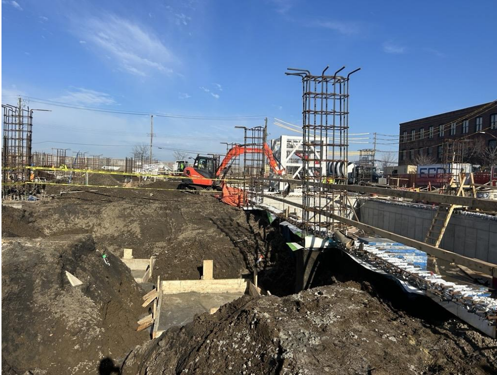
Photo 3: ECD backfilling with previously imported clean fill in the central part of the site (facing northwest)
