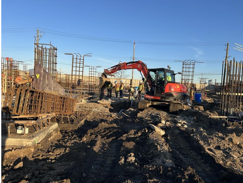
Photo 3: ECD backfilling with previously imported ¾-inch stone in the western part of the site (facing west)
