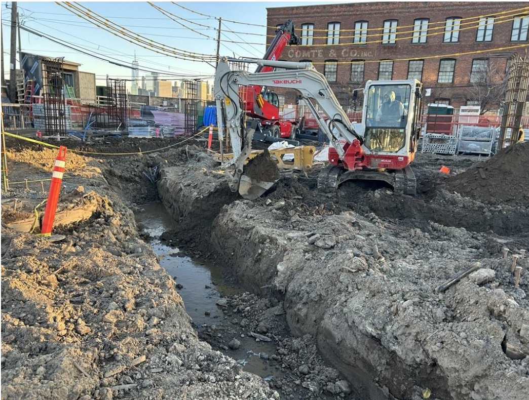
Photo 1: ECD excavating non-native fill for utility trenches in the northern part of the site (facing north)
