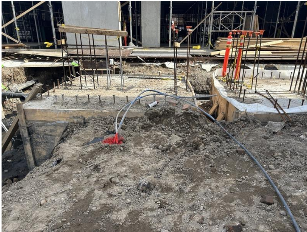
Photo 1: ECD injecting PetroFix within Treatment Area 2 in the central part of the site (facing east)
