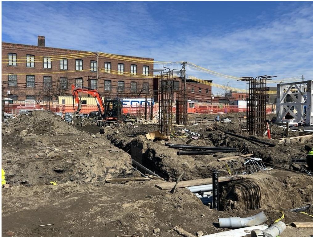
Photo 4: ECD backfilling a utility pipe trench with previously imported clean fill in the northern part of the site (facing east)
