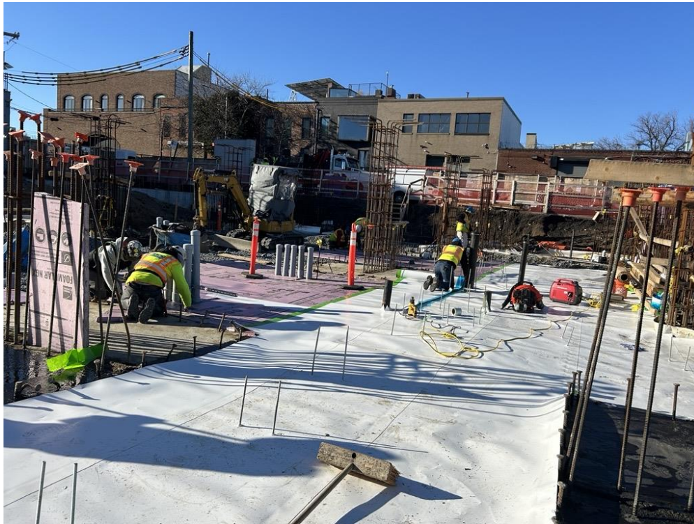
Photo 1: ECD laying Preprufe 300R Plus waterproofing vapor barrier membrane atop a rat slab in the western side of the site (facing southwest)
