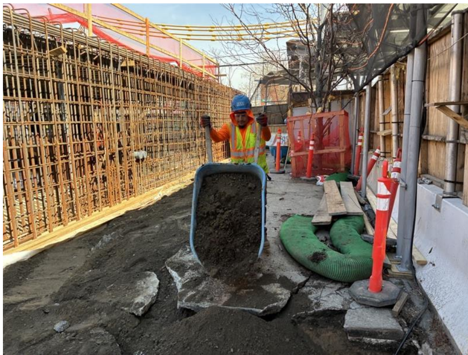
Photo 2: ECD backfilling utility trenches in the eastern part of the site (facing northeast)
