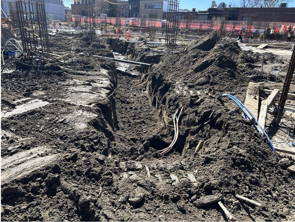
Photo 3: ECD excavating for the installation of utility piping in the northern part of the site (facing southwest)
