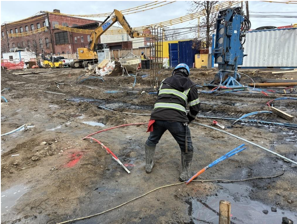
Photo 4: ECD injecting PetroFix within Treatment Area 2 in the central part of the site (facing northeast)
