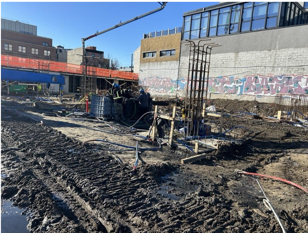
Photo 4: ECD injecting PetroFix within Treatment Area 2 in the central part of the site (facing southwest)
