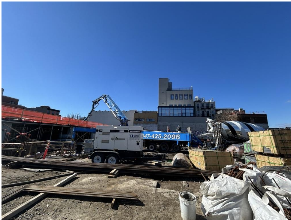
Photo 2: ECD pouring concrete within the building's foundation in the southern part of the site (facing west)
