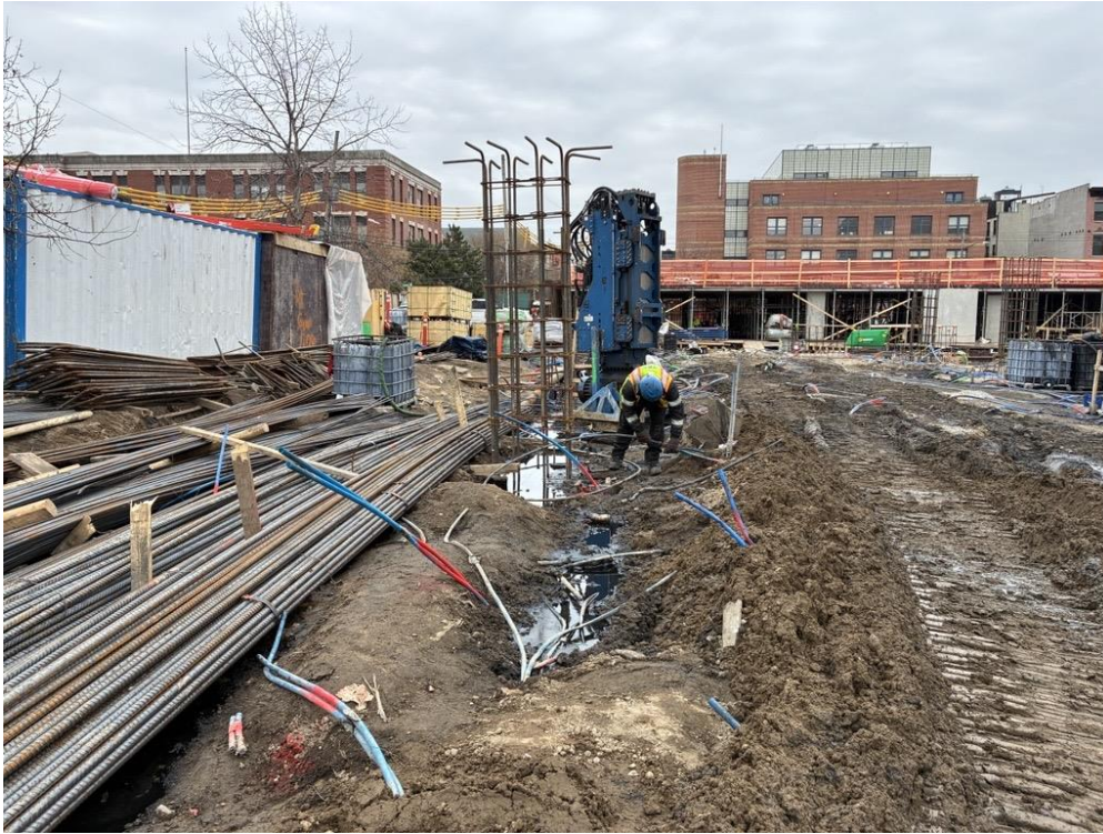
Photo 1: ECD injecting PetroFix within Treatment Area 2 in the central part of the site (facing east)
