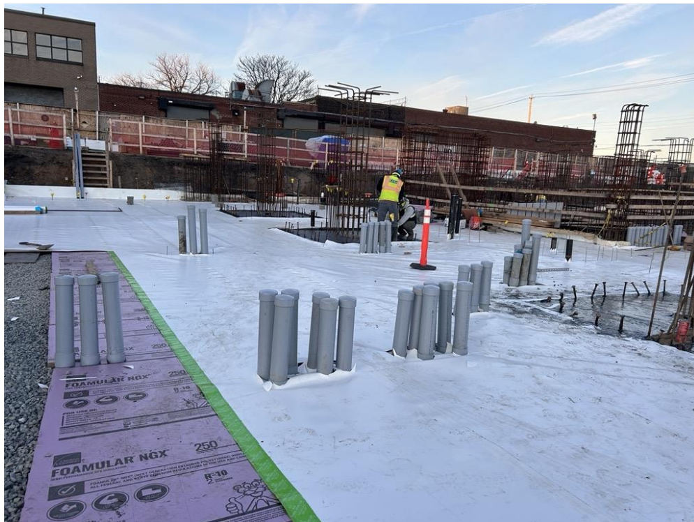
Photo 1: ECD installing Preprufe 300R Plus waterproofing vapor barrier membrane atop a rat slab in the western part of the site (facing west)
