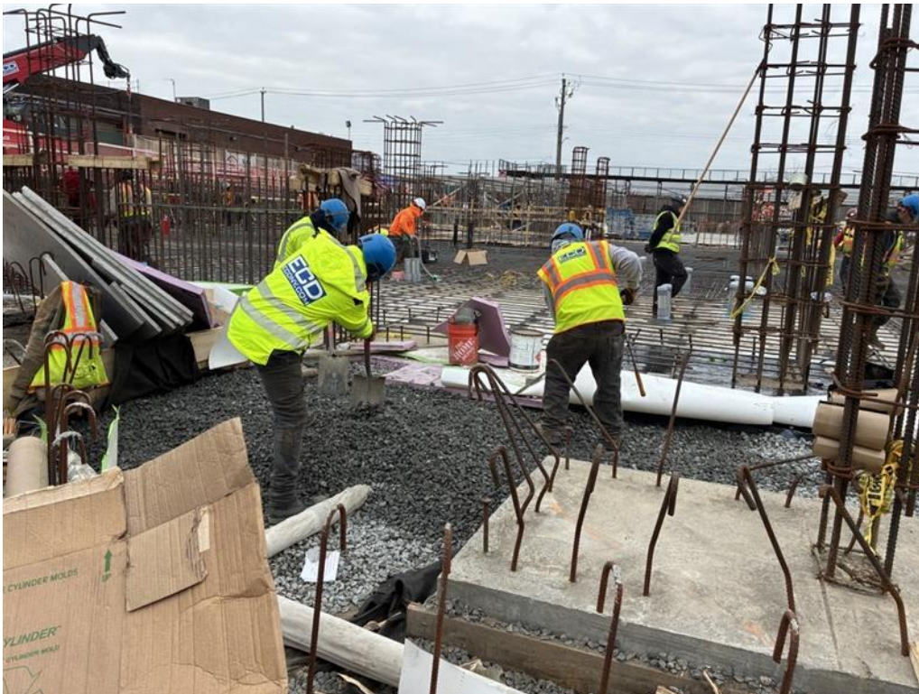
Photo 4: ECD backfilling ASTM #5 stone atop SSDS piping in the southern part of site (facing west).
