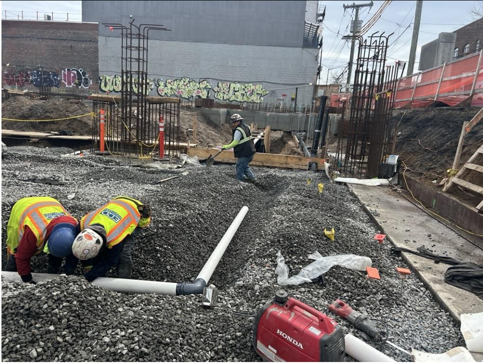
Photo 3: ECD installing PVC piping for the installation of the SSDS in the western part of the site (facing south)
