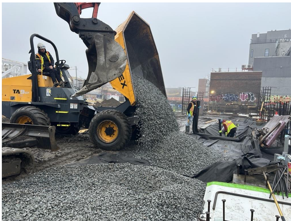
Photo 2: ECD backfilling with previously imported ¾-inch stone in the western part of the site for SSDS installation (facing southeast)
