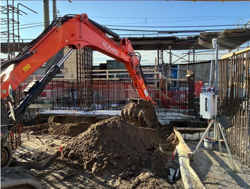
Photo 3: ECD excavating within clean fill for utility piping in the northwestern part of the site (facing northwest)
