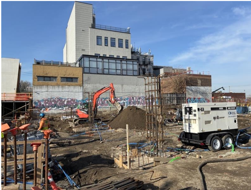
Photo 4: ECD stockpiling clean fill collected from grading in the southern part of site (facing south).
