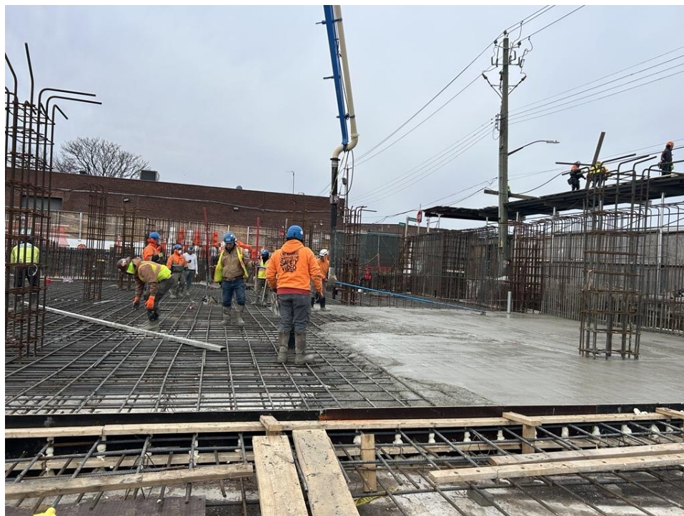
Photo 2: ECD pouring concrete for the site cover in the western part of the site (facing southwest)
