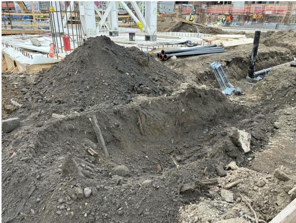
Photo 2: ECD excavating within clean fill for utility piping in the western part of the site (facing southeast)
