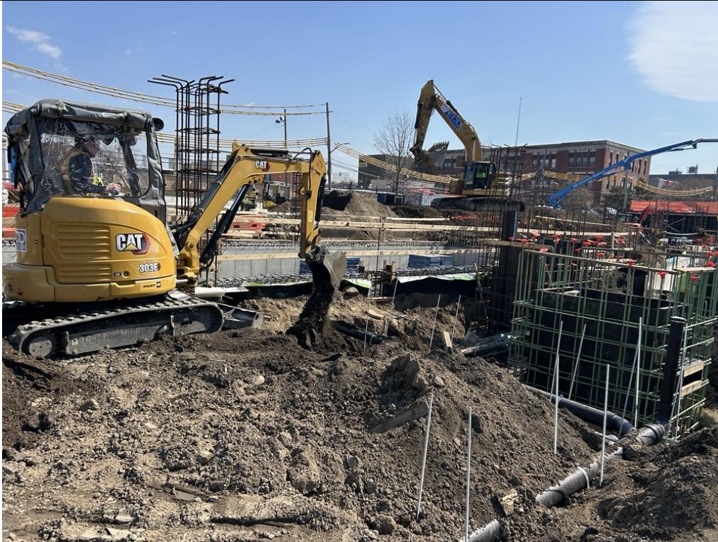
Photo 3: ECD backfilling with previously imported clean fill to surface grade around the detention tank in the central part of the site (facing east)
