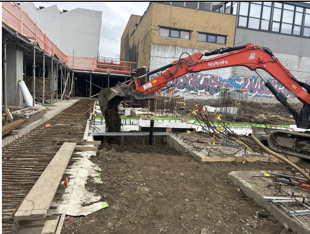
Photo 3: ECD backfilling with previously imported clean fill to surface grade around utility piping in the southern part of the site (facing southwest)
