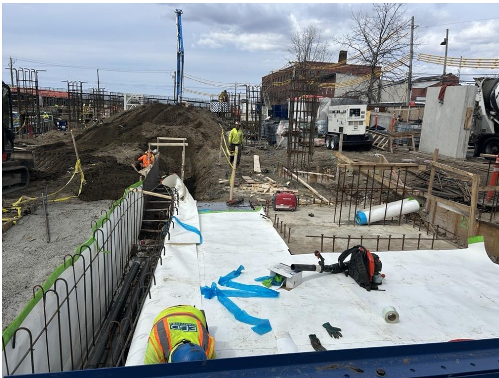
Photo 4: ECD installing Preprufe 300R Plus waterproofing / vapor barrier atop rat slab in the southern part of the site (facing north)
