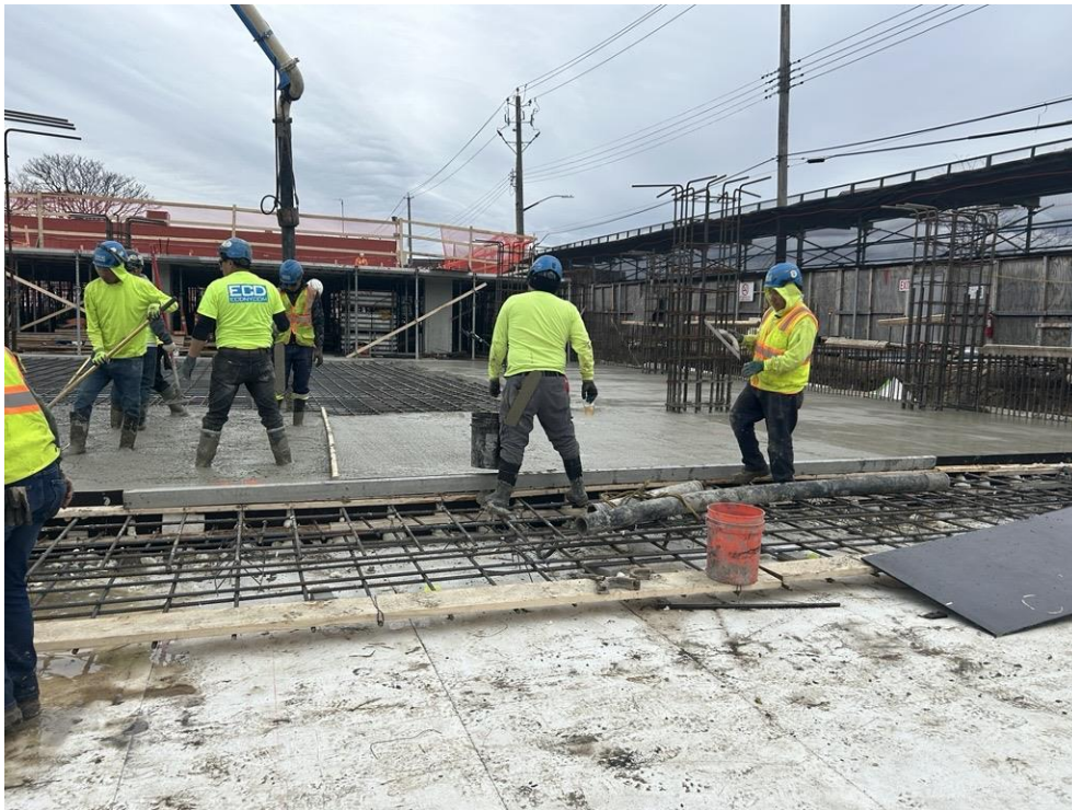
Photo 2: ECD pouring a 12-inch-thick concrete slab in the northern part of the site (facing west)
