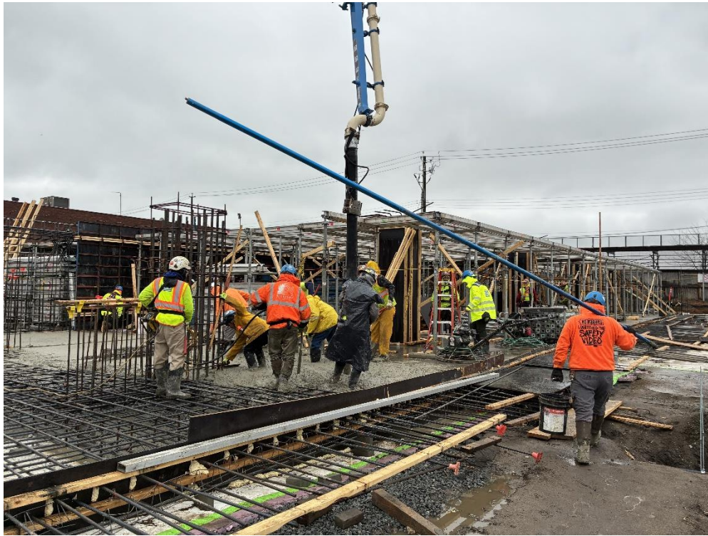
Photo 1: ECD pouring an about 8-inch-thick concrete slab in the northeastern part of the site (facing east)
