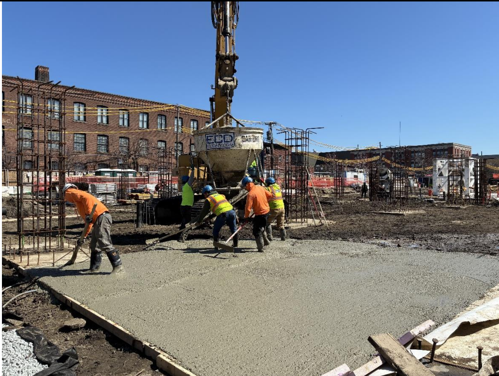
Photo 3: ECD pouring an about 3-inch-thick concrete rat slab in the northwestern part of the site (facing east)
