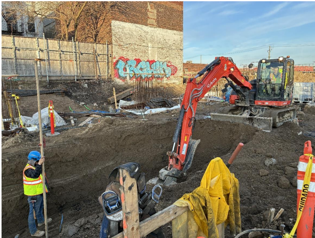
Photo 4: ECD excavating within clean fill for utility piping installation in the southern part of the site (facing west)
