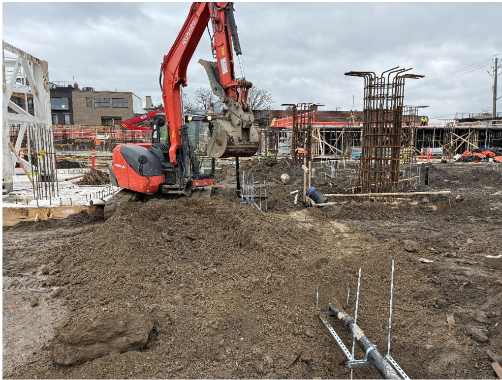
Photo 4: ECD backfilling clean fill to working grade in the northern part of site (facing east).
