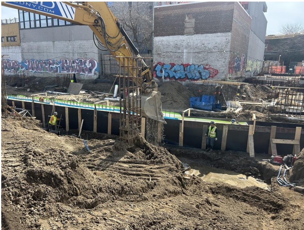
Photo 4: ECD backfilling an about 6-inch-thick layer of previously imported ¾-inch stone for utility piping installation (facing west)
