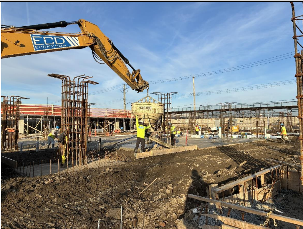
Photo 3: ECD pouring an about 3-inch-thick concrete rat slab in the northern part of the site (facing west)
