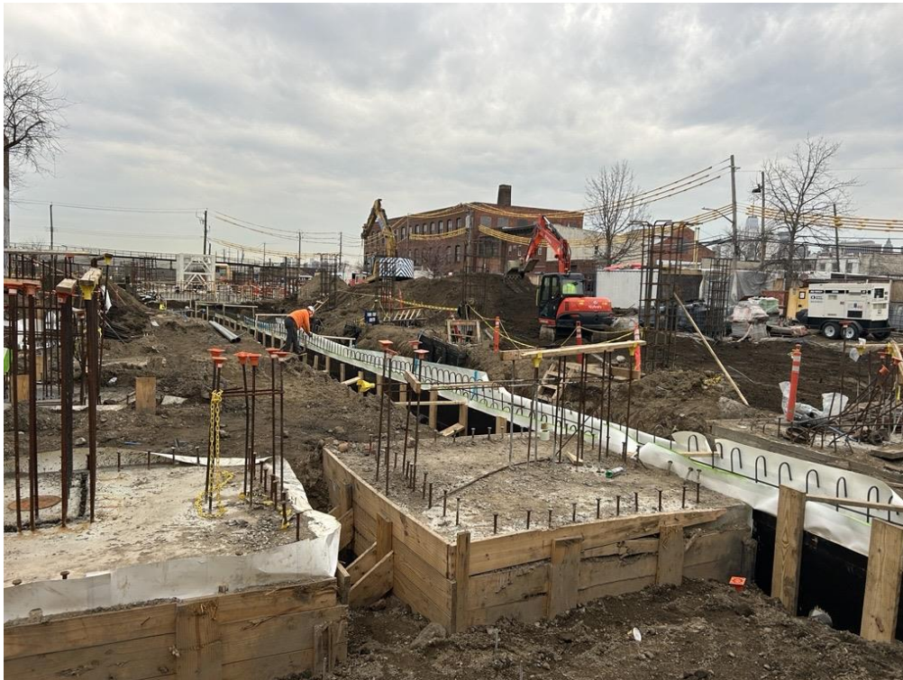
Photo 1: ECD adding previously imported clean fill to the stockpile in the central part of the site (facing northeast)
