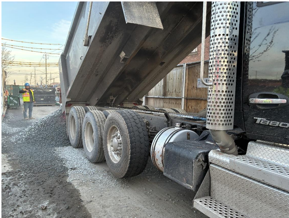
Photo 1: ECD importing ASTM #5 stone in the northeastern part of the site (facing north)
