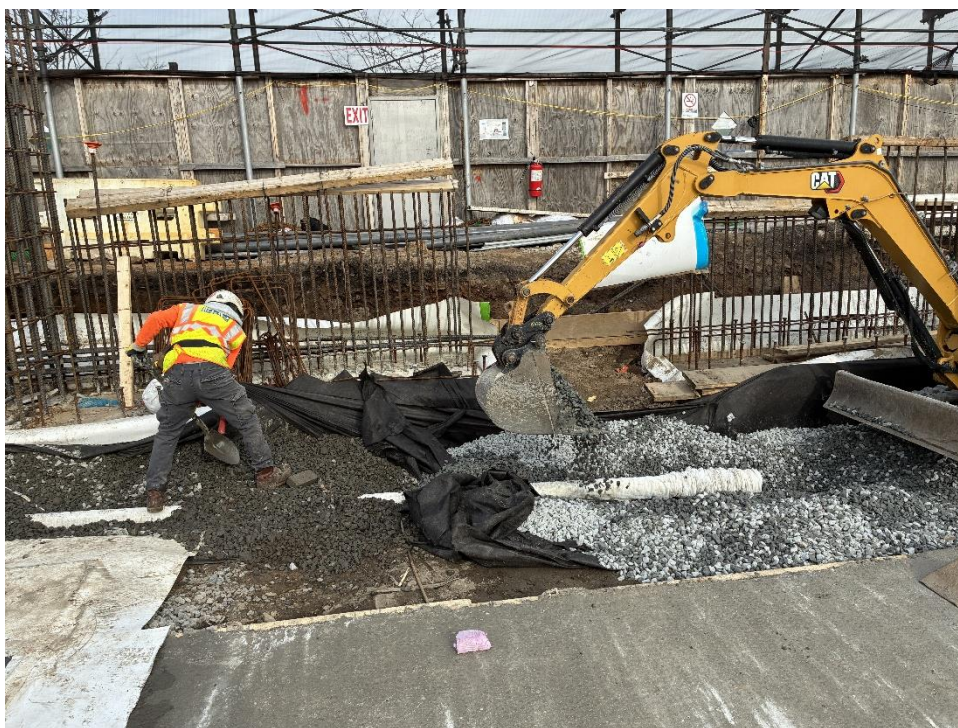
Photo 2: ECD backfilling \frac{3}{4} -inch virgin stone (ASTM No. 5) as part of the SVE system in the northern part of the site (facing north)
