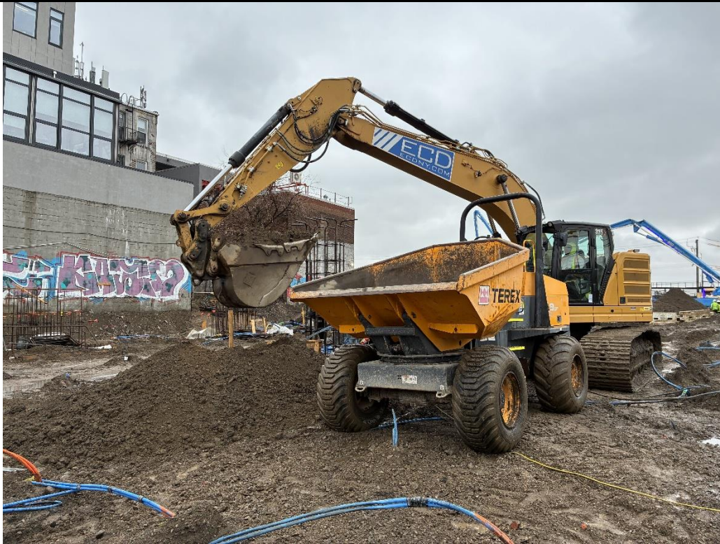
Photo 3: ECD relocating clean fill in the southern part of the site (facing east)
