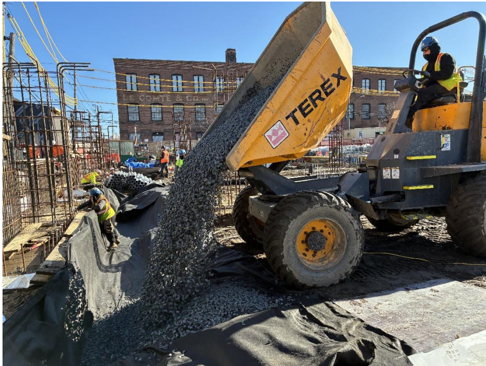
Photo 2: ECD backfilling \frac{3}{4} -inch virgin stone (ASTM No. 5) as part of the SVE system in the northern part of the site (facing northwest)
