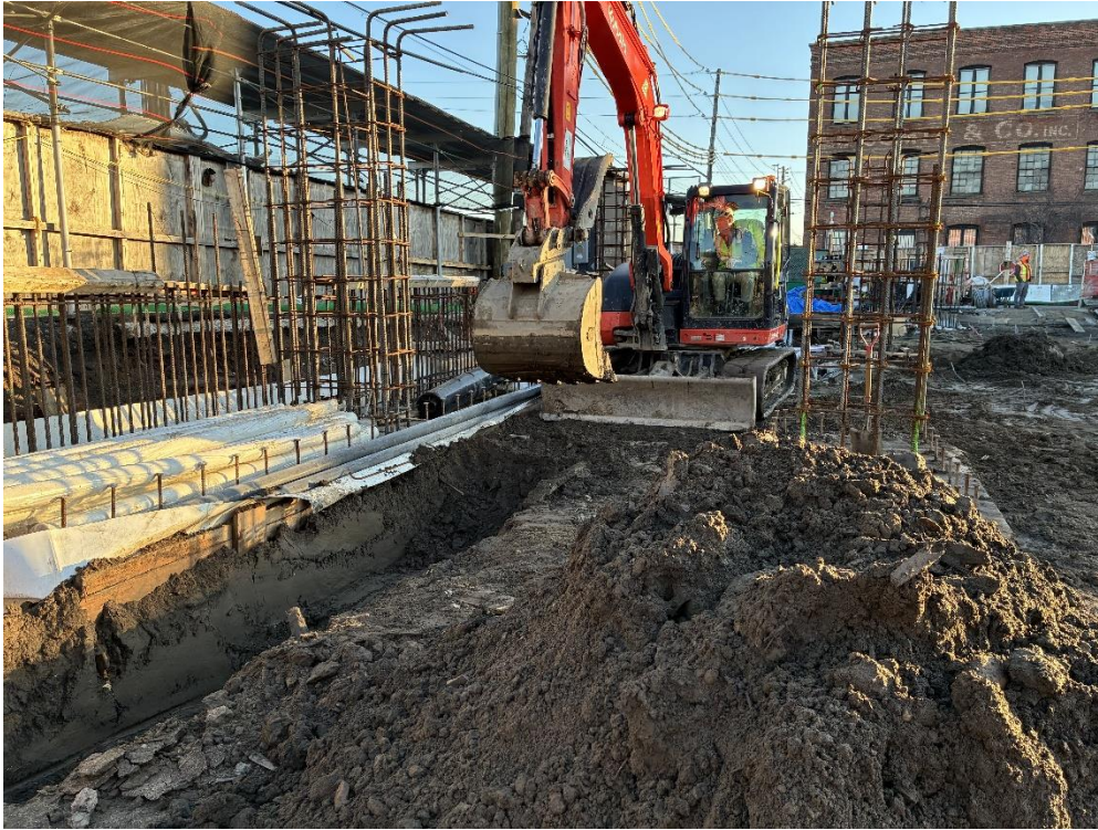
Photo 1: ECD excavating within non-native fill for installation of SVE system components in the northern part of the site (facing north)
