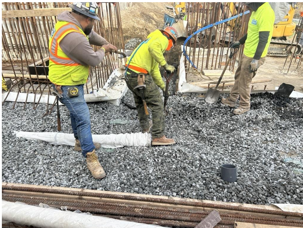
Photo 4: ECD backfilling with \frac{3}{4} -inch virgin stone (gas permeable aggregate) as part of the SSDS in the southern part of the site (facing northwest)
