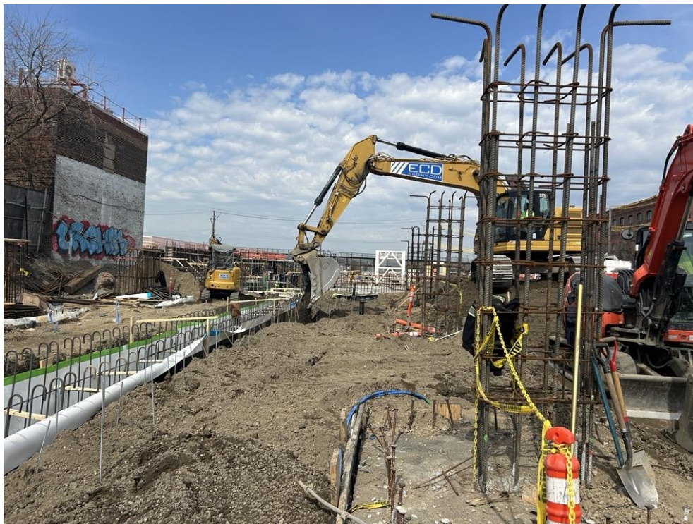
Photo 4: ECD backfilling with previously imported clean fill atop utility piping in the central part of the site (facing northwest)
