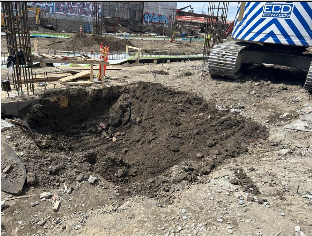
Photo 3: ECD excavating non-native fill beneath the base of the former steel tank in the southeastern part of the site (facing west)
