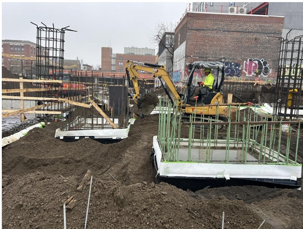
Photo 1: ECD backfilling with previously imported clean fill to surface grade around ConEd utility boxes in the western part of the site (facing north)
