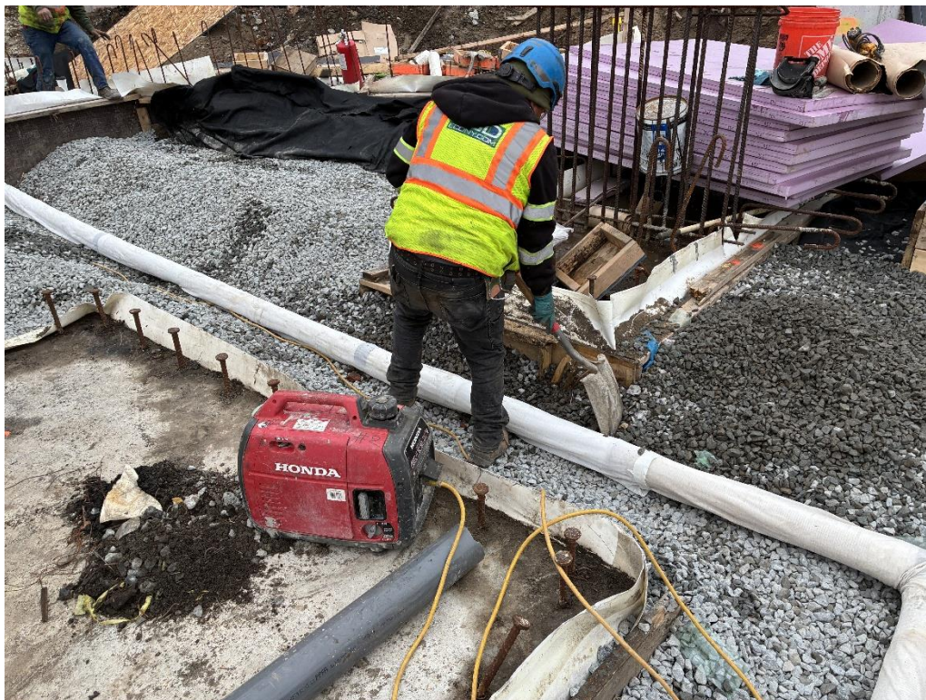
Photo 2: ECD installing the SSDS in the western part of the site (facing west)
