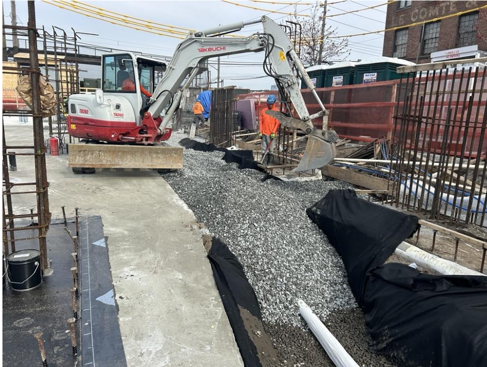
Photo 3: ECD backfilling with \frac{3}{4} -inch virgin stone (gas permeable aggregate) as part of the SVE system in the northern part of the site (facing north)
