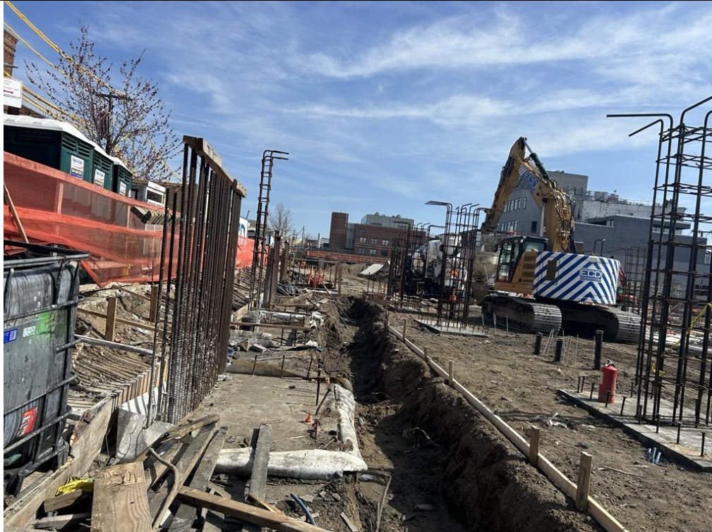
Photo 3: ECD excavating previously imported clean fill for SVE installation in the northern part of the site (facing southeast)
