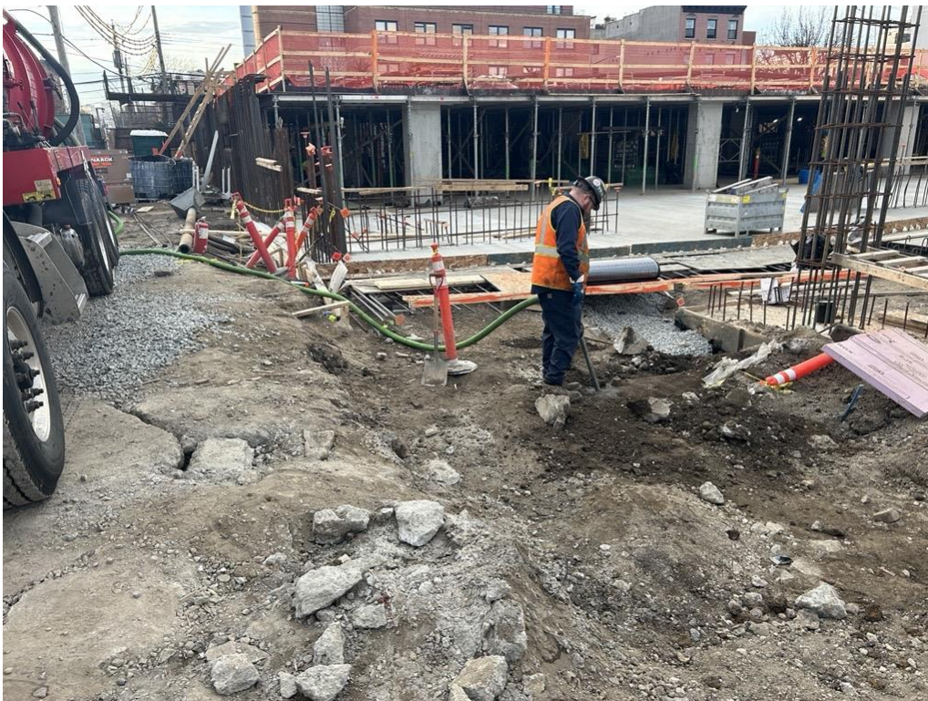
Photo 2: Arcwood extracting the contents of the steel tank for off-site disposal (facing south)
