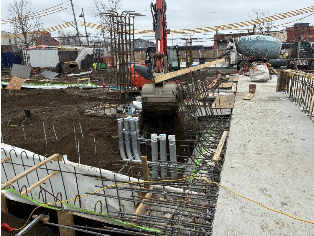
Photo 3: ECD backfilling a utility pipe trench with previously imported clean fill in the southern part of the site (facing east)
