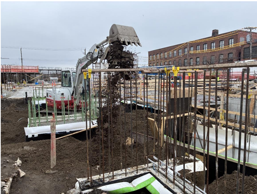
Photo 1: ECD backfilling with previously imported clean fill to surface grade around ConEd utility boxes in the western part of the site (facing north)
