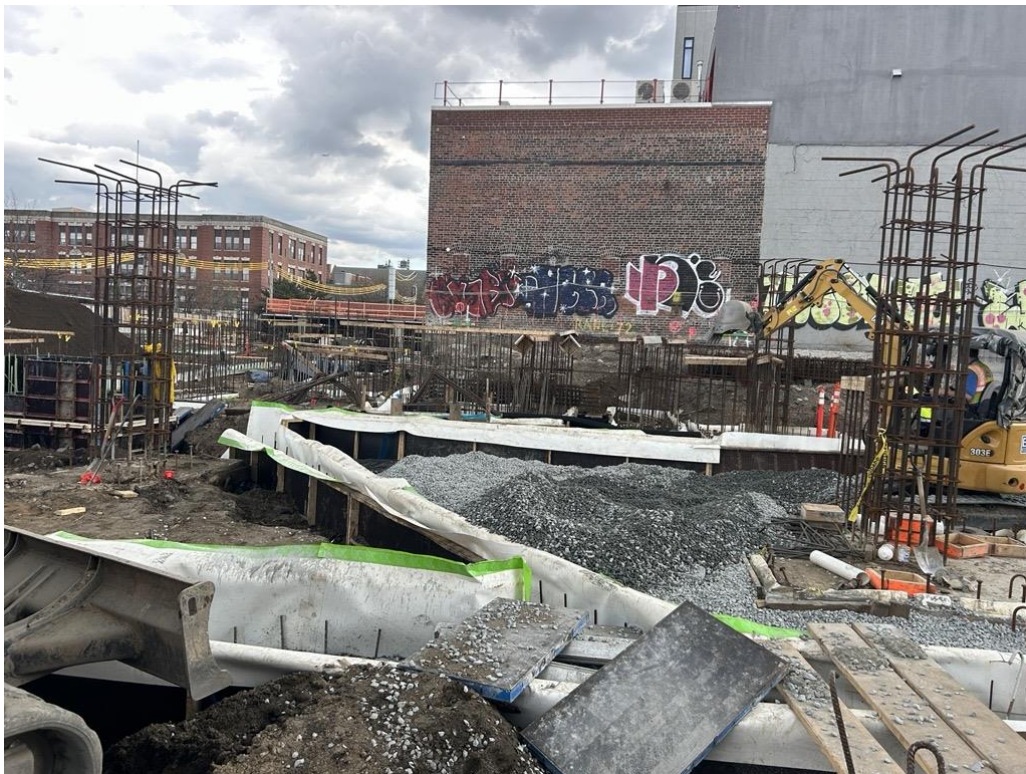
Photo 4: ECD backfilling SVE piping with previously imported ¾-inch stone in the western part of the site (facing east)
