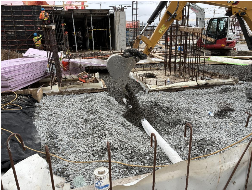
Photo 4: ECD backfilling SSDS piping with previously imported 3/4-inch stone in the western part of the site (facing north)
