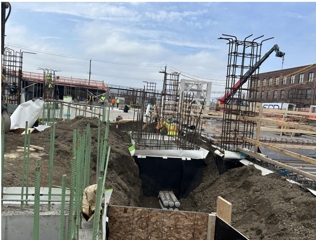
Photo 4: ECD installing utility piping in the central part of the site (facing north)
