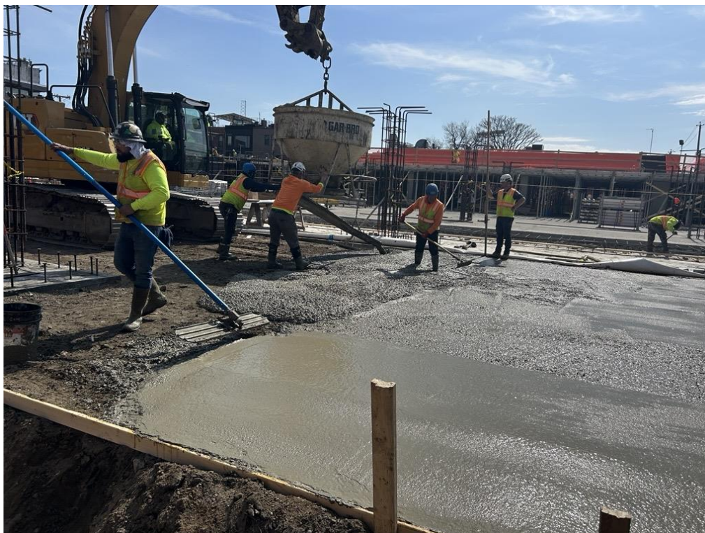
Photo 2: ECD pouring a 3-inch-thick rat slab in the northern part of the site (facing southwest)
