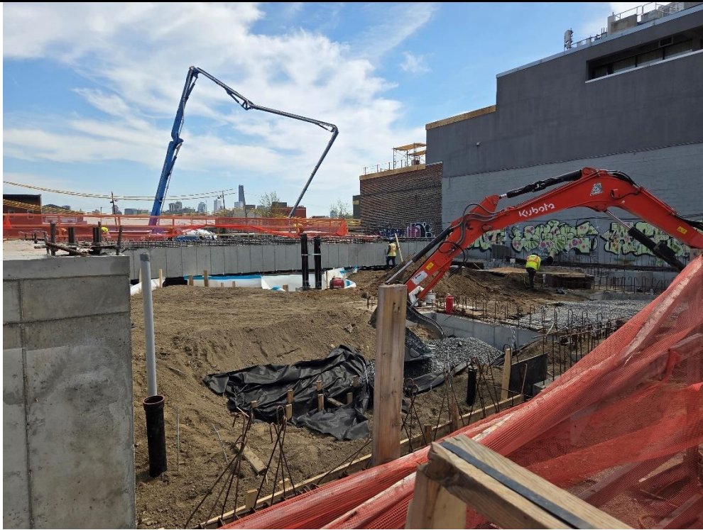
Photo 3: ECD backfilling with imported ¾-inch ASTM No. 5 stone for the SVE system installation in the western part of the site (facing east)
