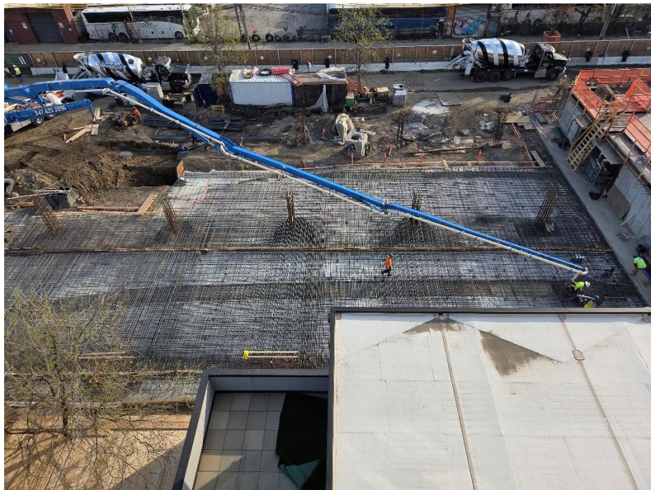
Photo 4: ECD pouring concrete in the central part of the site (facing down)
