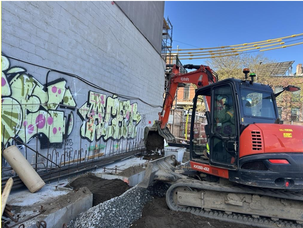
Photo 4: ECD backfilling with previously imported clean fill in the western part of the site (facing west)
