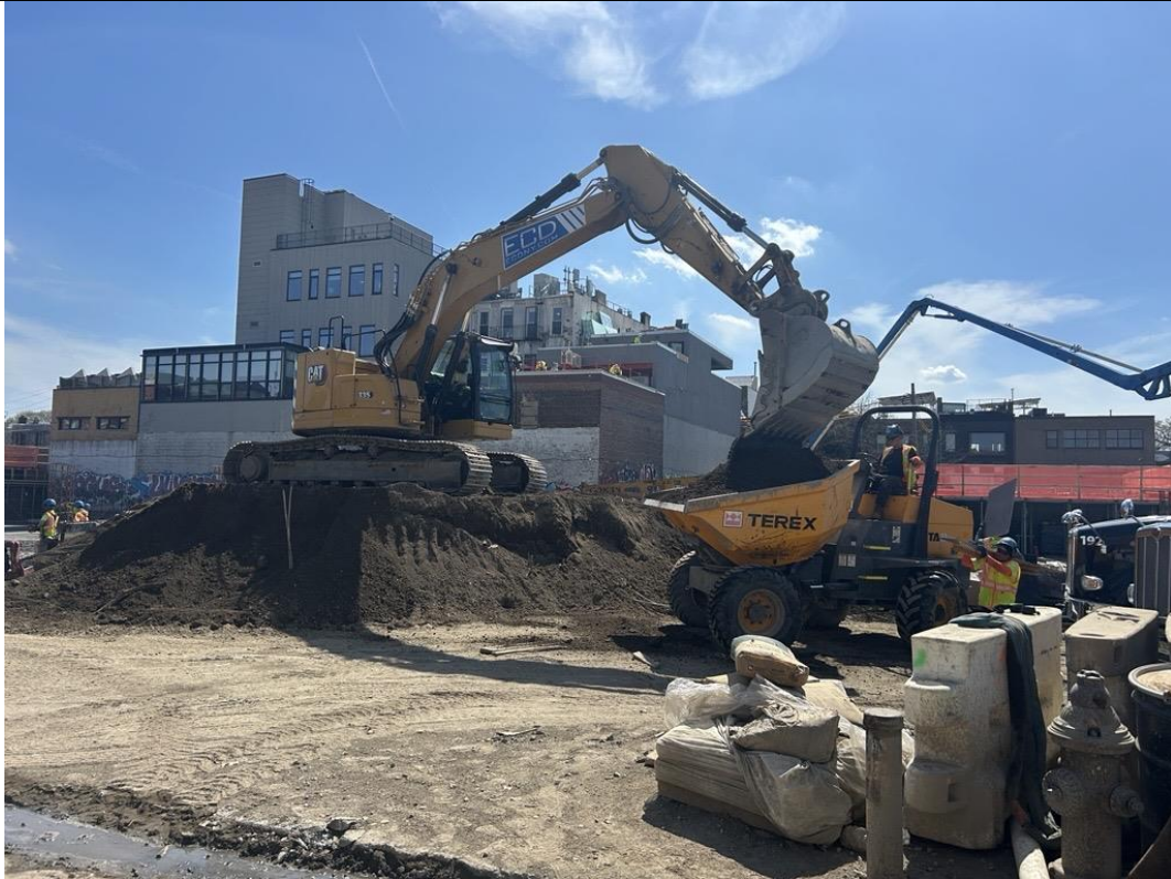
Photo 3: ECD relocating stockpiled imported clean fill from the eastern part of the site to the western part of the site for future backfill (facing south)
