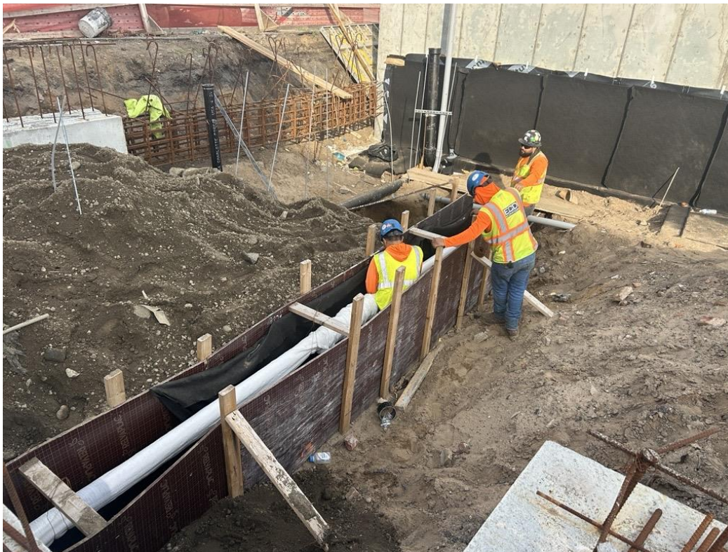
Photo 1: ECD installing SVE piping in the western part of the site (facing west)
