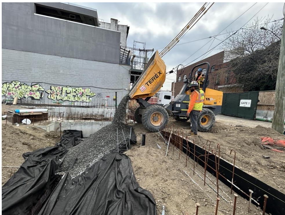
Photo 2: ECD backfilling \frac{3}{4} -inch ASTM No.5 stone atop geotextile fabric in the western part of the site (facing south)
