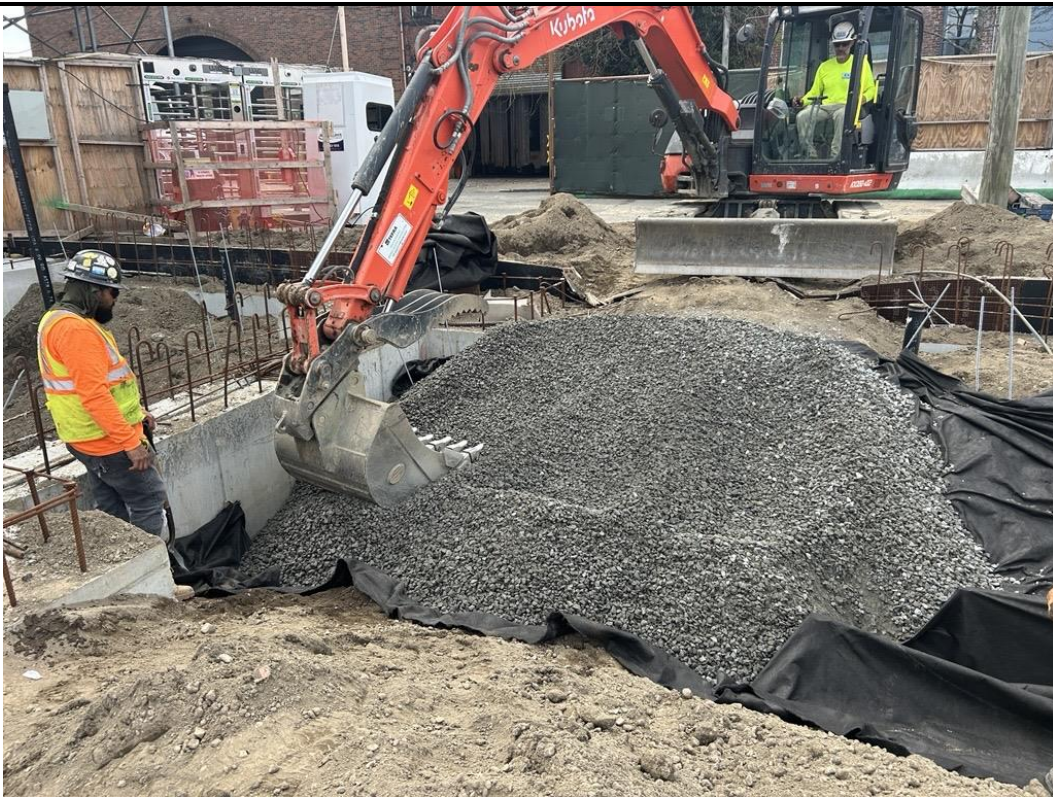
Photo 3: ECD backfilling with imported 3/4-inch ASTM No. 5 stone for the SVE system installation in the western part of the site (facing southwest)
