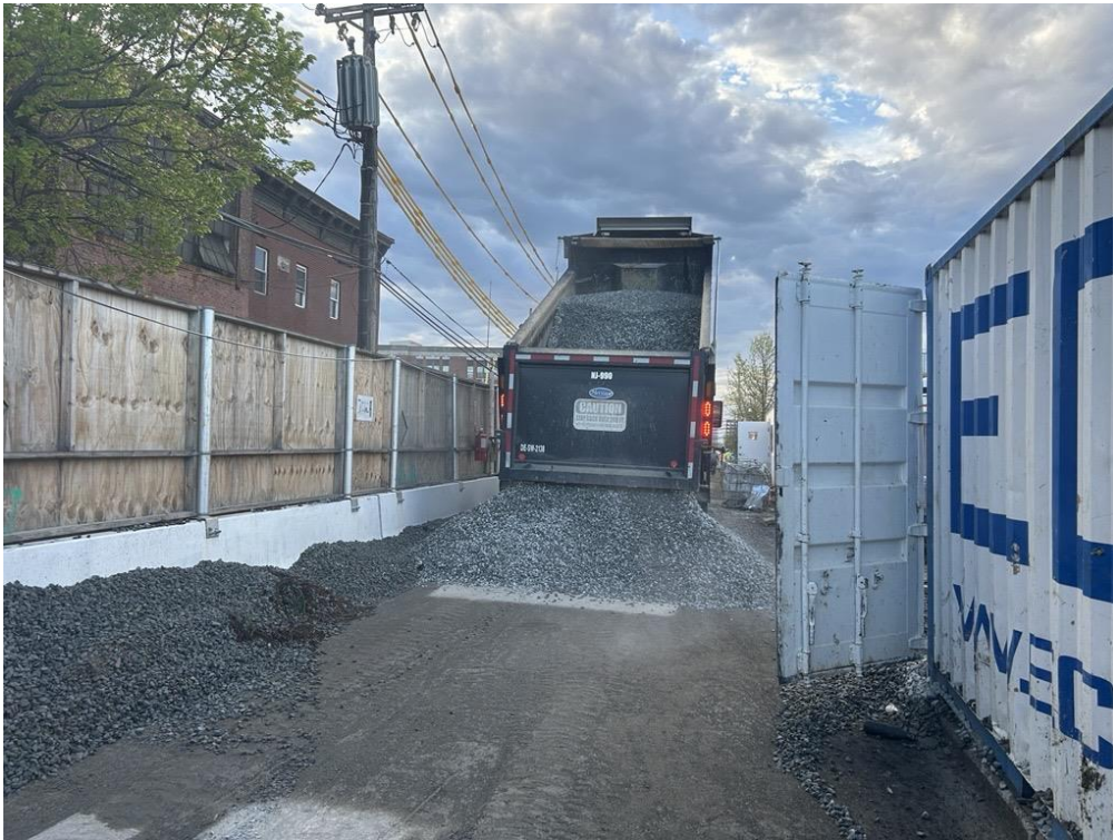
Photo 1: ECD importing approved ¾-inch ASTM No.5 stone in the eastern part of the site (facing southeast)
