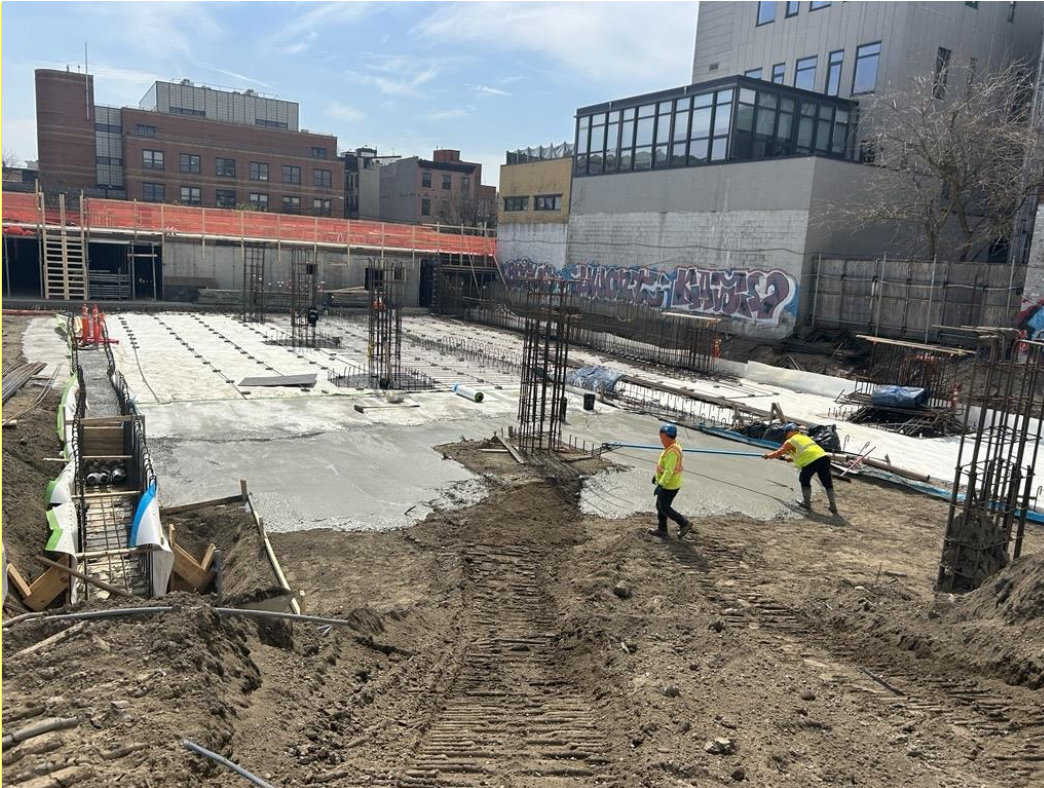
Photo 4: ECD pouring a 3-inch rat slab in the central part of the site (facing south)
