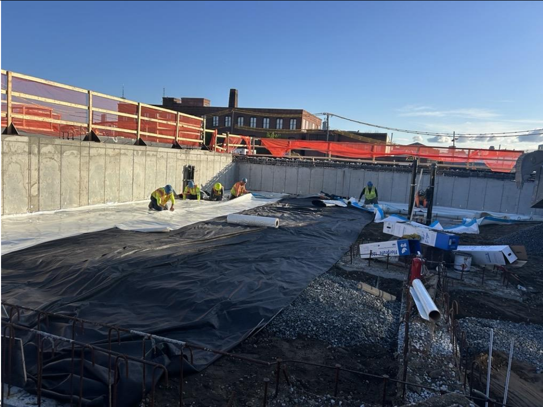
Photo 3: ECD installing Florprufe 120 waterproofing / vapor barrier in the western part of the site (facing north)
