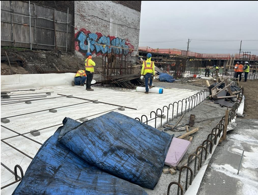
Photo 3: ECD installing Preprufe 300R Plus waterproofing / vapor barrier membrane in the central part of the site (facing northwest)
