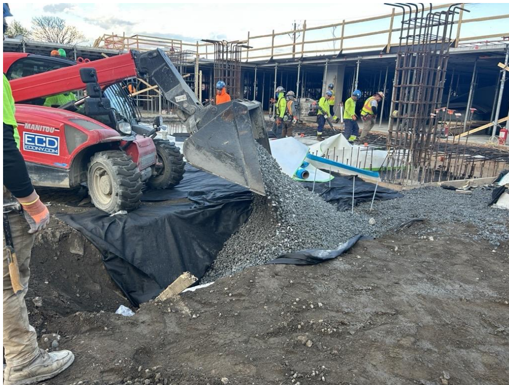
Photo 2: ECD backfilling with ¾-inch virgin stone (gas permeable aggregate) as the SVE system in the northern part of the site (facing west)
