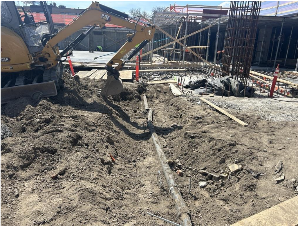
Photo 1: ECD excavating non-native fill for utility pipe installation in the northern part of the site (facing southwest)
