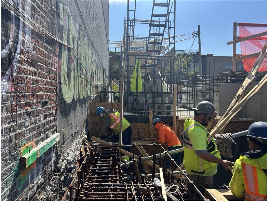
Photo 3: ECD installing scaffolding in the western side of the site (facing west)
