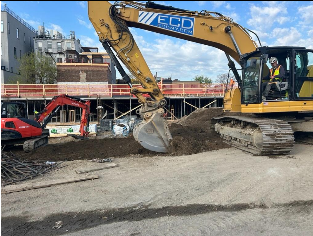
Photo 3: ECD excavating for future soil vapor extraction system installation in the eastern part of the site (facing west)
