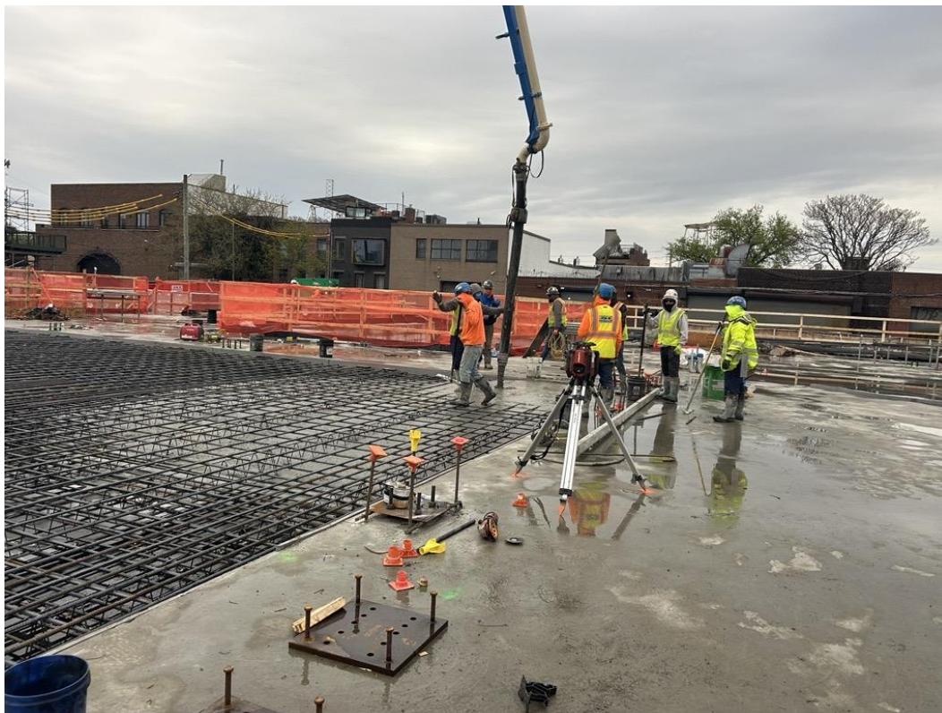
Photo 4: ECD pouring concrete on the second floor of the building (facing south)
