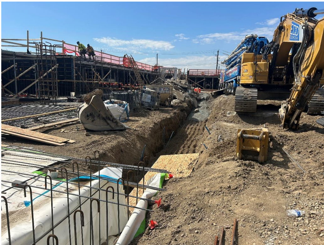
Photo 2: ECD excavating for utility piping installation in the central part of the site (facing north)
