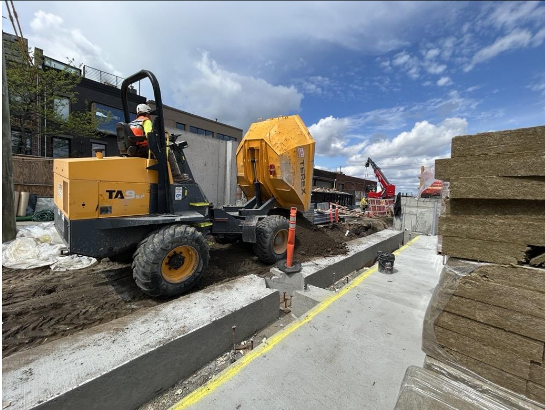
Photo 3: ECD backfilling with previously imported clean fill in the western part of the site (facing west)
