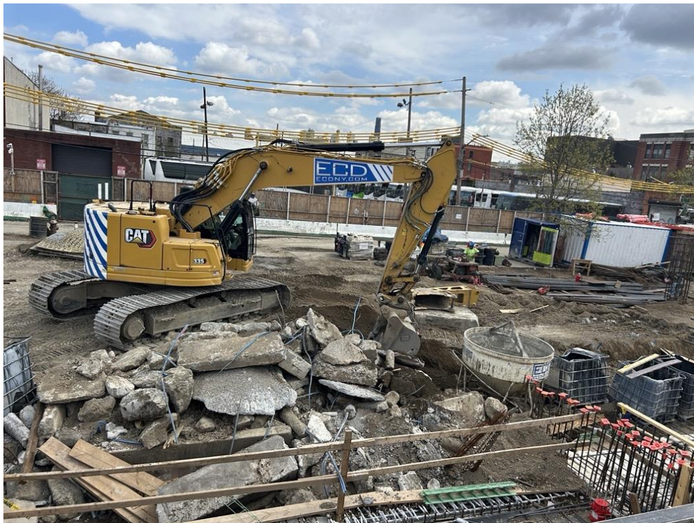
Photo 2: ECD excavating for utility piping in the central part of the site (facing east)
