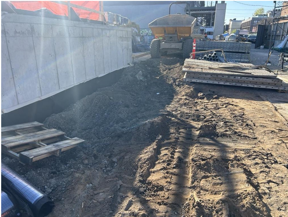
Photo 1: ECD backfilling with clean imported fill in the western part of the site (facing southeast)
