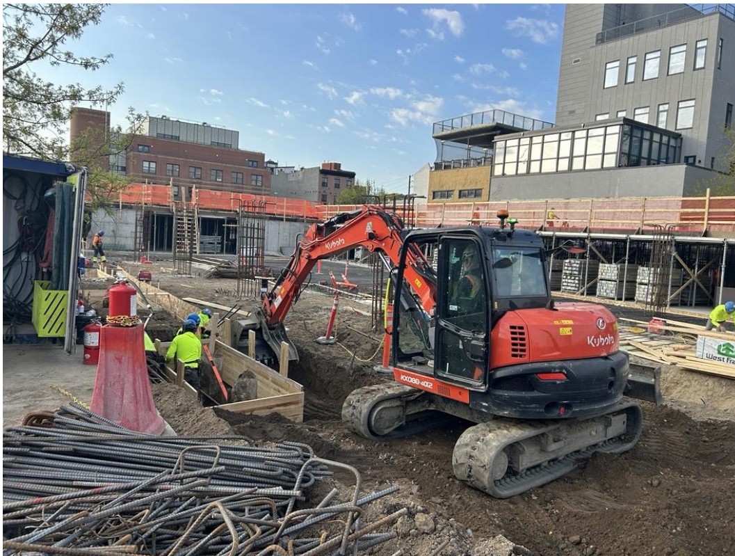
Photo 1: ECD backfilling a utility trench with previously imported clean fill in the eastern part of the site (facing south)
