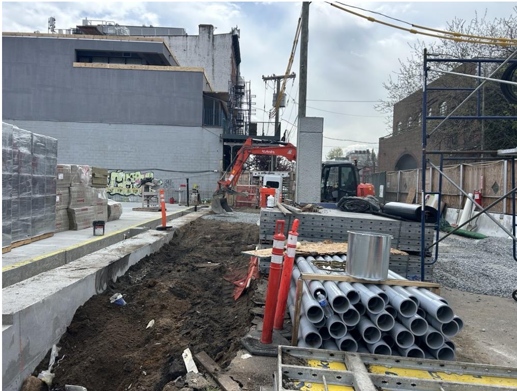
Photo 1: ECD backfilling with imported ¾-inch ASTM No.5 stone in the western part of the site (facing southeast)
