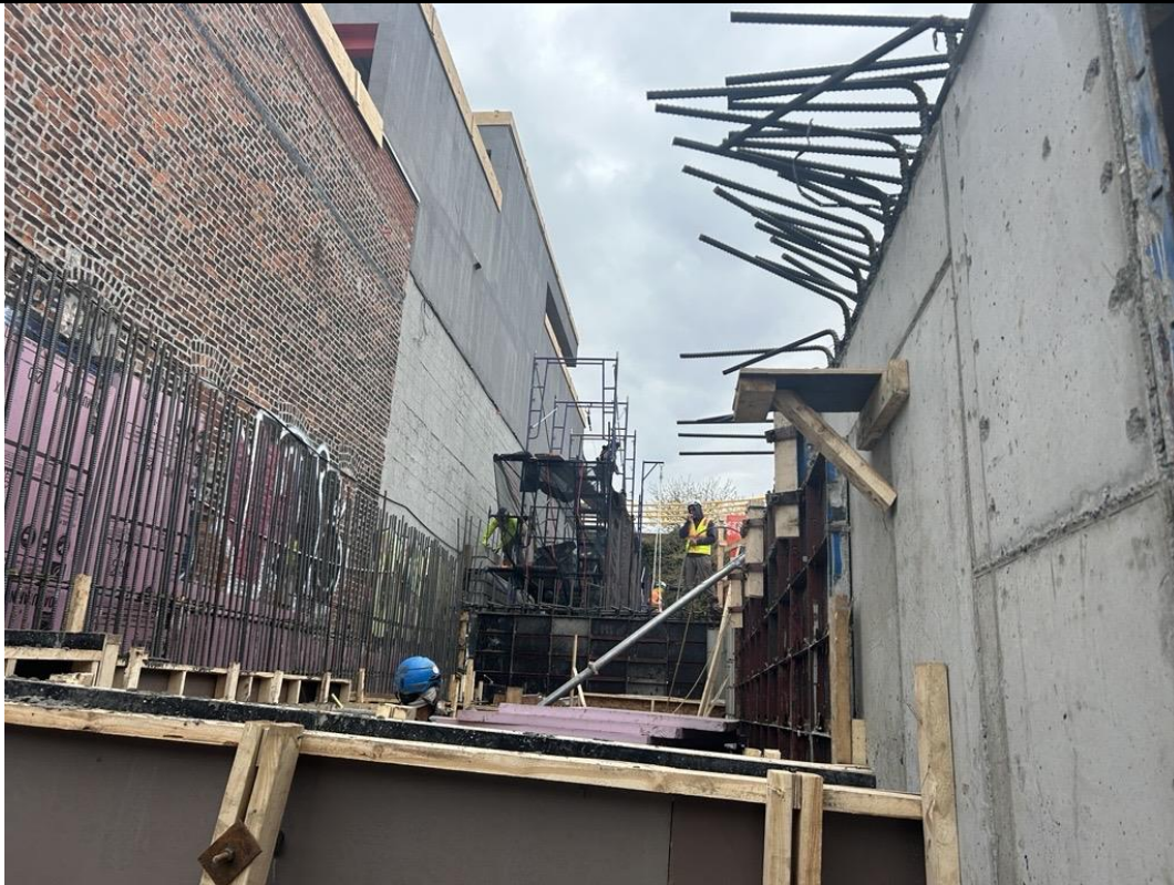
Photo 3: ECD installing scaffolding in the western part of the site (facing southwest)
