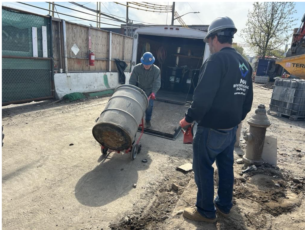
Photo 4: M&W Environmental Solutions collecting one 55-gallon drum for offsite disposal in the eastern part of the site (facing east)
