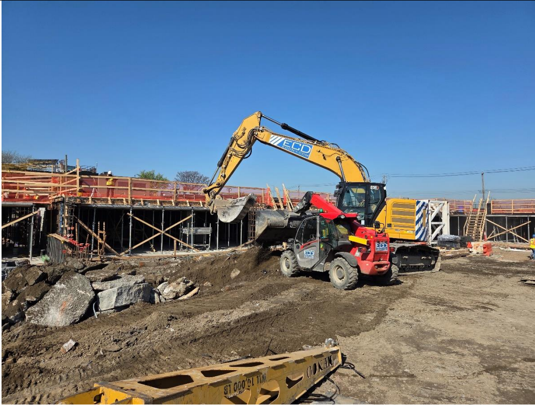
Photo 3: ECD stockpiling excavated non-native fill in the central part of the site (facing west)
