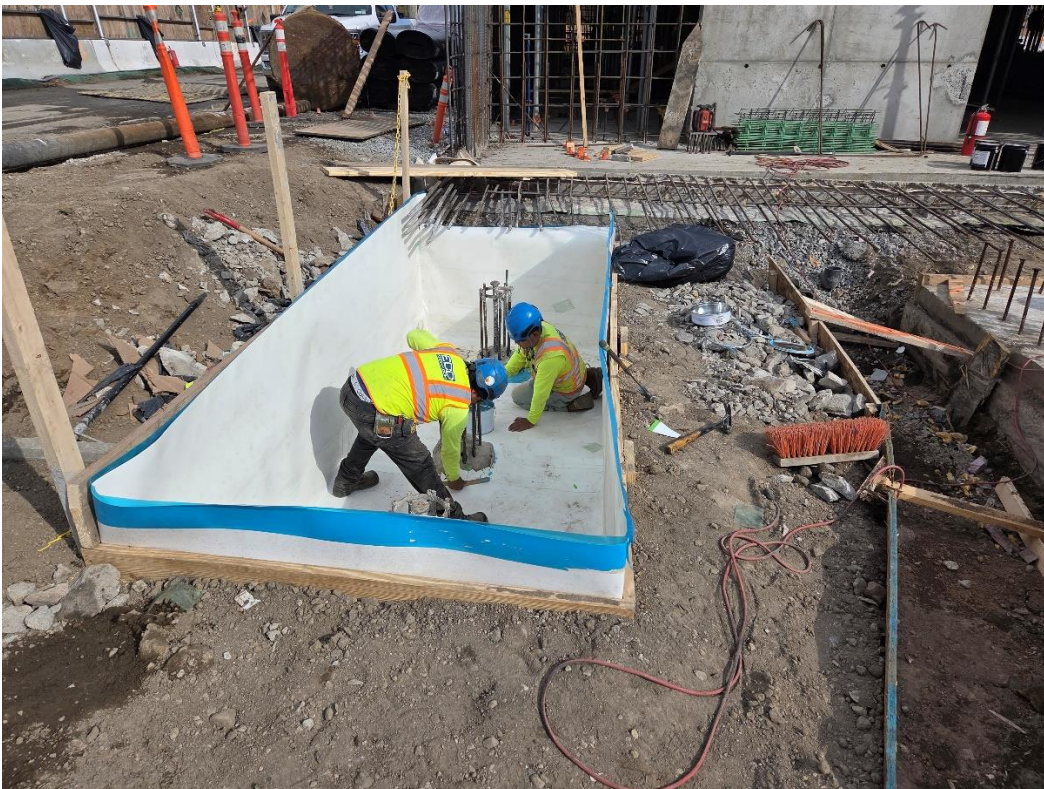
Photo 4: ECD installing Preprufe 300R Plus waterproofing/vapor barrier membrane in the eastern part of the site (facing southeast)
