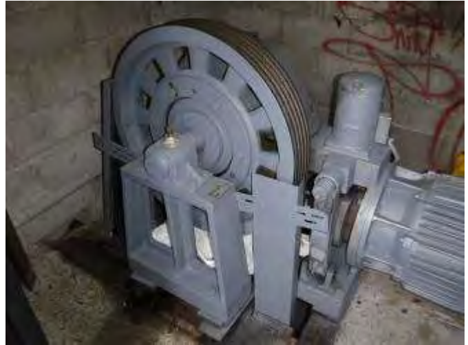
20. 100 South 4 th elevator motor
