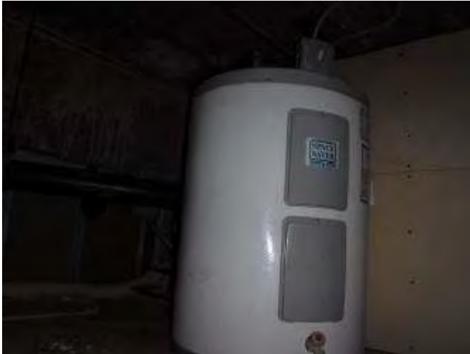
25. 100 South 4 th individual apartment hot water heater
