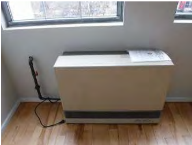
23. 100 South 4 th apartment PTAC unit
