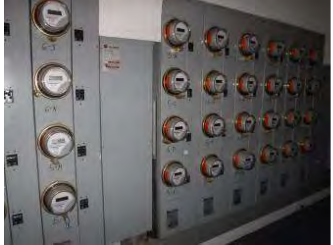
14. 100 South 4 th electric meters
