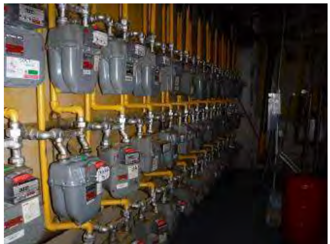
12. 100 South 4 th gas meters
