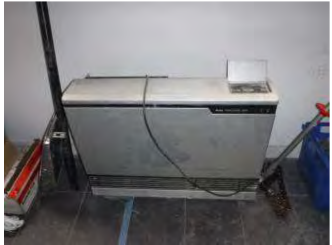
16. 100 South 4 th PTAC unit
