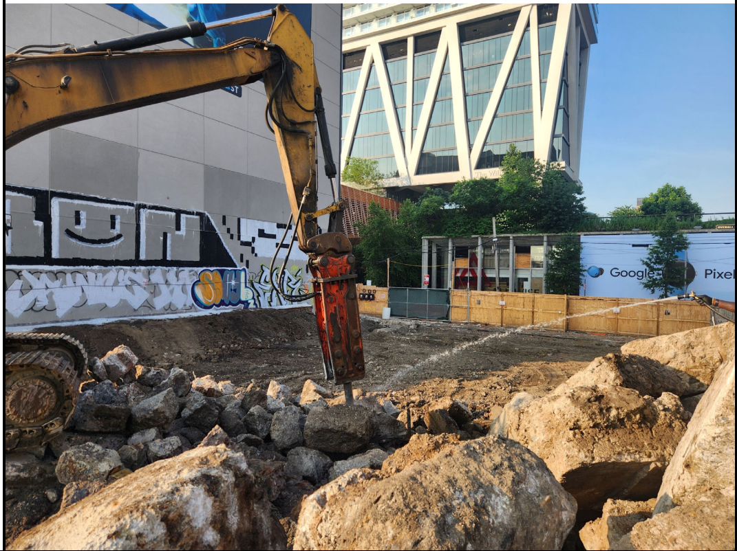
Photo 2: View of concrete demolition. Water is being utilized to minimize dust generation.
