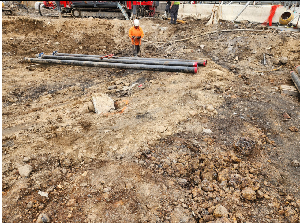
Photo 2: View of the top of the discovered UST.
