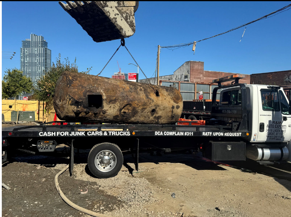
Photo 2: View of the cleaned tank being placed on a truck for offsite disposal.
