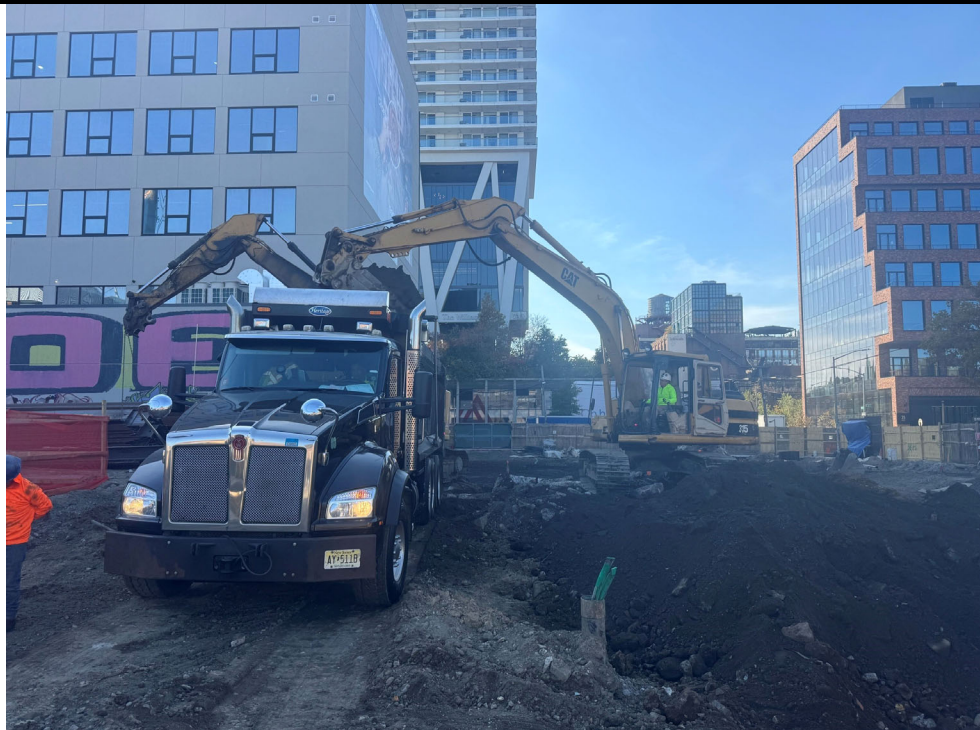
Photo 2: View of non-hazardous soil being loaded into a truck for disposal offsite.
