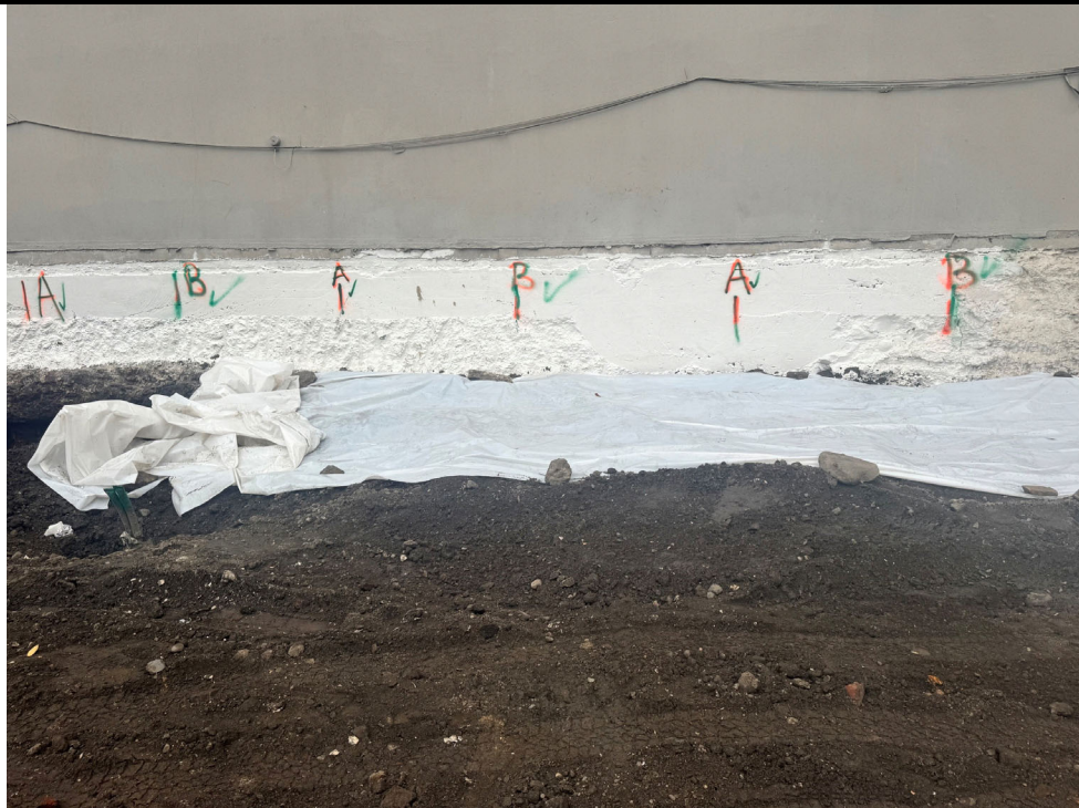
Photo 2: View of odorous soil covered with plastic sheeting.
