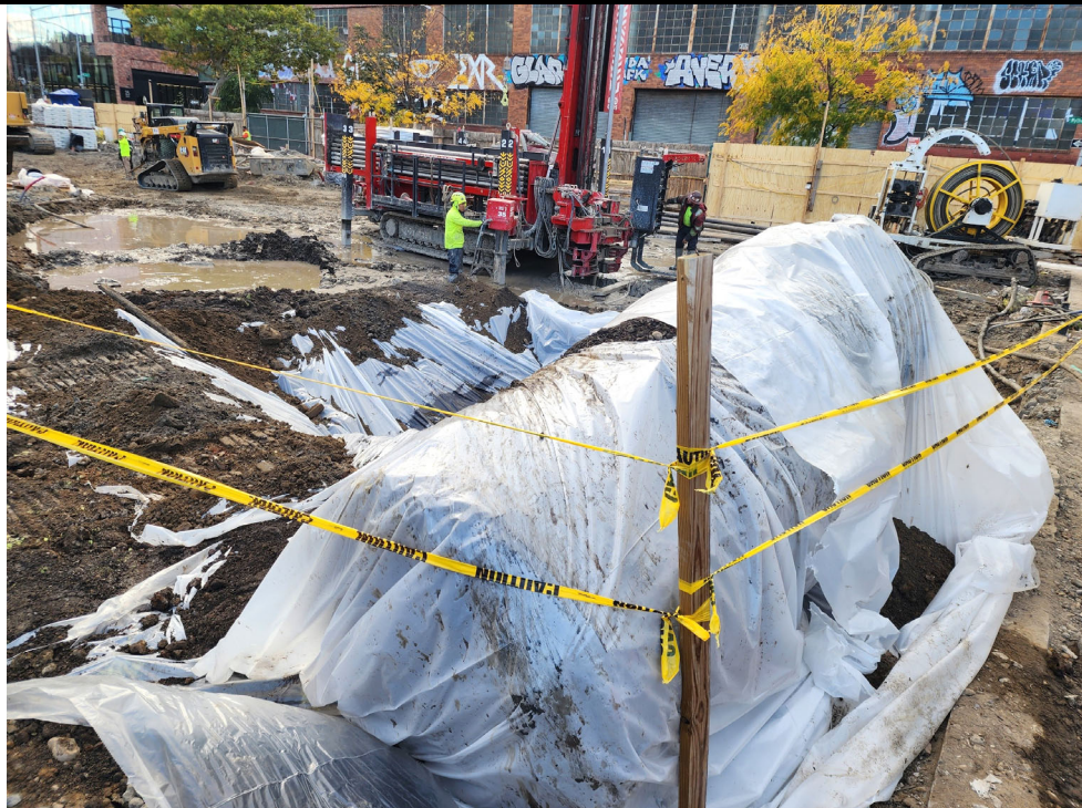
Photo 2: View of the 3,000-gallon UST placed on and under poly sheeting to await offsite disposal.
