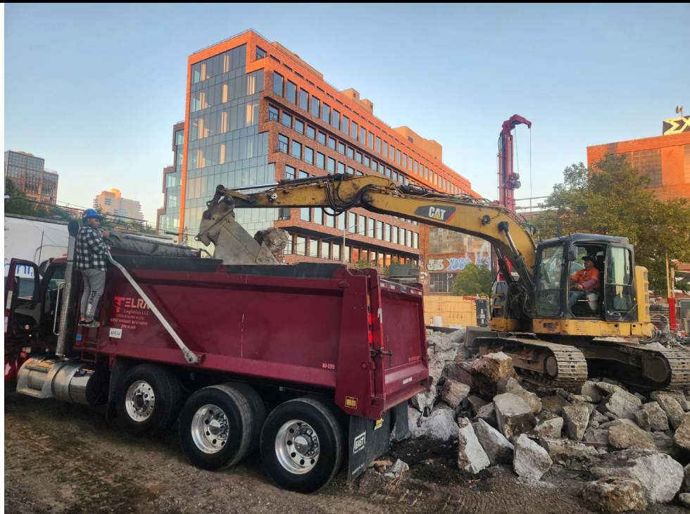
Photo 2: View of concrete debris being loaded into a truck for disposal offsite.
