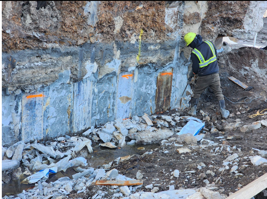
Photo 1: View of concrete chipping along adjacent building.
