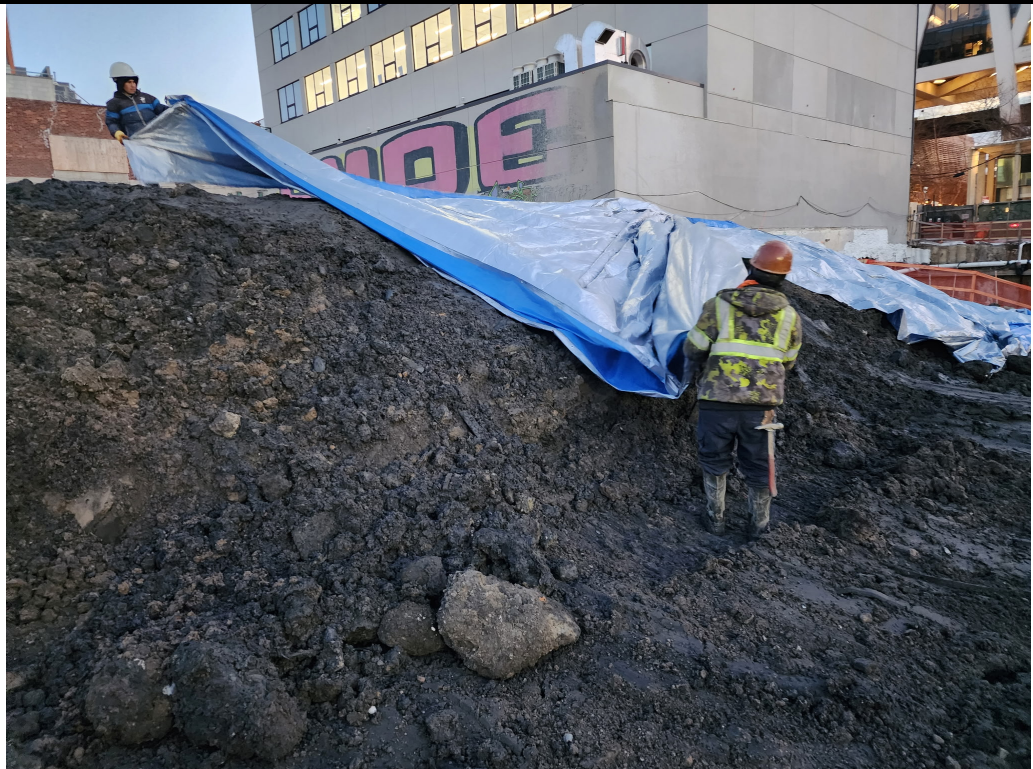
Photo 2: View of covering soil stockpiled for offsite disposal.
